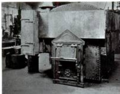
One of four Haden warm air stoves in St Pauls Cathedral, London, 1912
