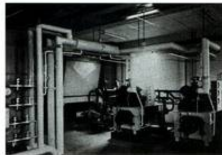
Air conditioning plant room for H.M. Customs Laboratory in Adelaide
