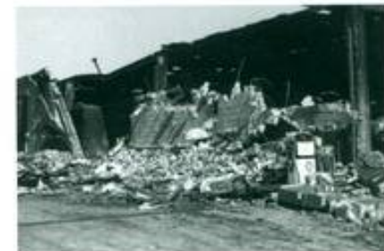
Fire damage at Haden's Rosebery office, Sydney, 1981
