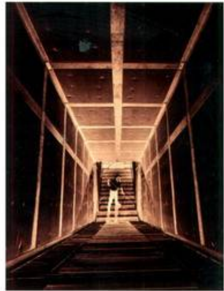
The large relief duct above the concert hall at Sydney Opera House
