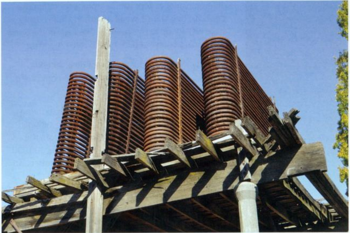
Rusty roof coils remain intact
