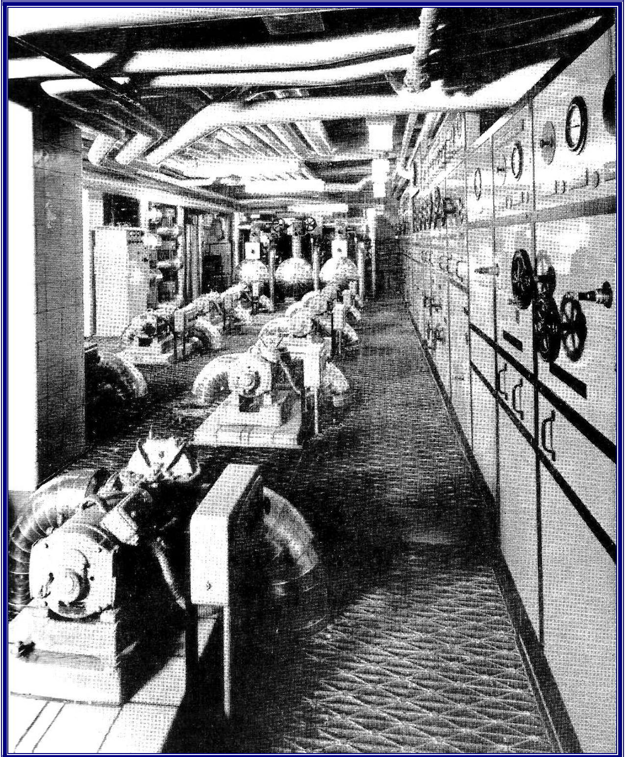
Pump Room at the new House of Commons (installed by Benham & Sons Ltd)
