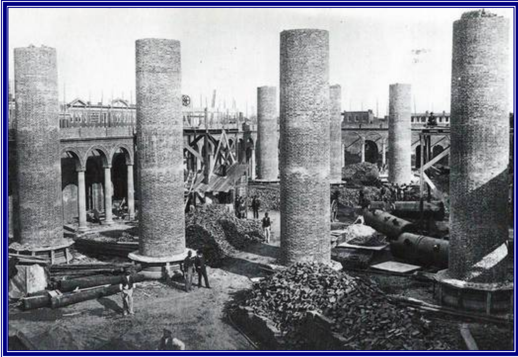
The giant columns, which are 75 feet high and 8 feet diameter, under construction.
