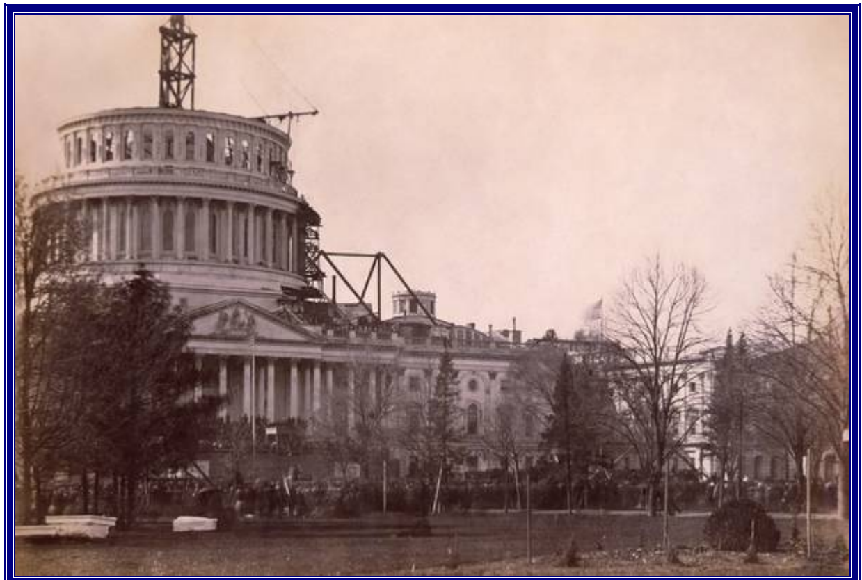
Building the Capitol's new dome at the time of President Abraham's inauguration in 1861
