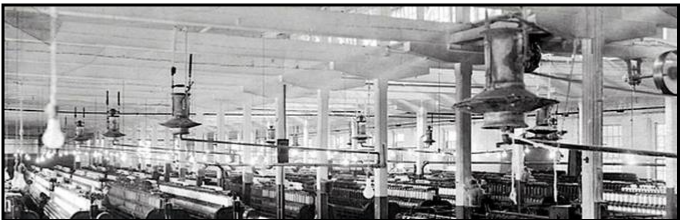
Ceiling-hung humidifiers in a textile mill
