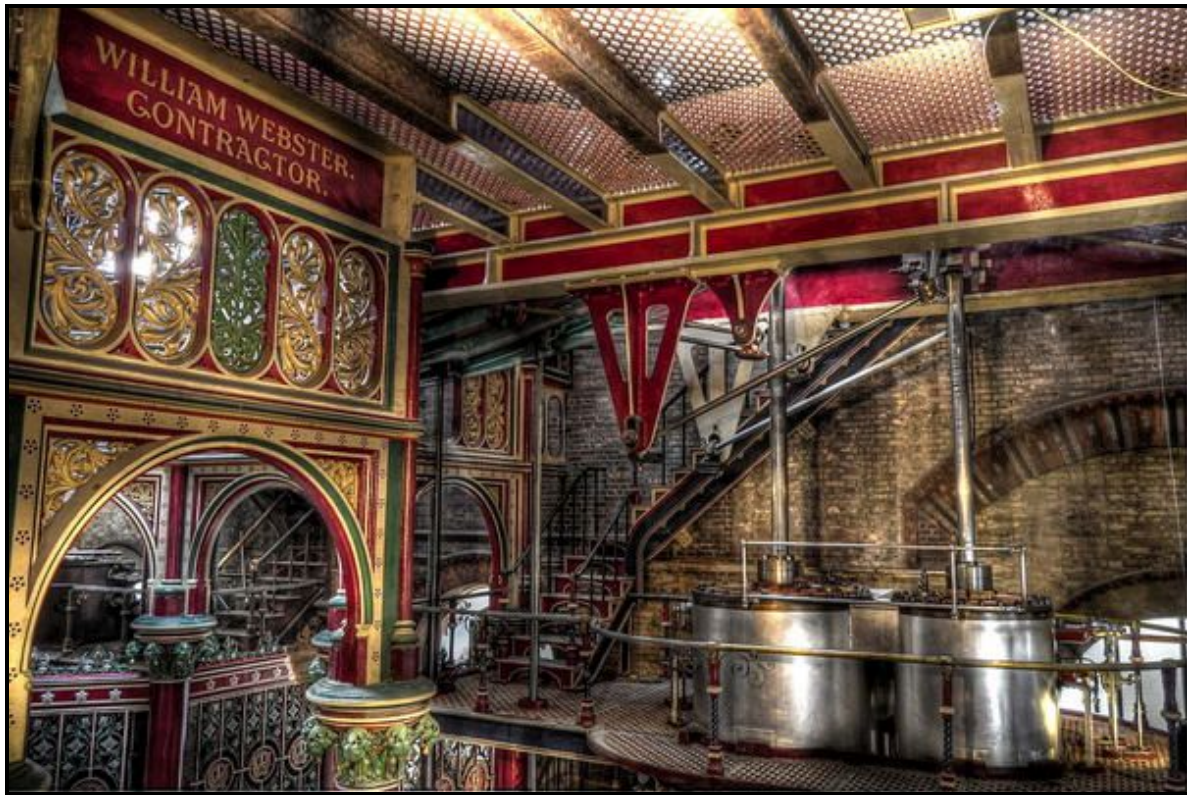
The sewage was pumped by four steam-driven rotative beam engines: Prince Consort, Victoria, Albert Edward & Alexandra
