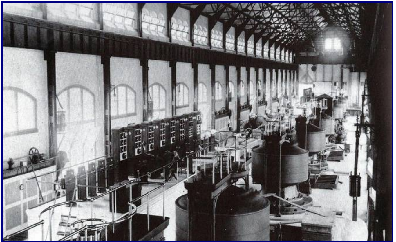
The success of AC was assured when in 1896 the Niagara Falls hydroelectric power station went on-line with the first four of ten Tesla-Westinghouse 5000 horsepower generators providing 3-phase distribution lines to Buffalo, some 22 miles away
