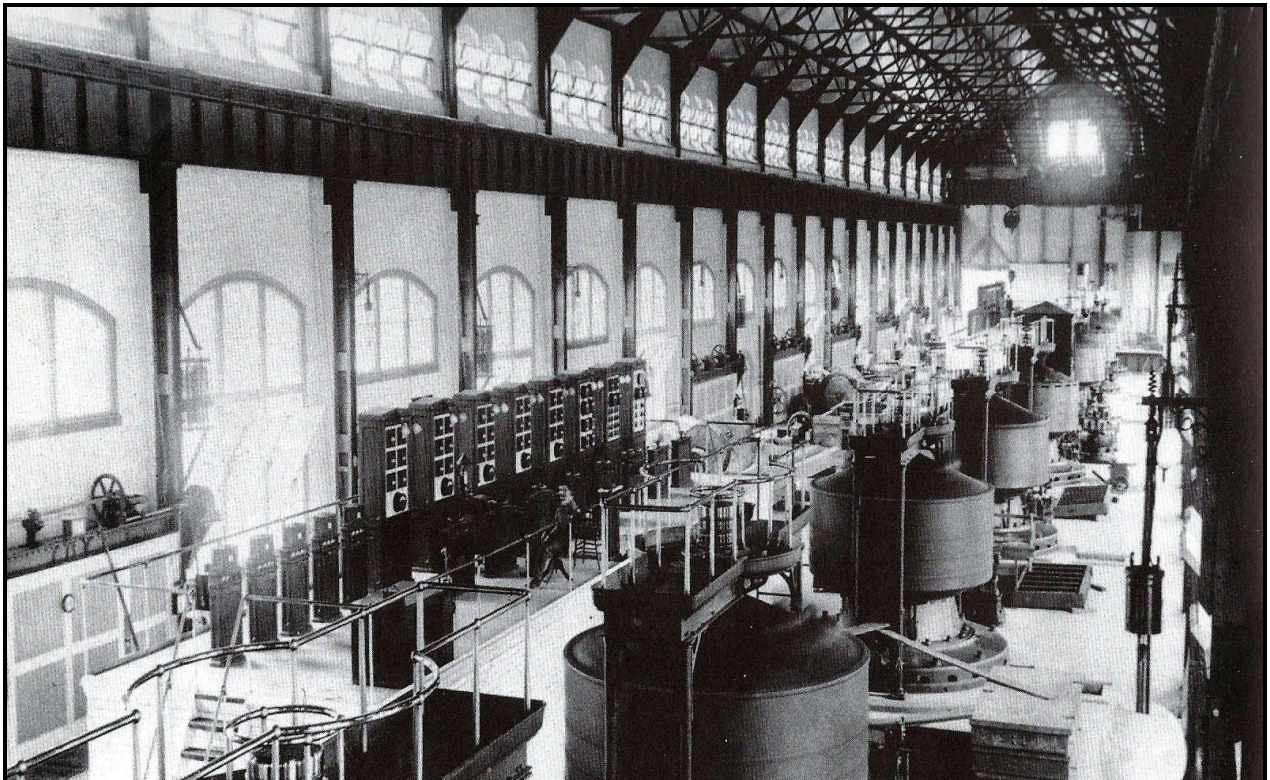
The Edward Dean Adams Power Station at Niagara Falls with ten 5000 horsepower Tesla-Westinghouse AC generators
