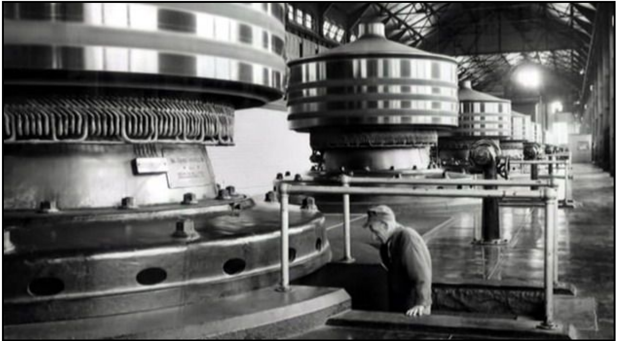
Niagara Falls Power Station which transmitted AC at 22 kV to Buffalo some 22 miles away and later to New York a distance of over 300 miles
