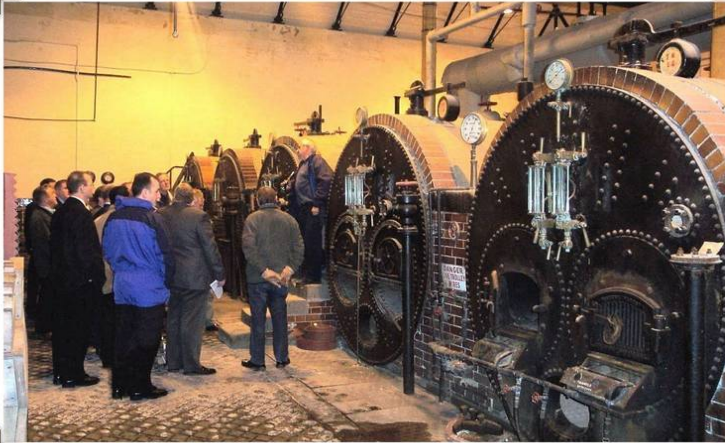
Steam boilers, Papplewick pumping station, Nottinghamshire CIBSE visit, 2007
