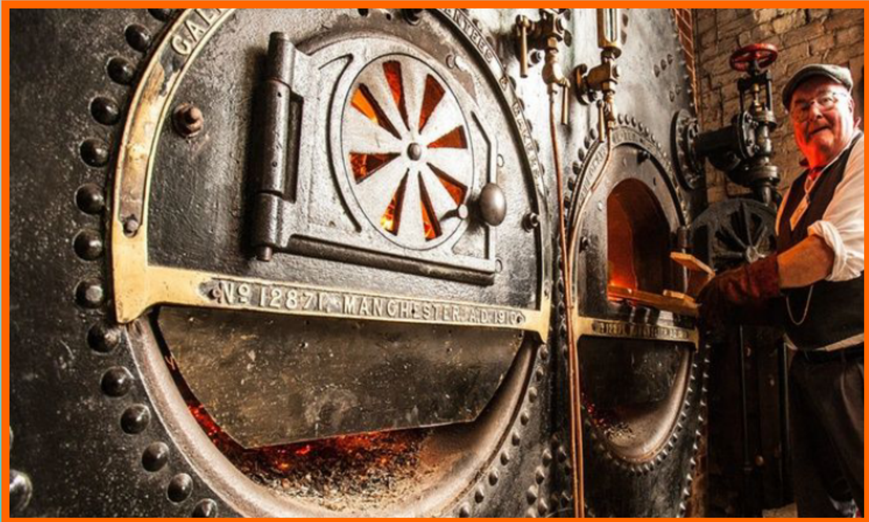
Galloway steam boiler "No.12871 Manchester AD 1910," Coldharbour Mill, Devon
