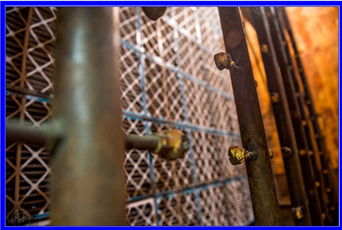
Two bank spray air washer and spray nozzle close-up
