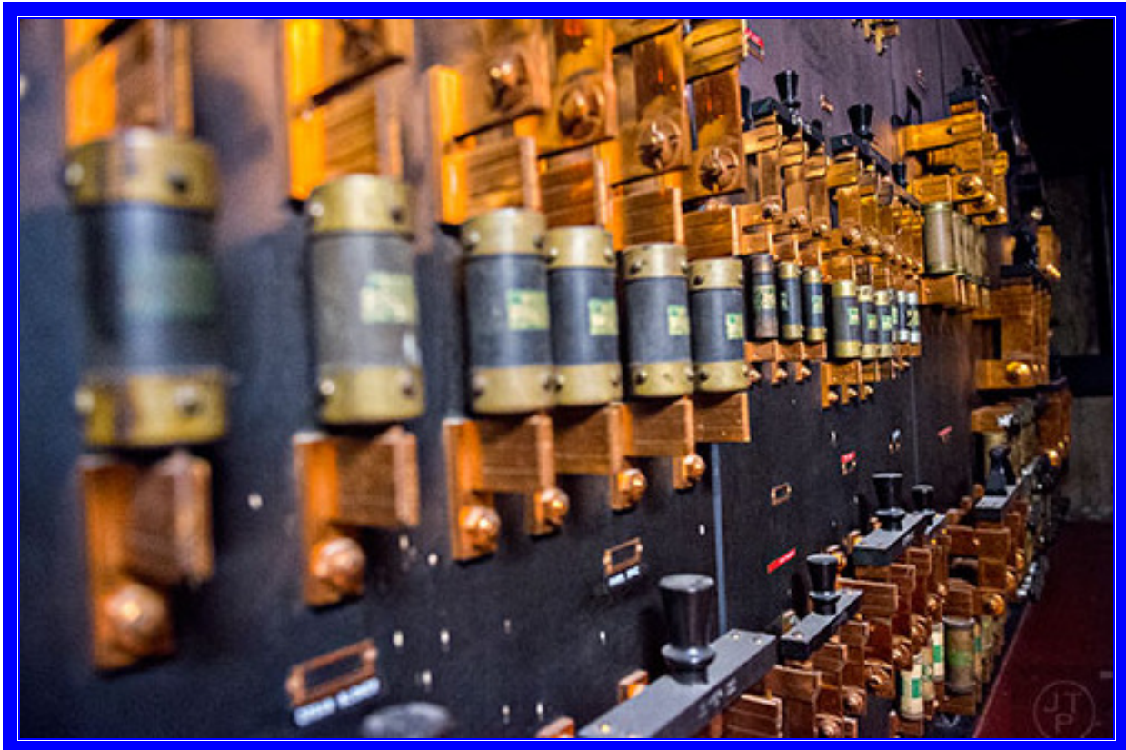
The now unused electrical switchboards
