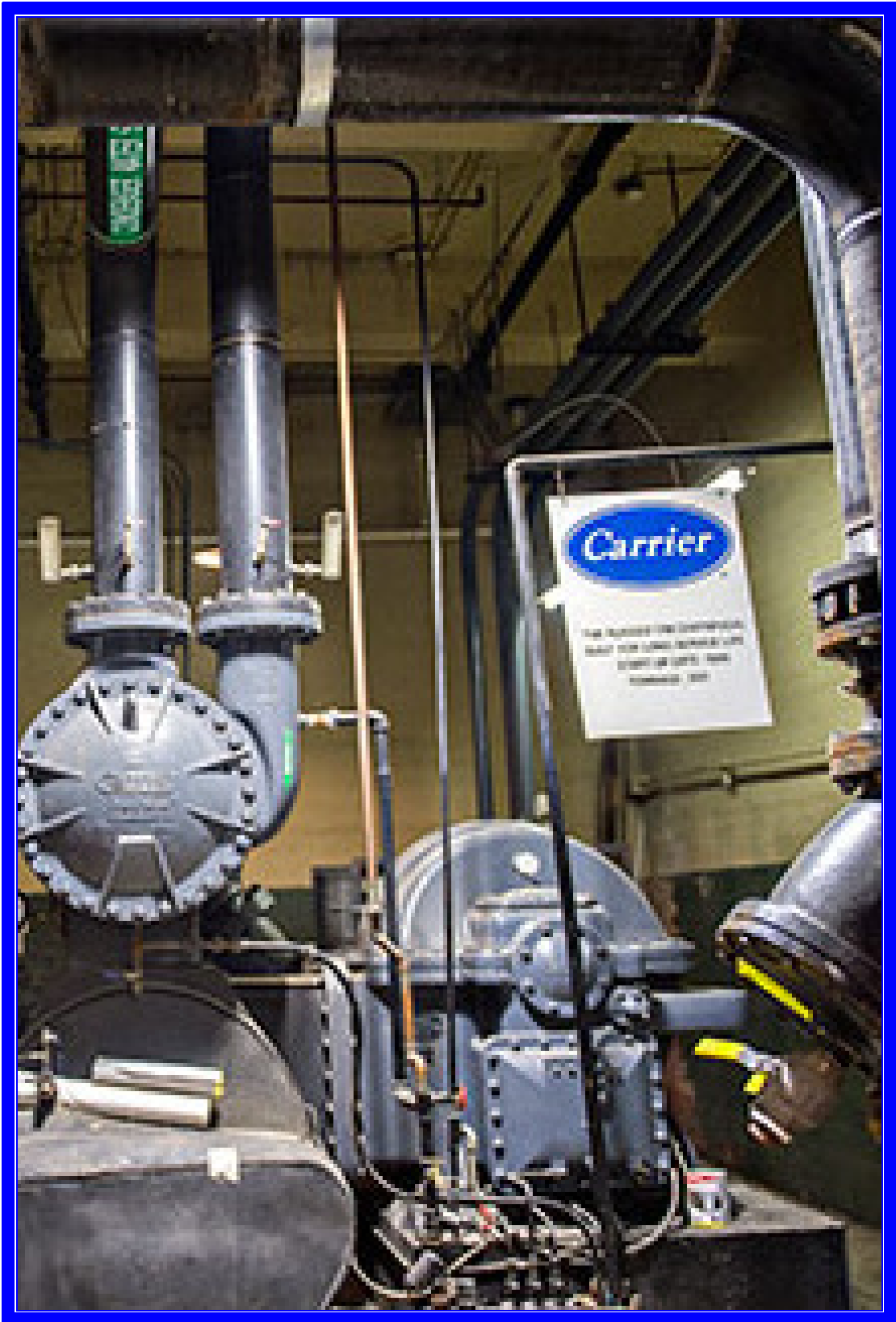
The 1946 Carrier centrifugal chiller
