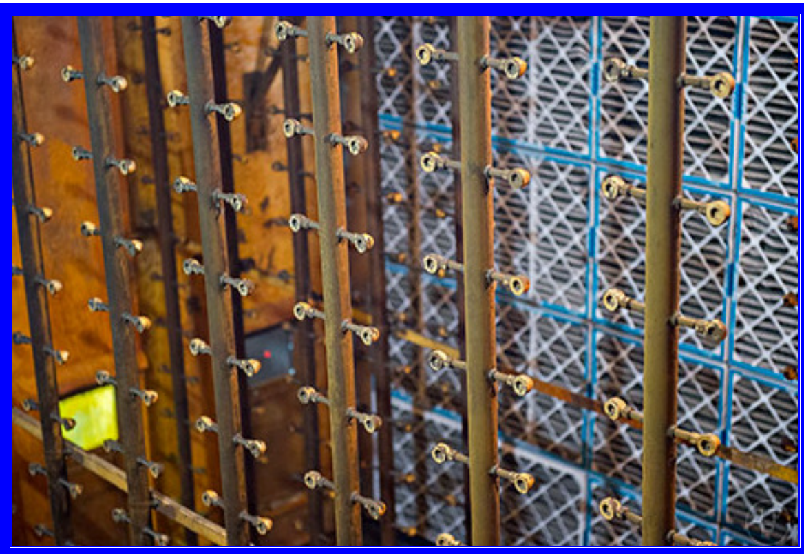
Spray air washer and filter bank
