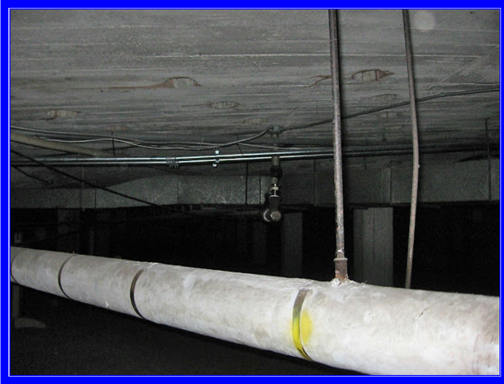
Basement supply air plenum chamber with the ceiling having multiple circular holes connecting to auditorium "mushroom" supply air outlets on the auditorium floor
