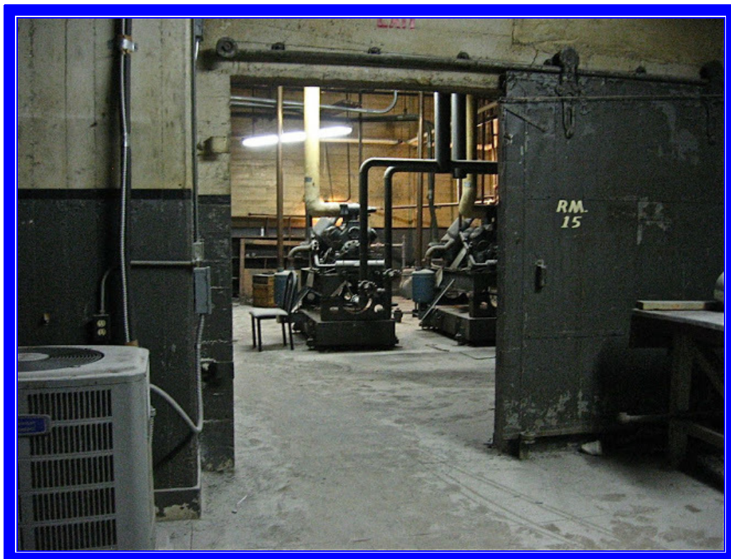
Refrigeration plant room with two ammonia machines ALL ENGINEERING SERVICES PHOTOGRAPHS FROM losangelestheatres.blogspot.com
