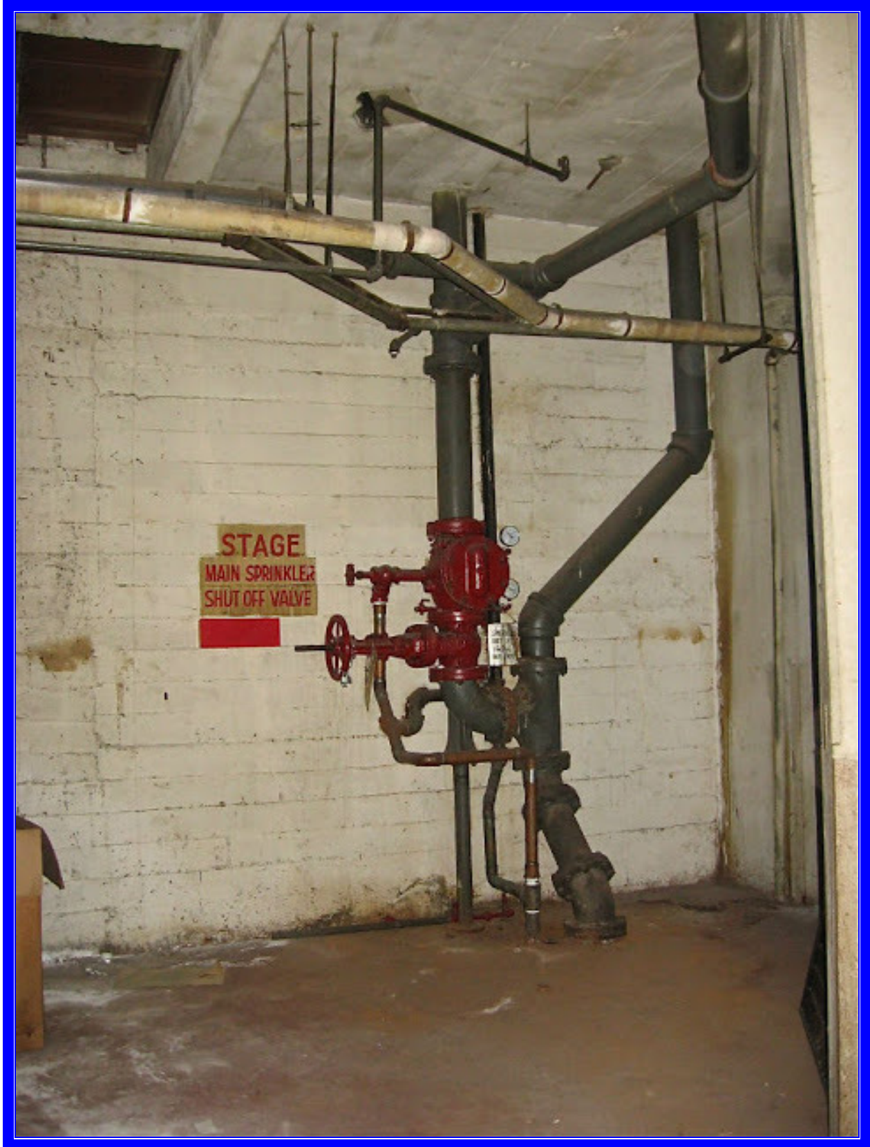
Stage sprinkler piping
