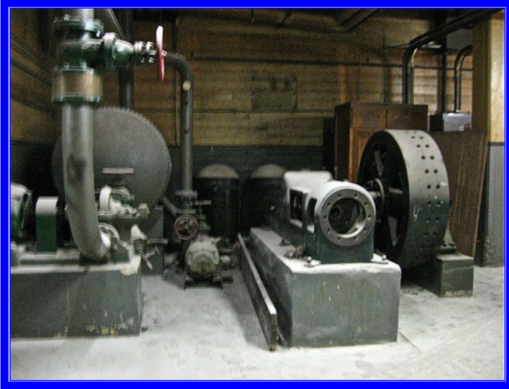
Remains of ammonia refrigerating compressor
