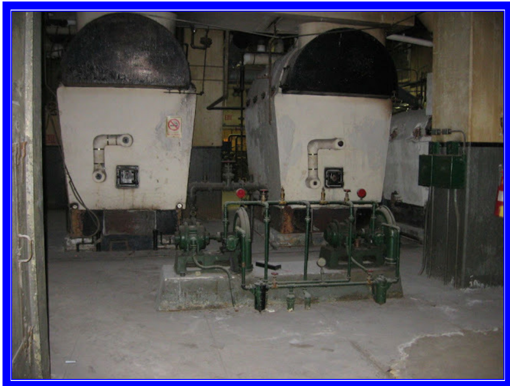
The boiler plant
