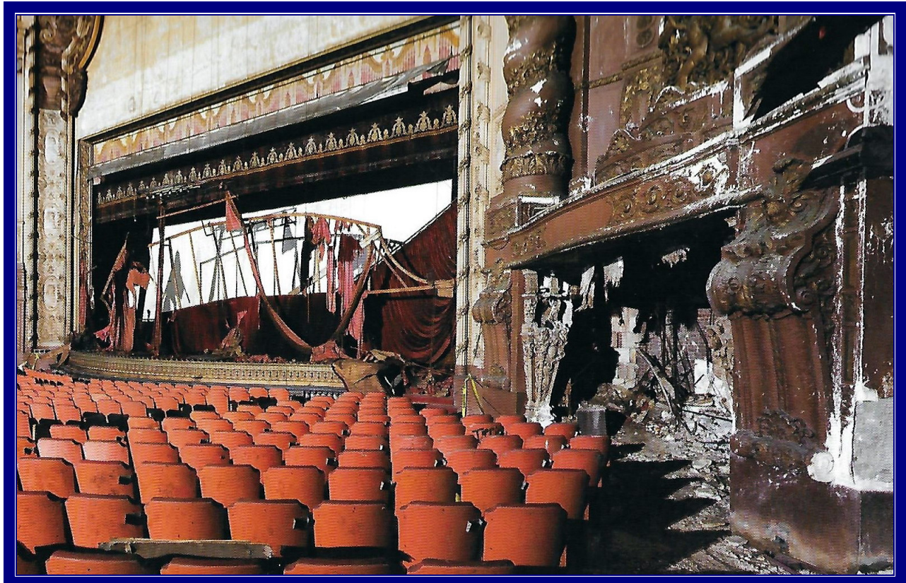
The auditorium damage before restoration (KTML)
