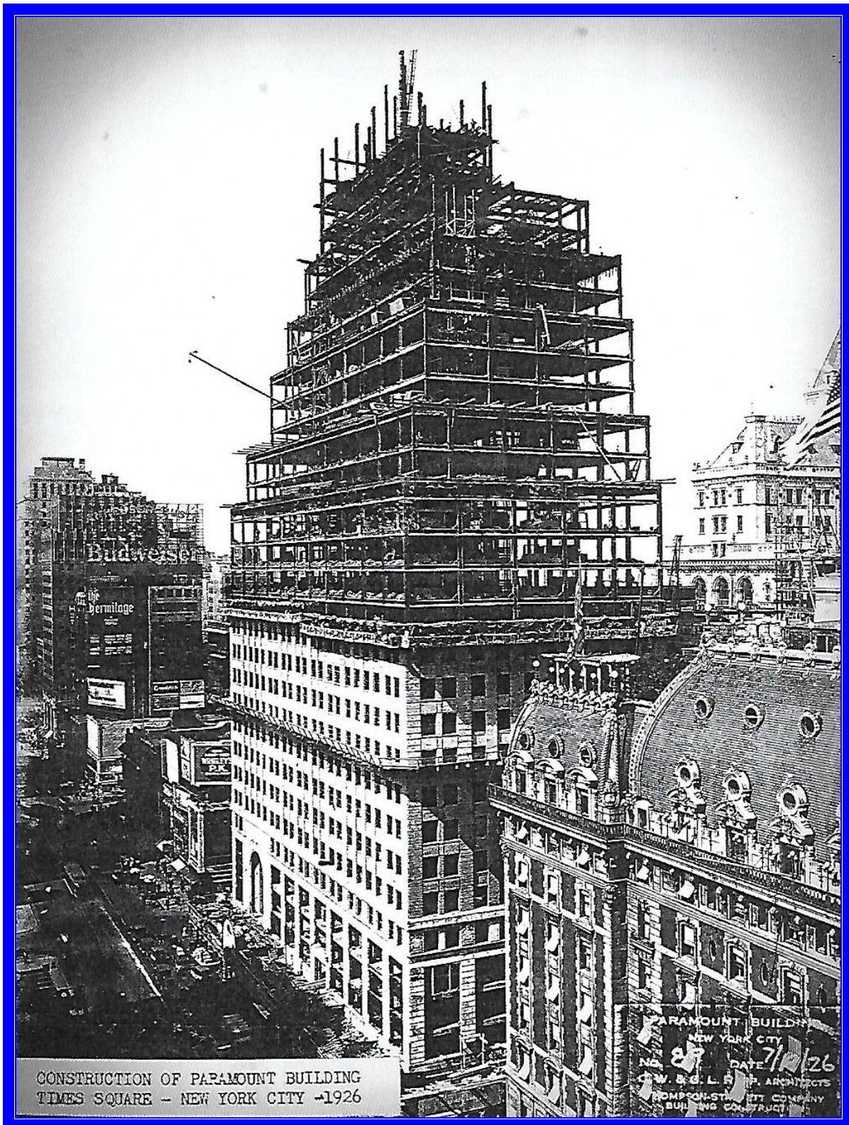
Construction to the designs of Rapp & Rapp underway on the Paramount Building & Theatre, Times Square, New York 1926
