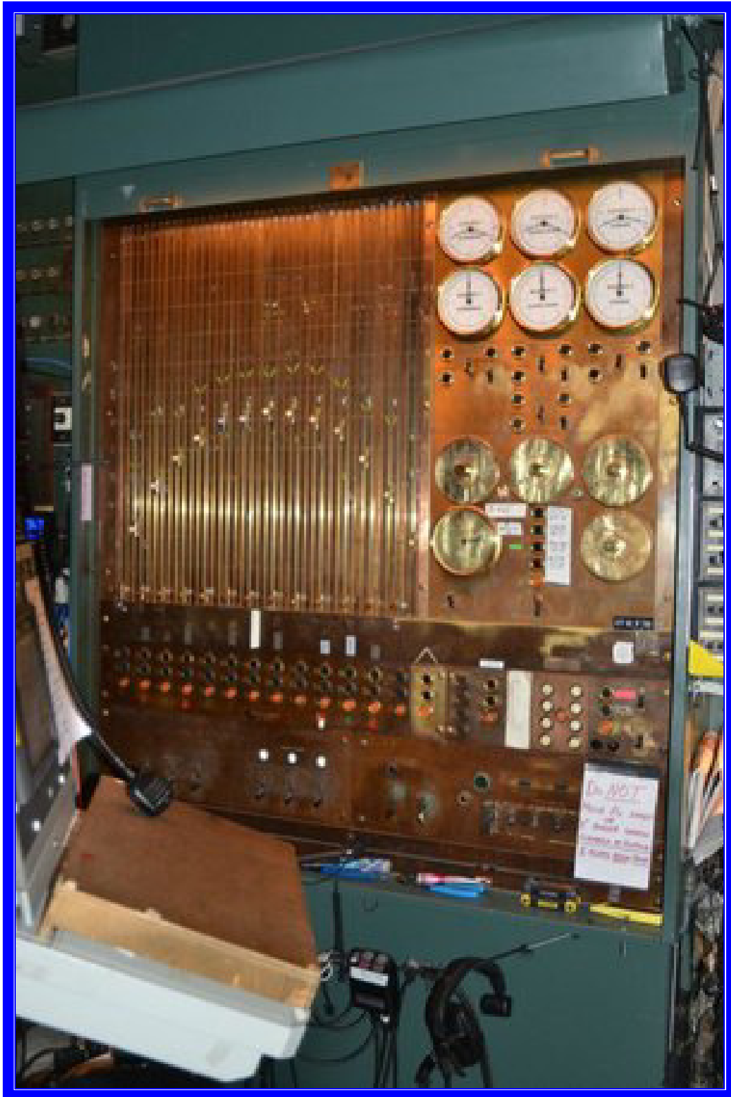
Original control panel for stage curtains
