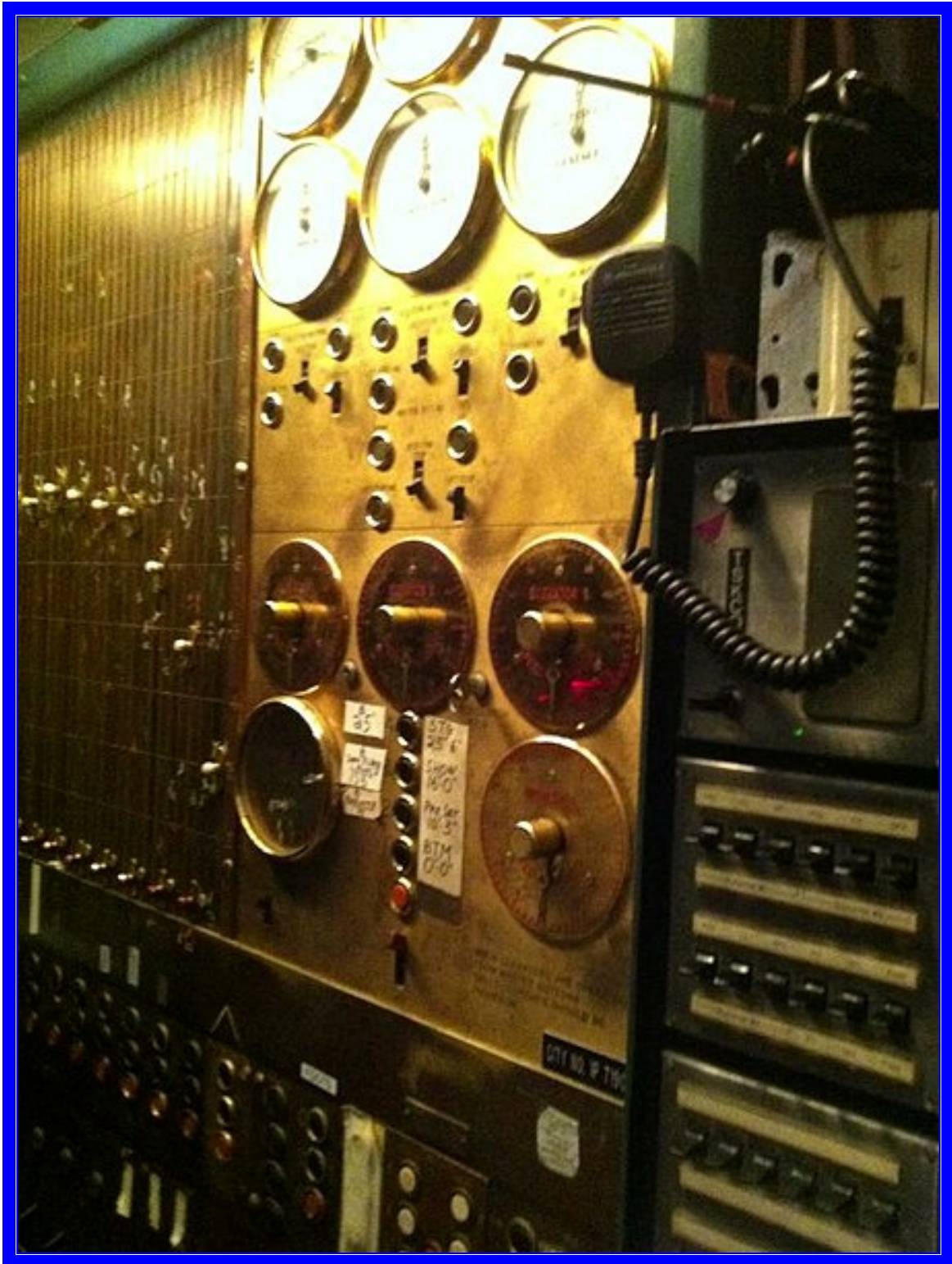
The original stage elevators control board
