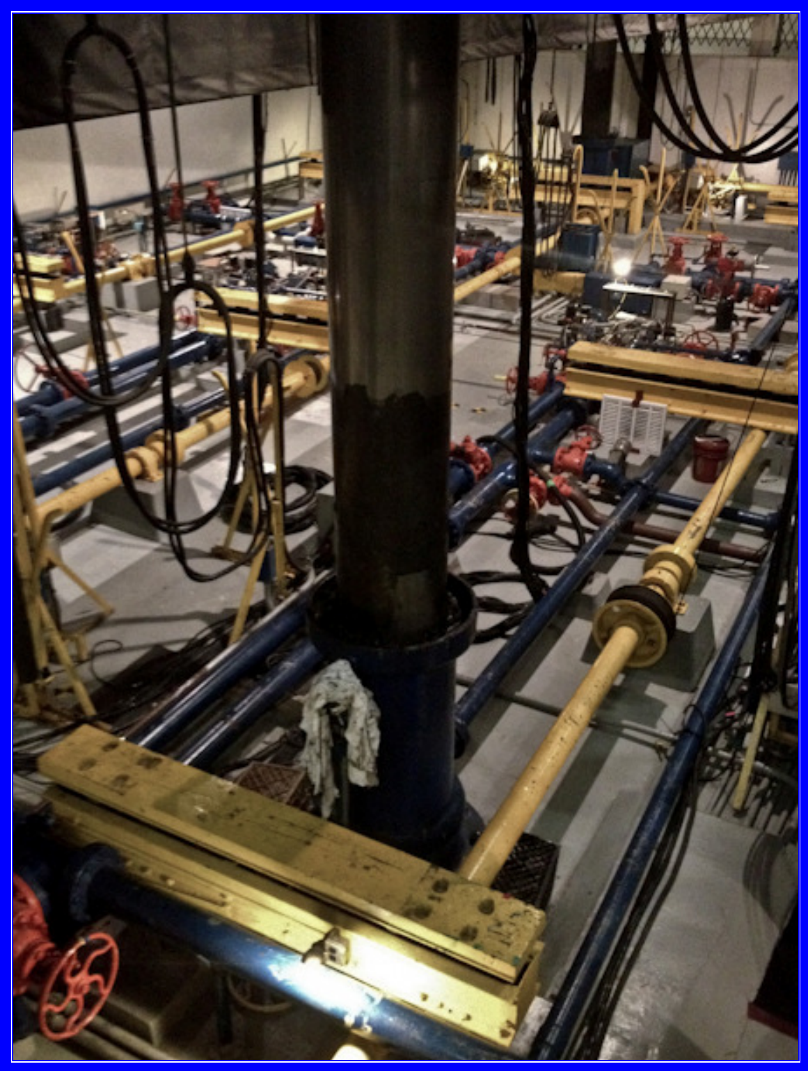
One of the stage elevator giant hydraulic pistons
