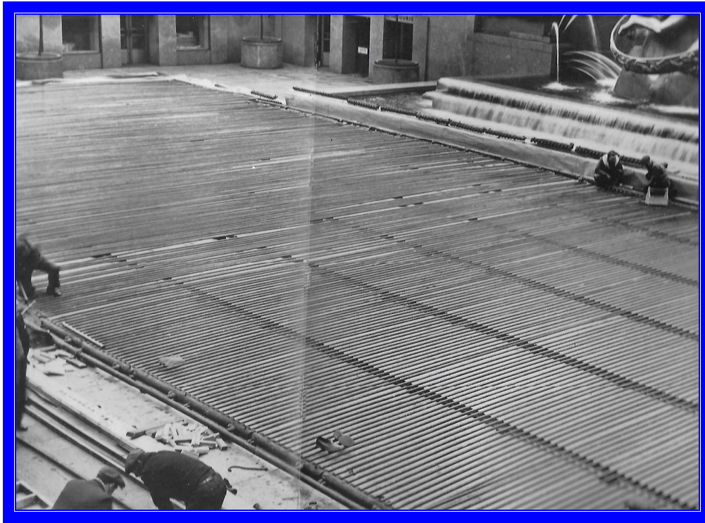
The grid of ice rink freezing pipes being installed in the Lower Plaza in front of the RCA Building. The rink opened Christmas Day 1936 (Works in Progress)
