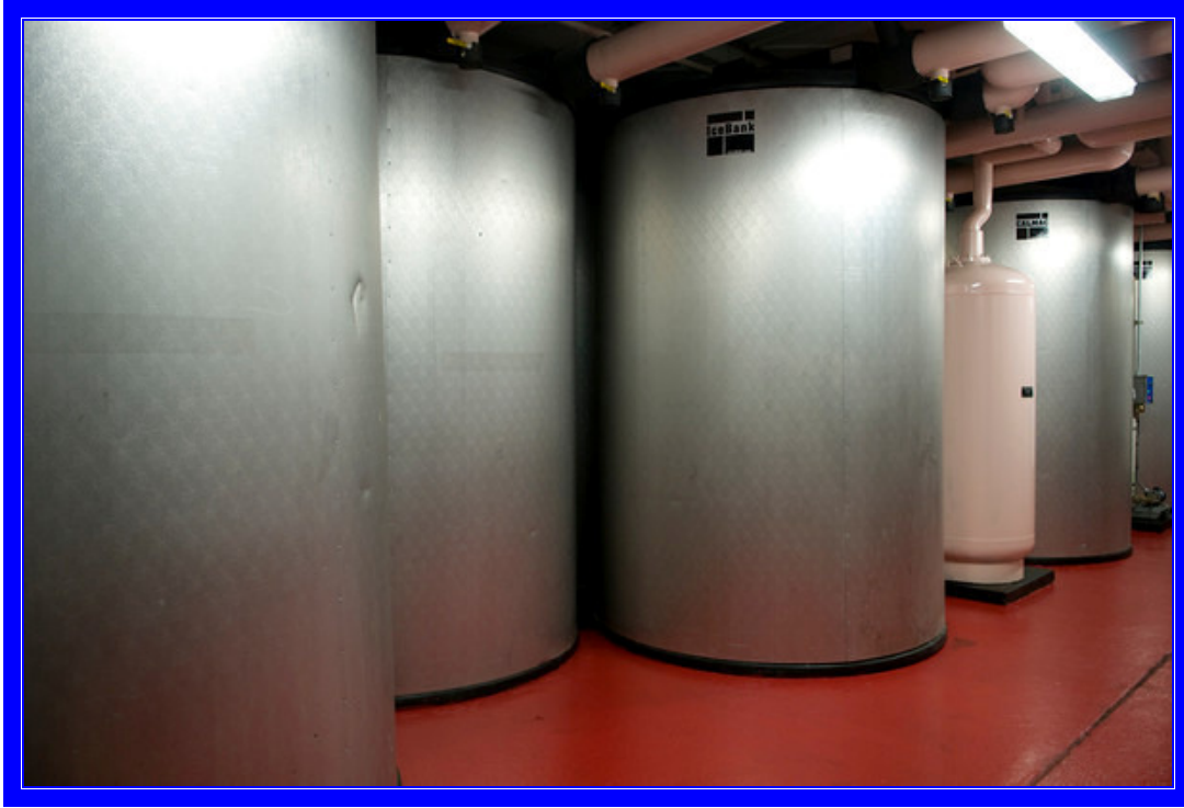
Calmac Ice-Storage Tanks (YouTube & HPAC Engineering 2012))
