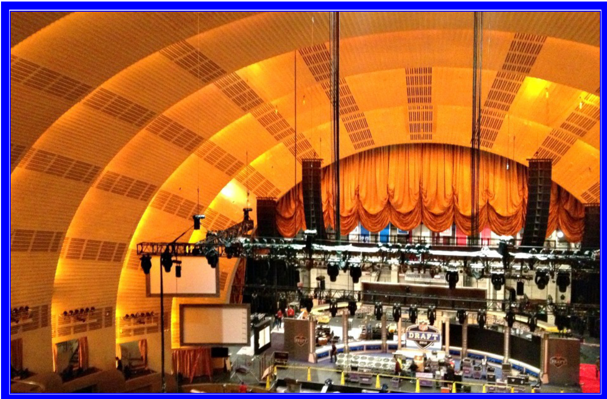
Suspended stage lighting
