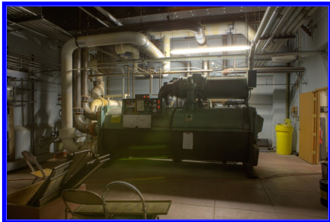
Centrifugal chilled water refrigeration machine
