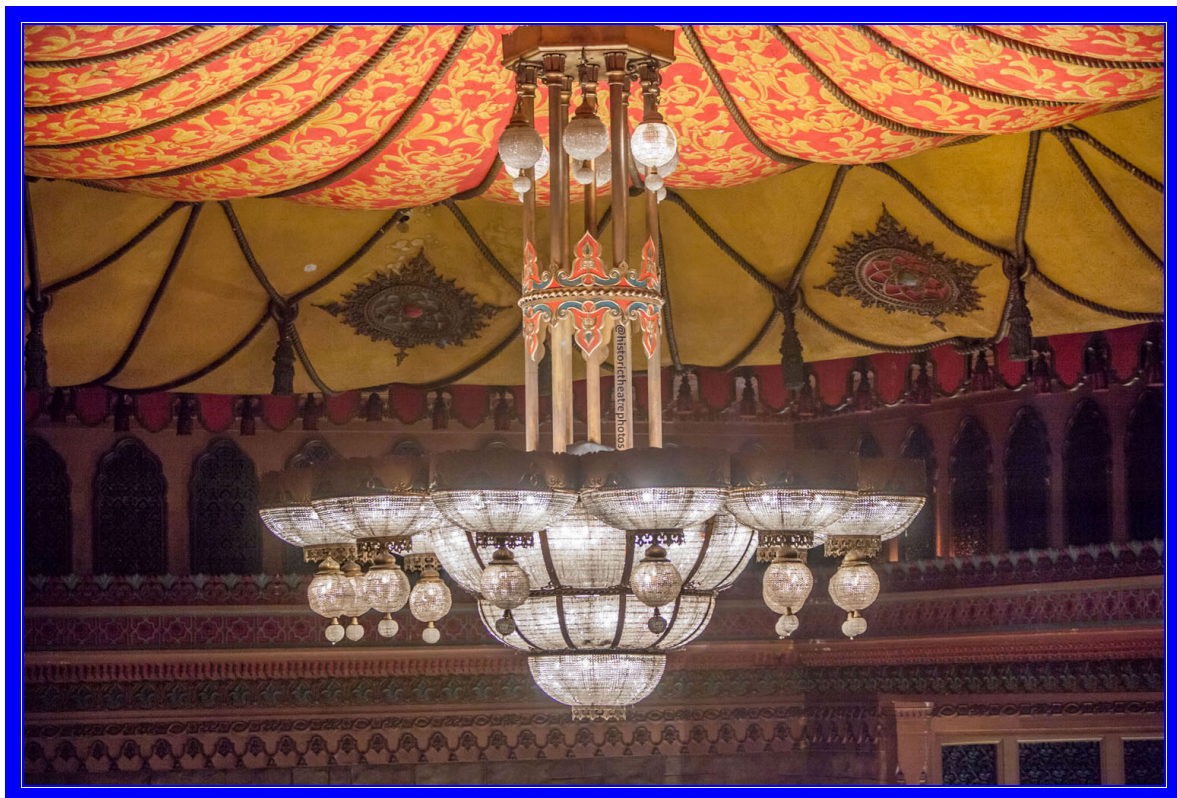
The auditorium chandelier weighing 4 tons with 500 light bulbs in four colours, rated at 64 kW
