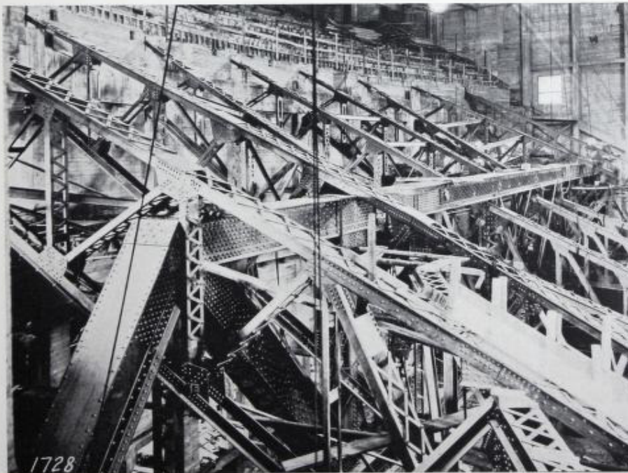
MAIN BALCONY TRUSS AND CANTILEVERS. CANTILEVERS WERE HOISTED TO CAMBERED POSITION. HOLES WERE DRILLED AND MATCHED BEFORE RIVETING. NOTE PIN JOINTS IN UPPER CHORD
