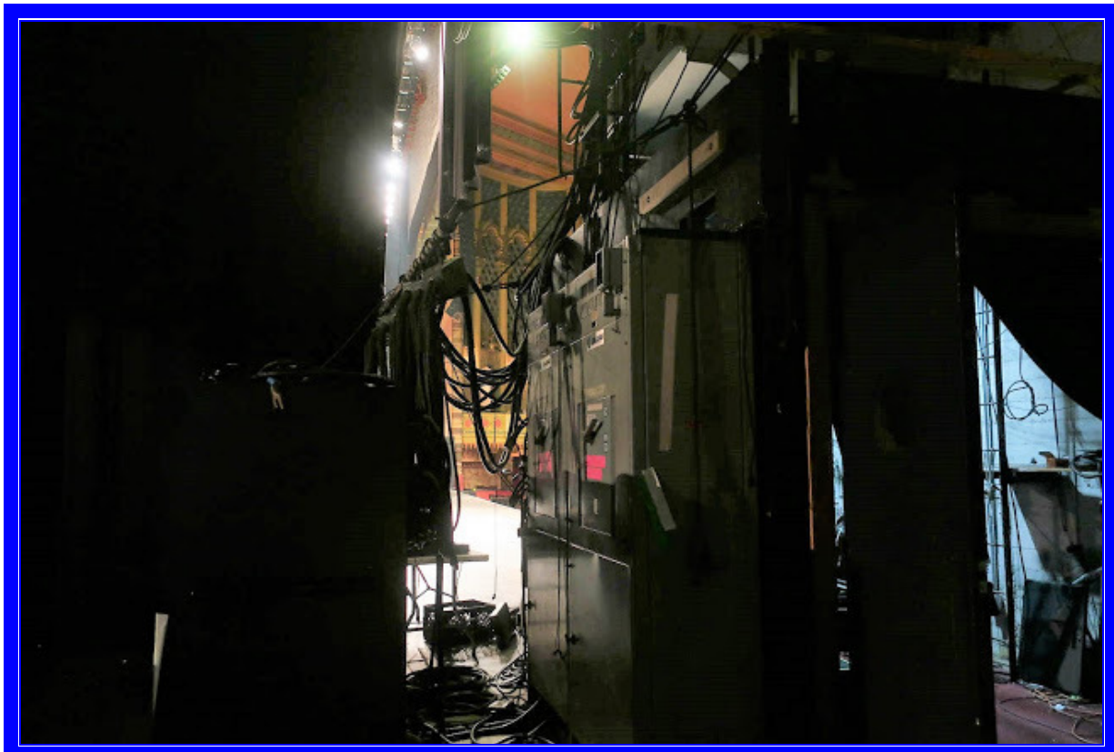
Dimmers and Supply Company switches
