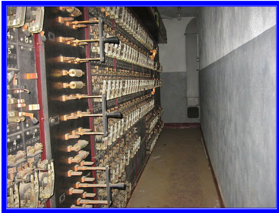
Main fuse board
