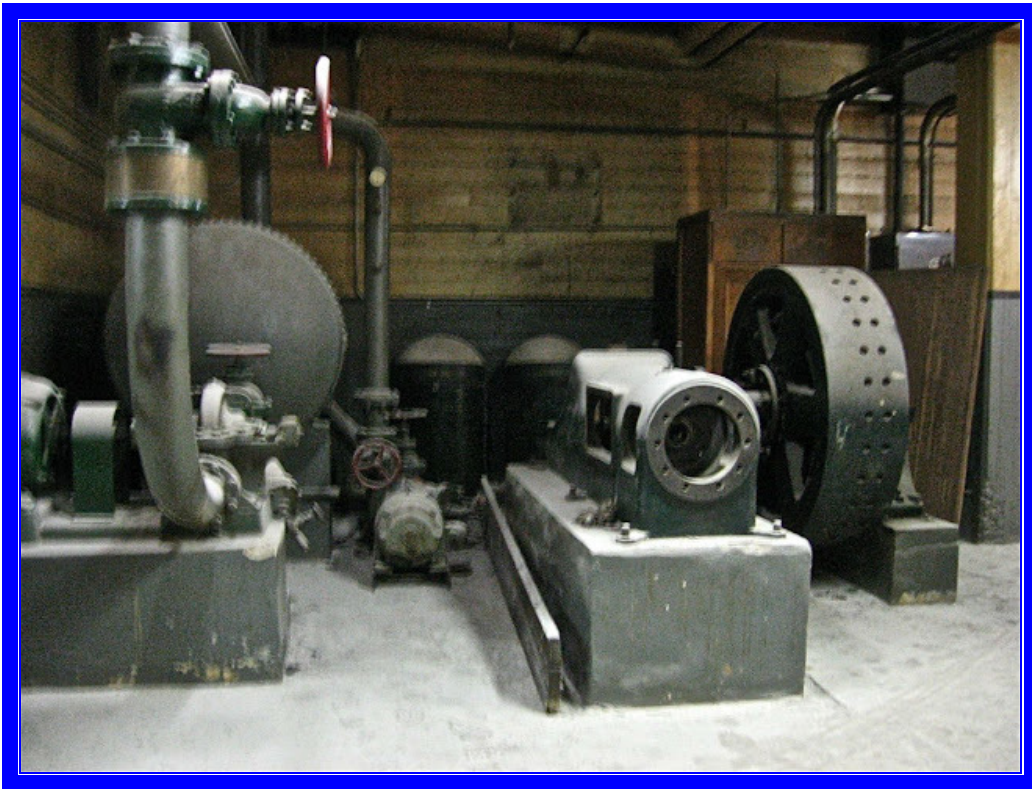
Remains of original ammonia refrigeration compressors
