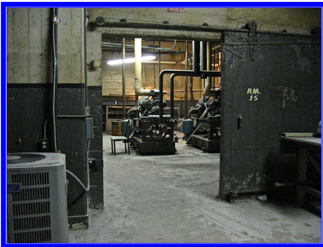
Later refrigeration compressors, believed to date from 1980s
