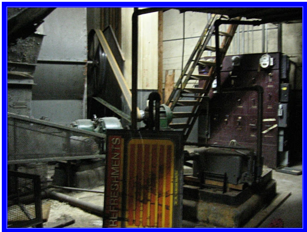
Control panel for mechanical equipment
