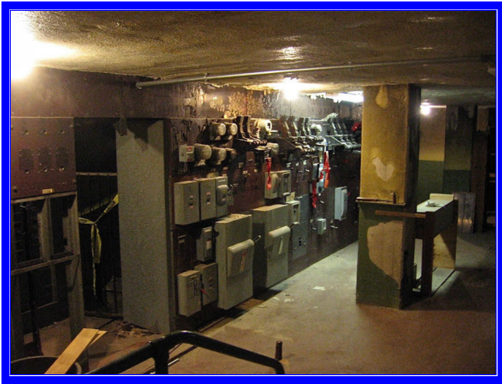
Main electrical switchboard
