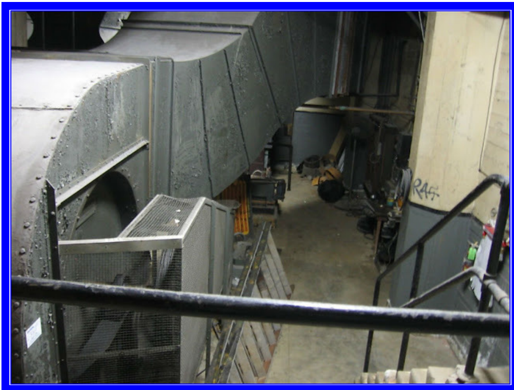
Another view of fan room
