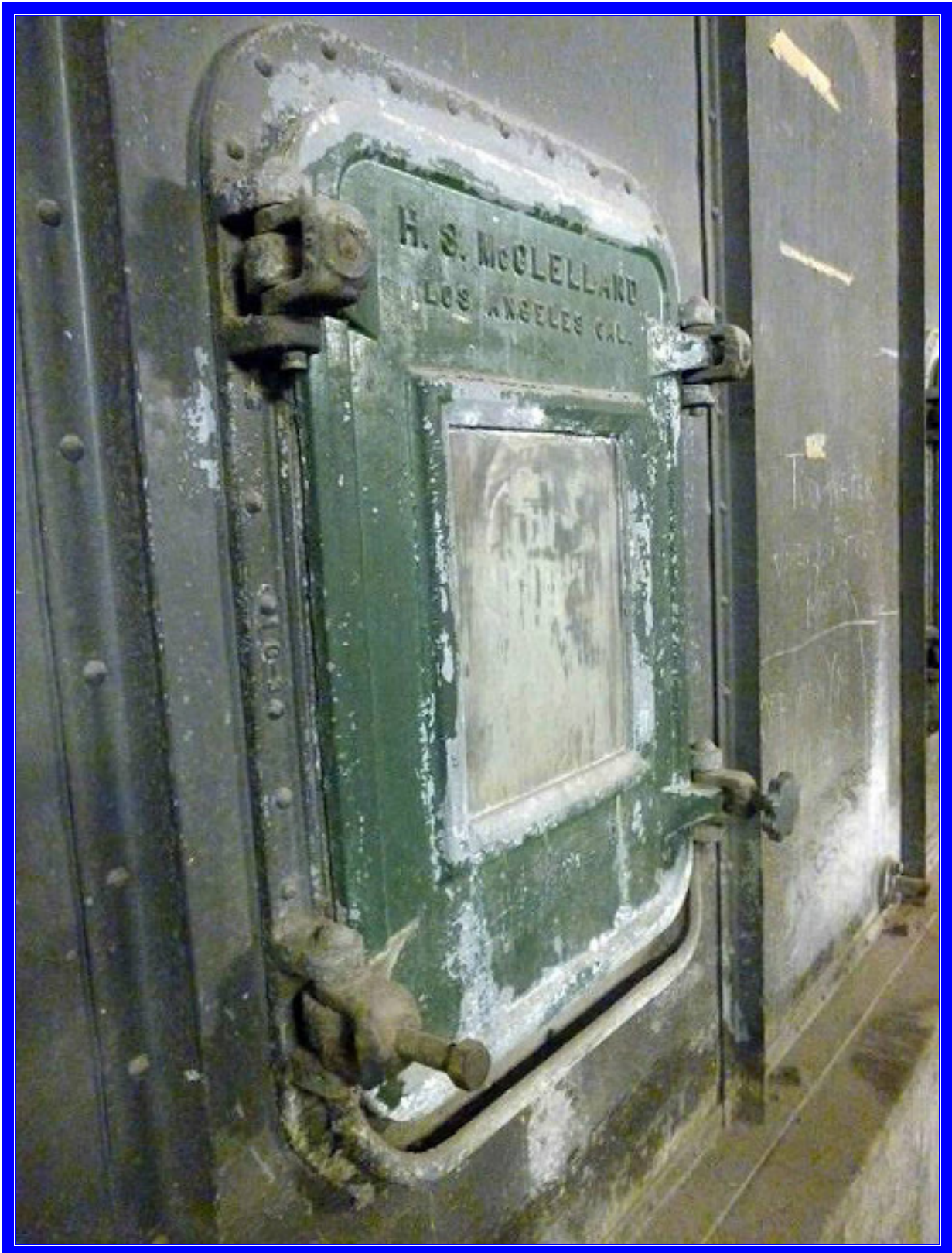
(Original air washer for evaporative cooling)
