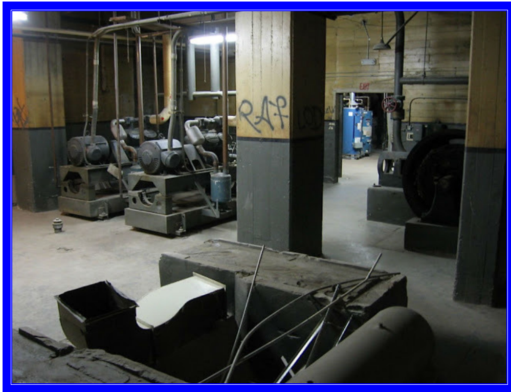
Refrigeration plant room
