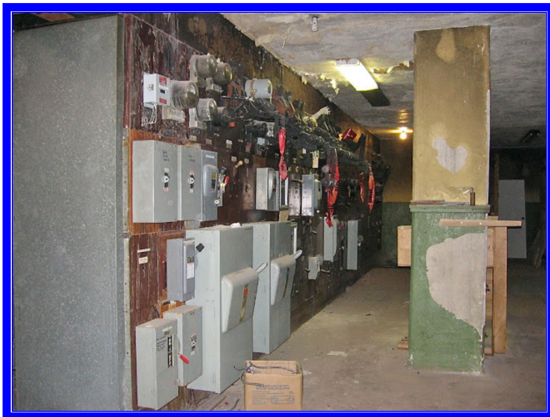
Main electrical switchboard
