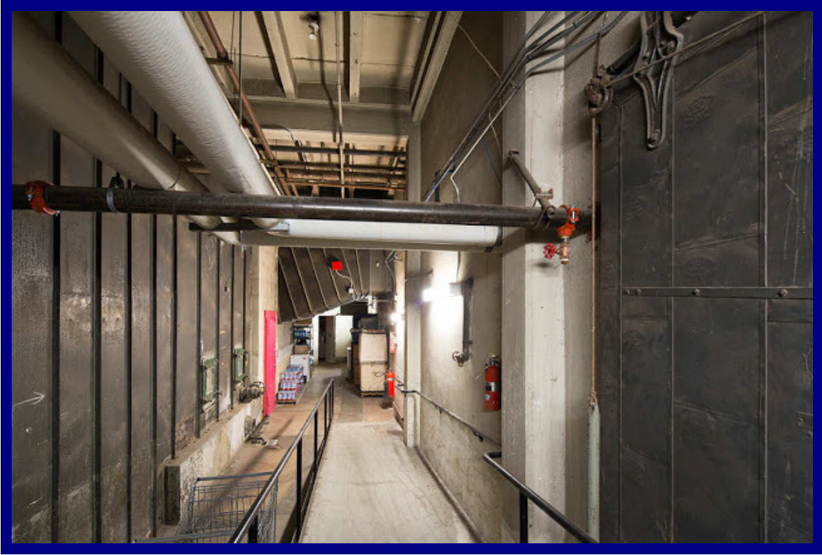
Air washer and supply air ductwork
