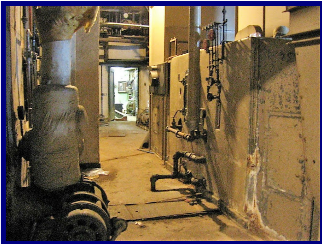
Air washer and steam coils
