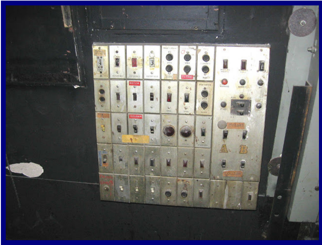
Projection room control panel
