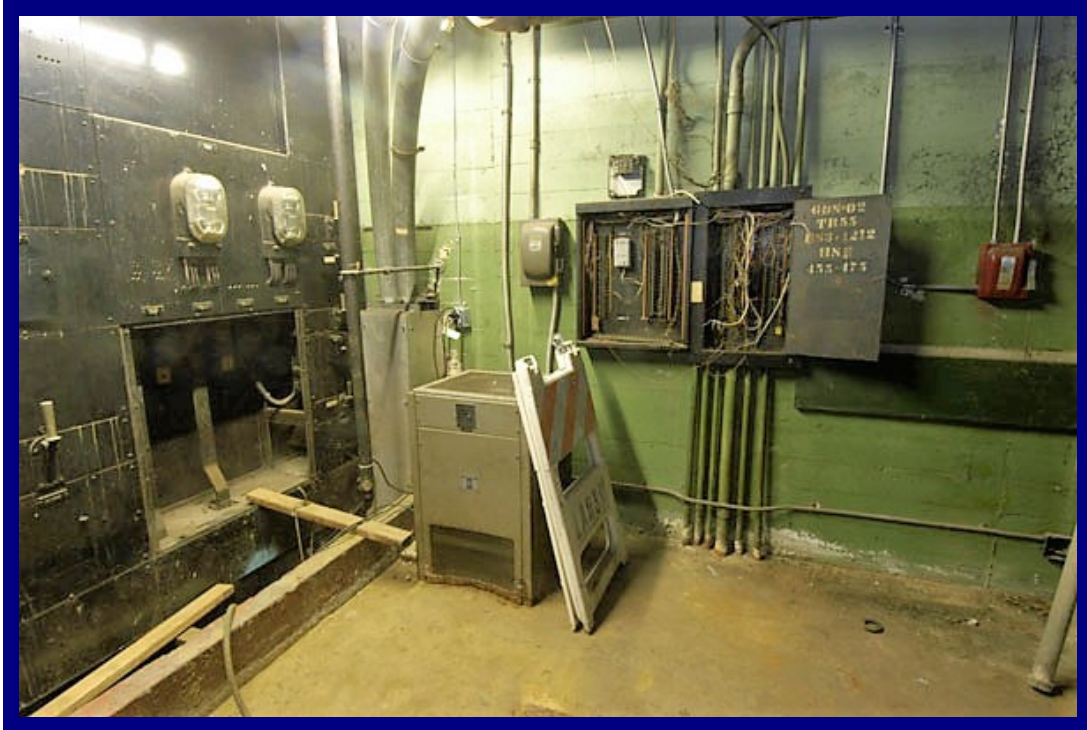
Detail of single phase switchboard (left)
