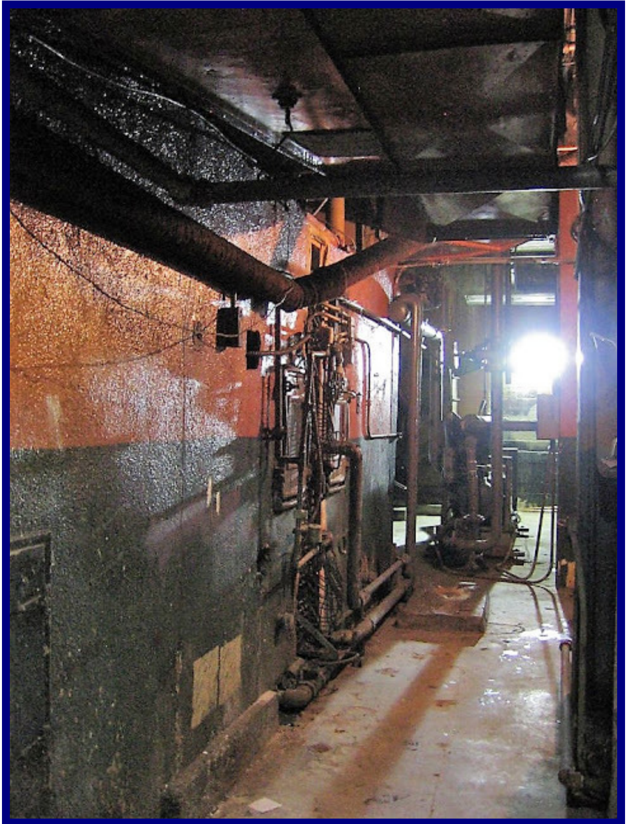
Mechanical equipment room
