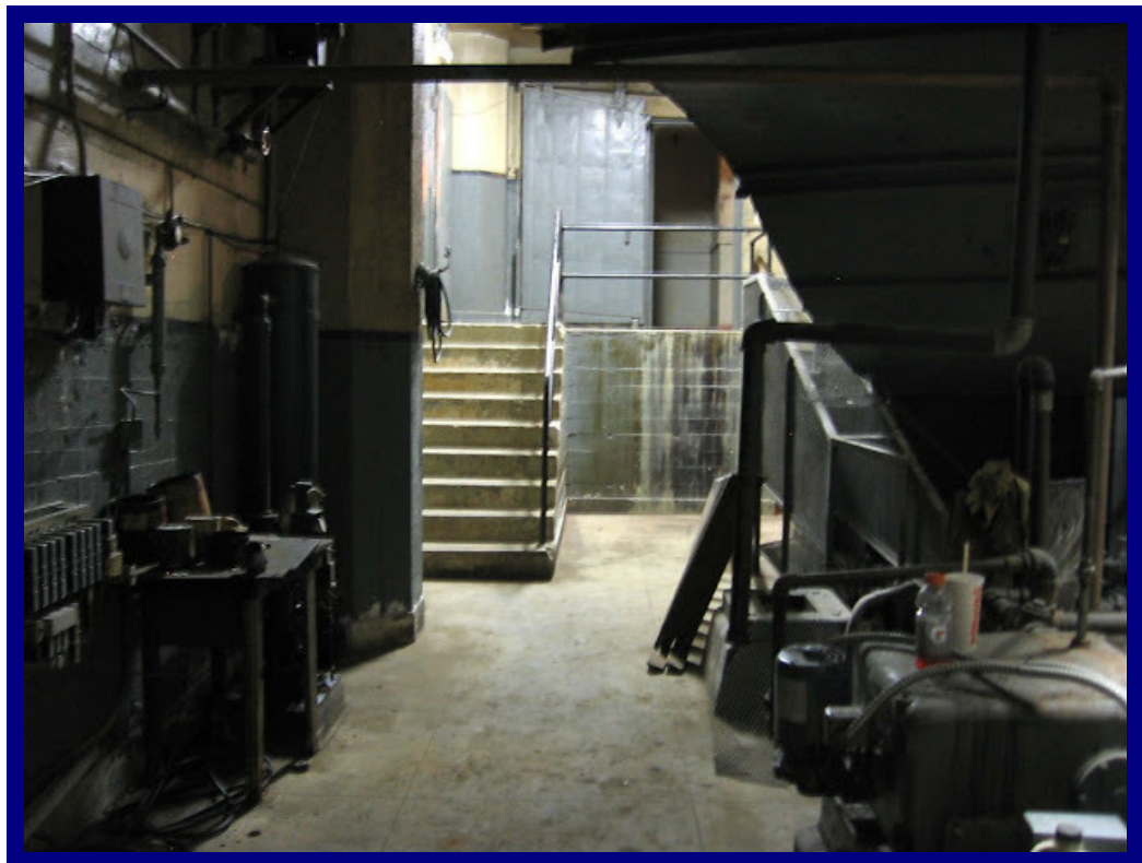
Fan room and distribution ductwork
