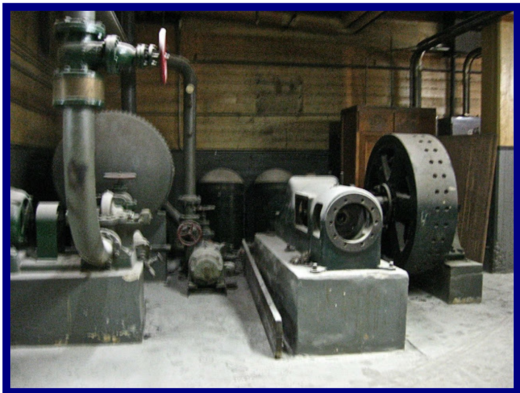
Ammonia refrigerating compressors
