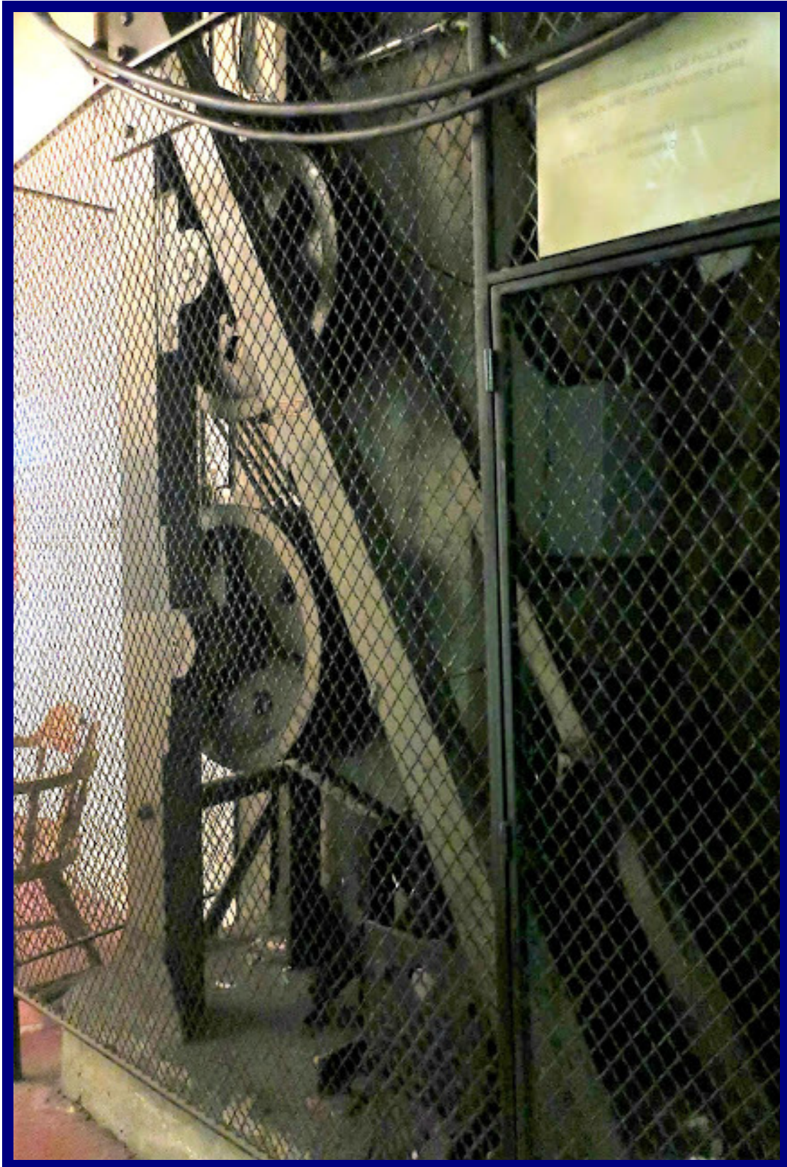
Fire curtain mechanism
