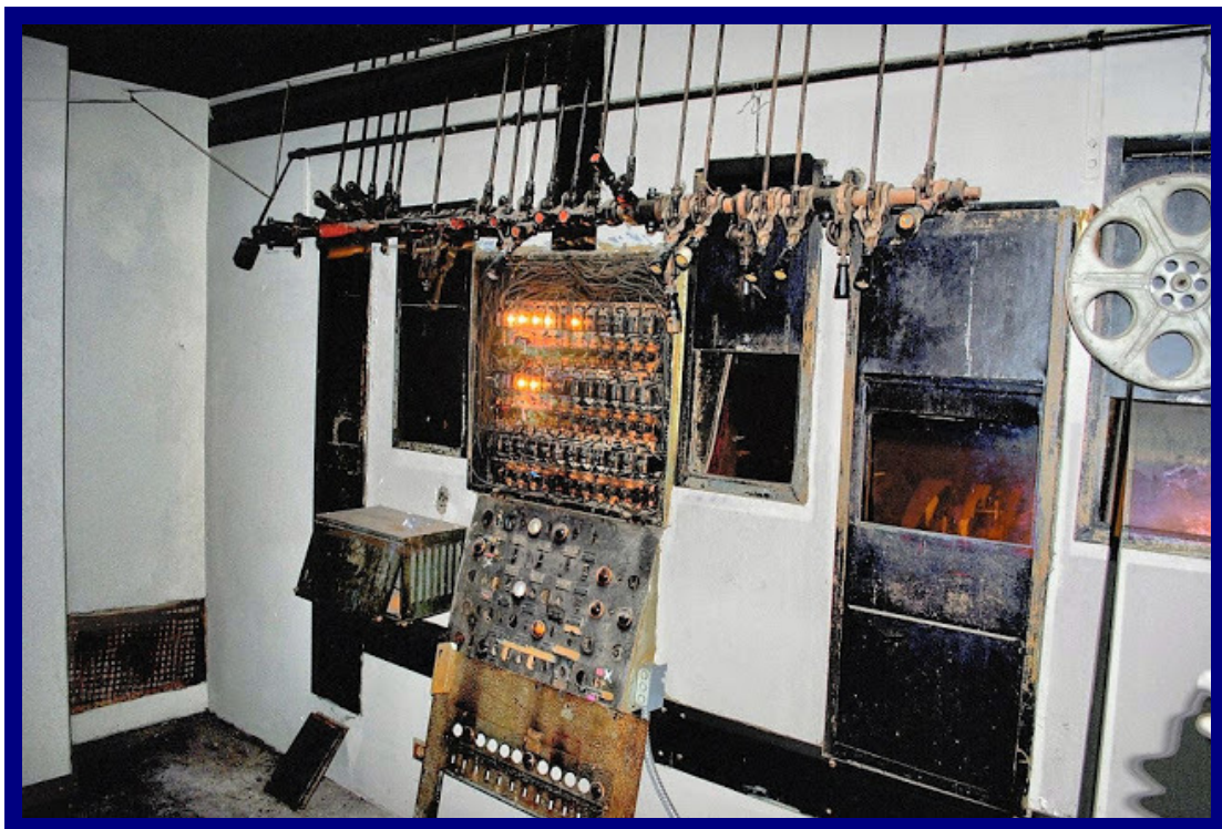
Main lighting control panel
