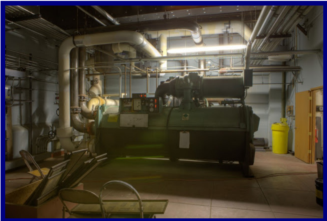
Centrifugal chilled water refrigeration machine
