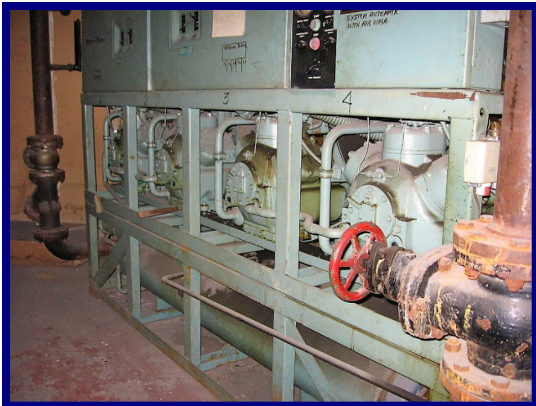
Replacement refrigeration plant
