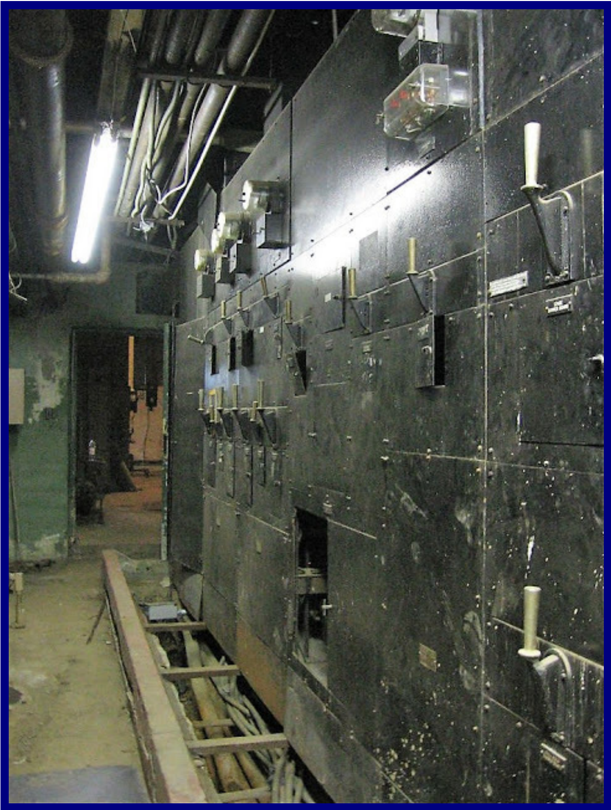
Looking past switchboard into fan room
