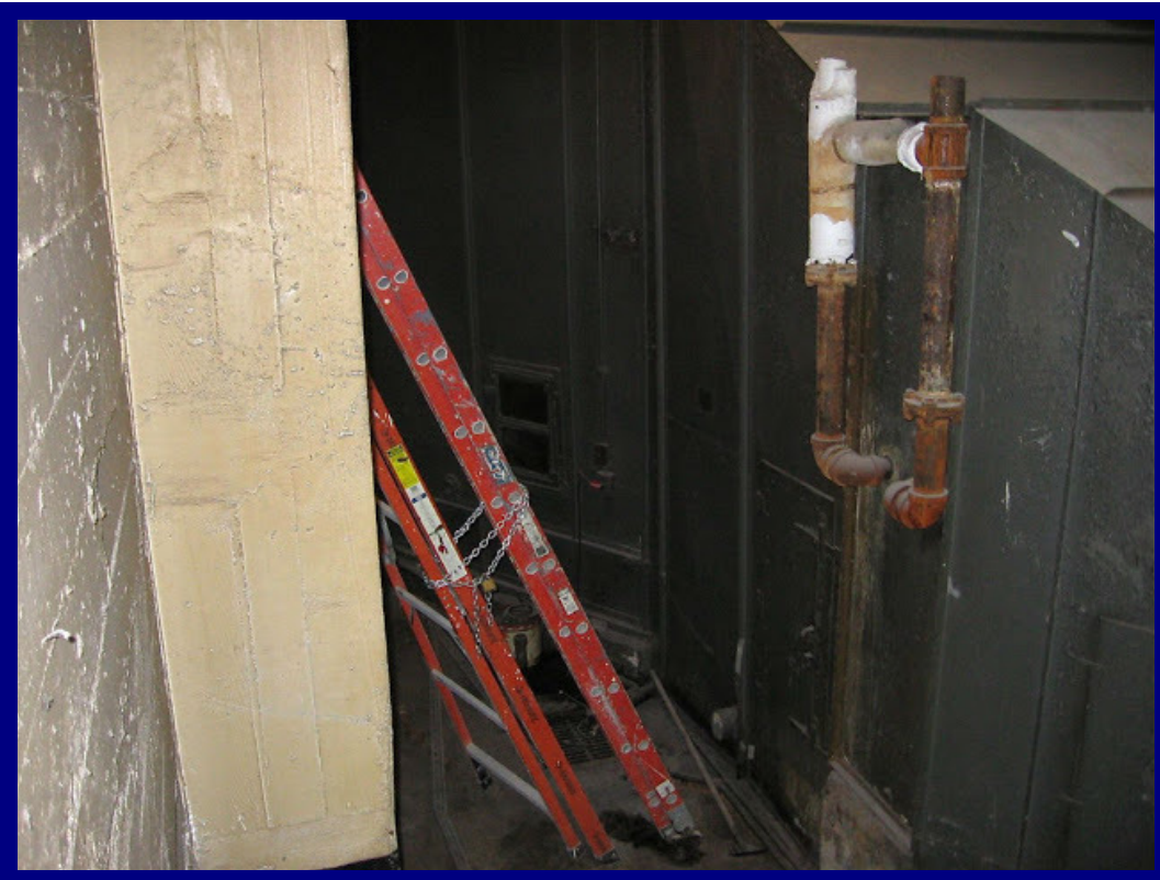
Spray air washer chamber
