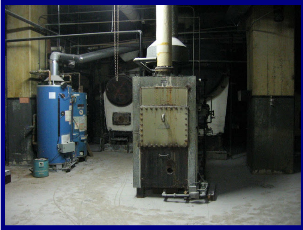
Main boilers (background) with smaller unit (in front) and water heaters (left)
