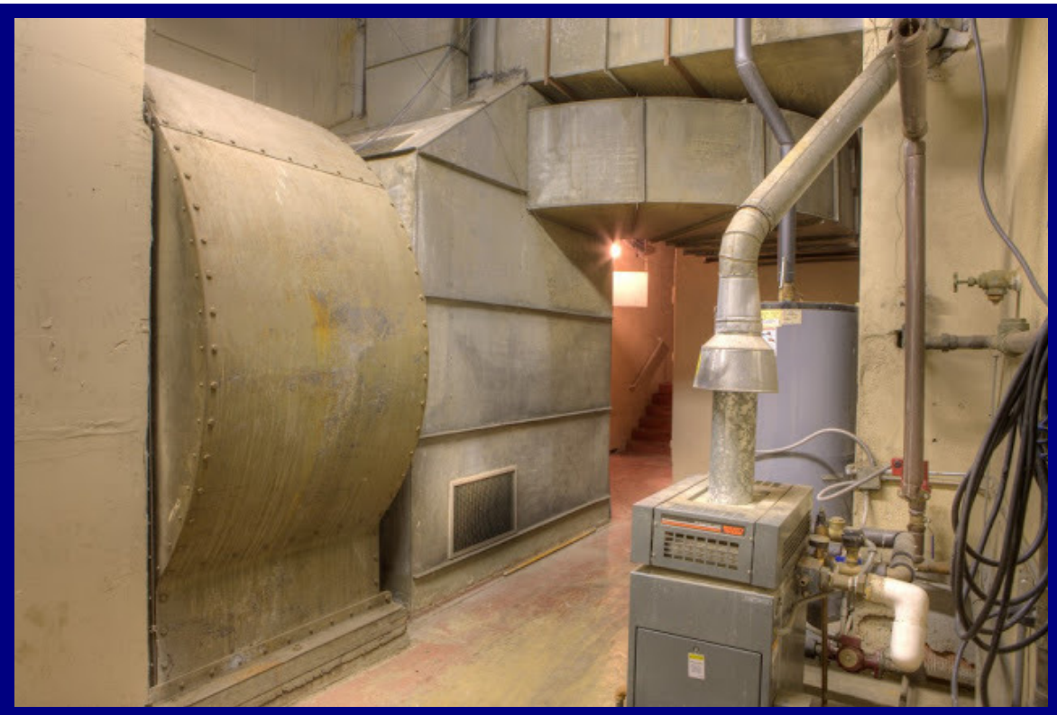
Centrifugal supply fan and water heating plant
