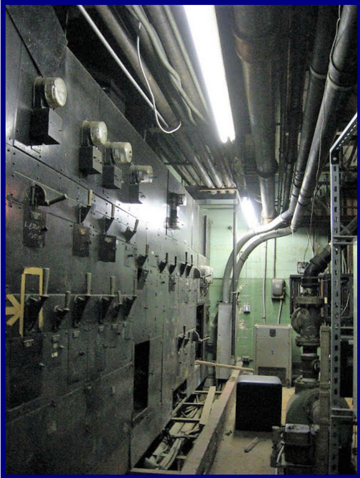
The single phase switchboard
