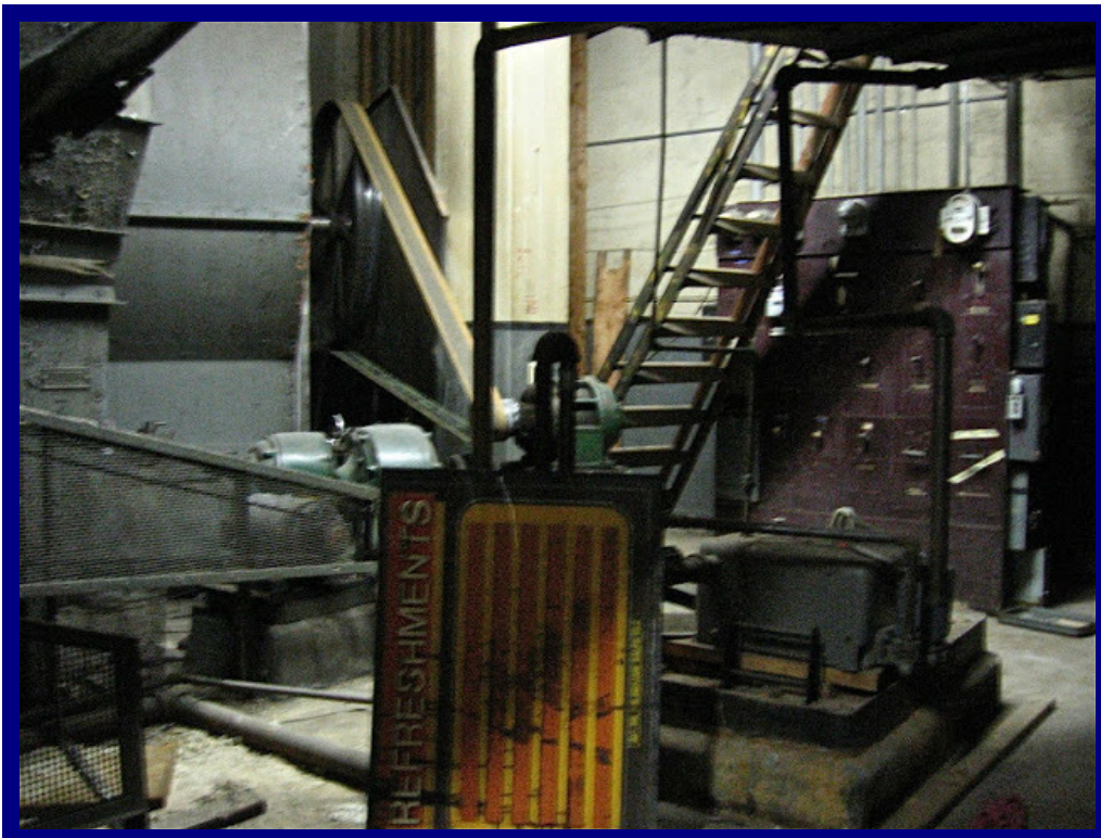
Fan and mechanical equipment control panel
