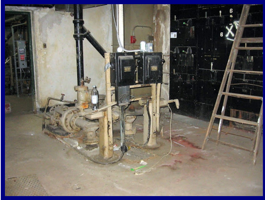
Sump pumps with section of 3-phase switch board
