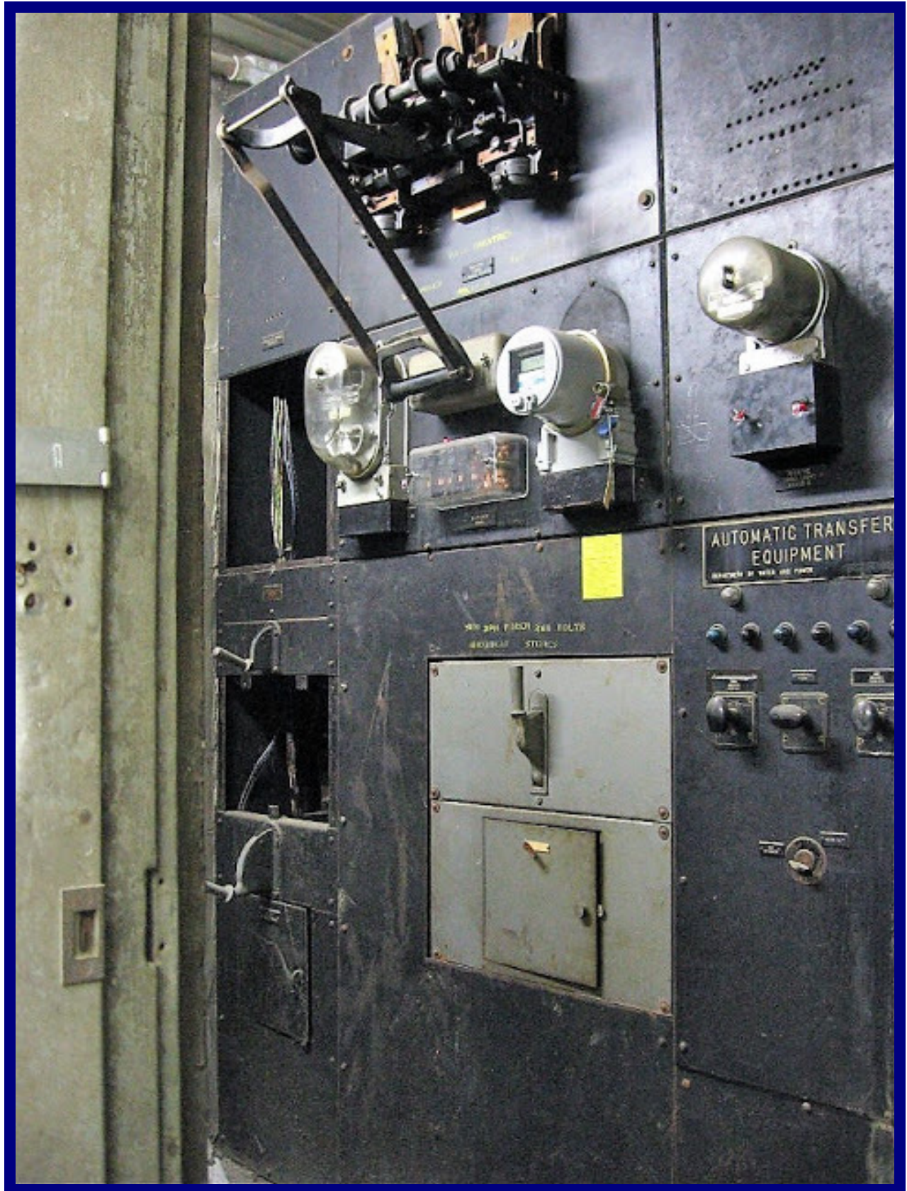
Main 3-phase switchboard
