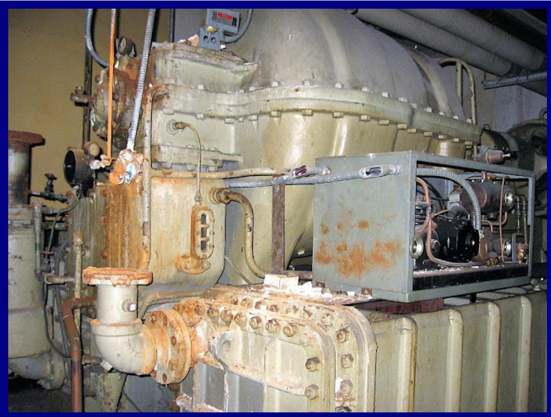
Early Carrier centrifugal chiller with square heat exchangers
