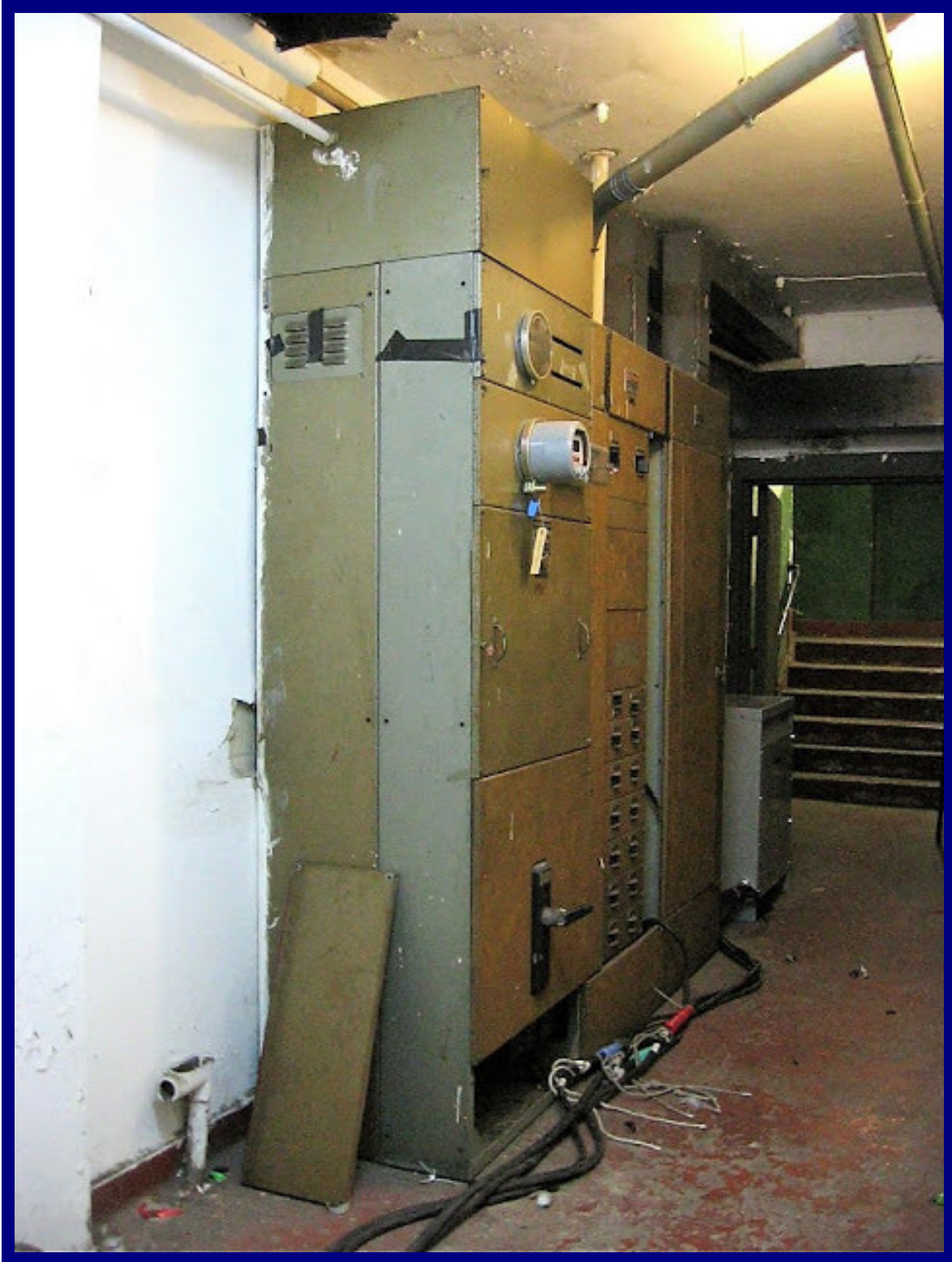
Newer 3-phase switchboard
