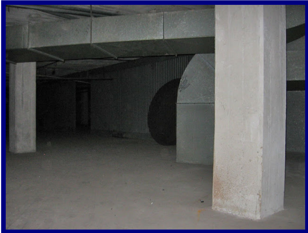
Ductwork system under auditorium
