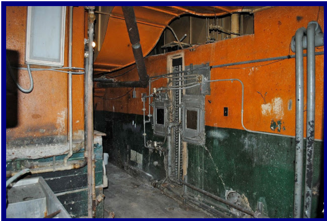
Air conditioning plant
