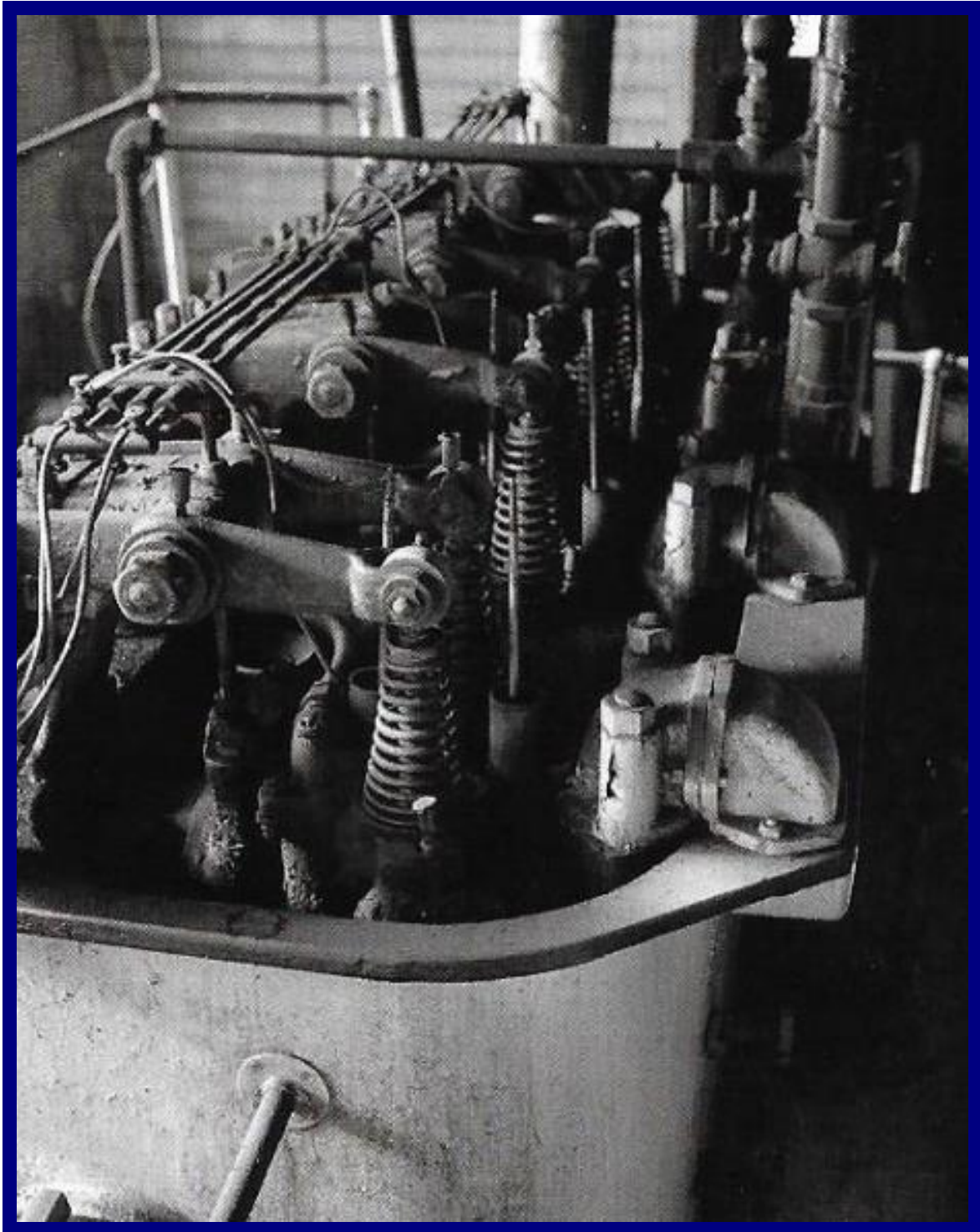
Diesel engine with cover removed
