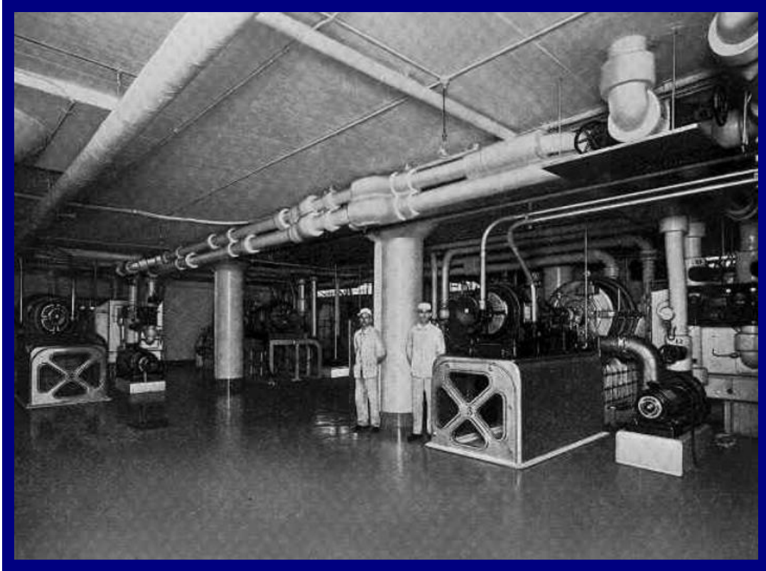
Wrigleys Products Ltd, Wembley c.1928.. Three Carrier centrifugal chillers total capacity 350 TR.
