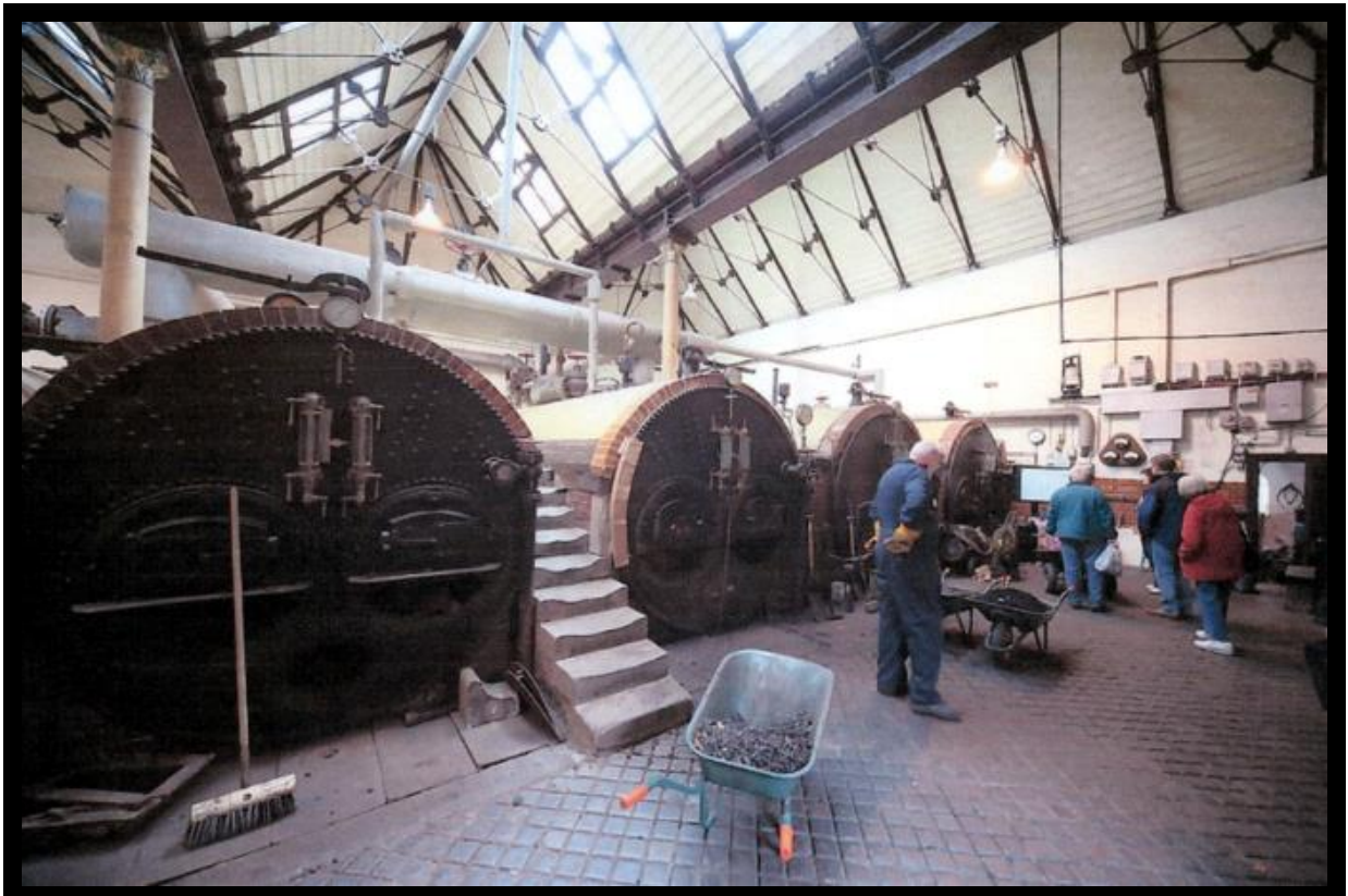
Four Lancashire Steam Boilers at Papplewick Water Pumping Station, now a Museum.
