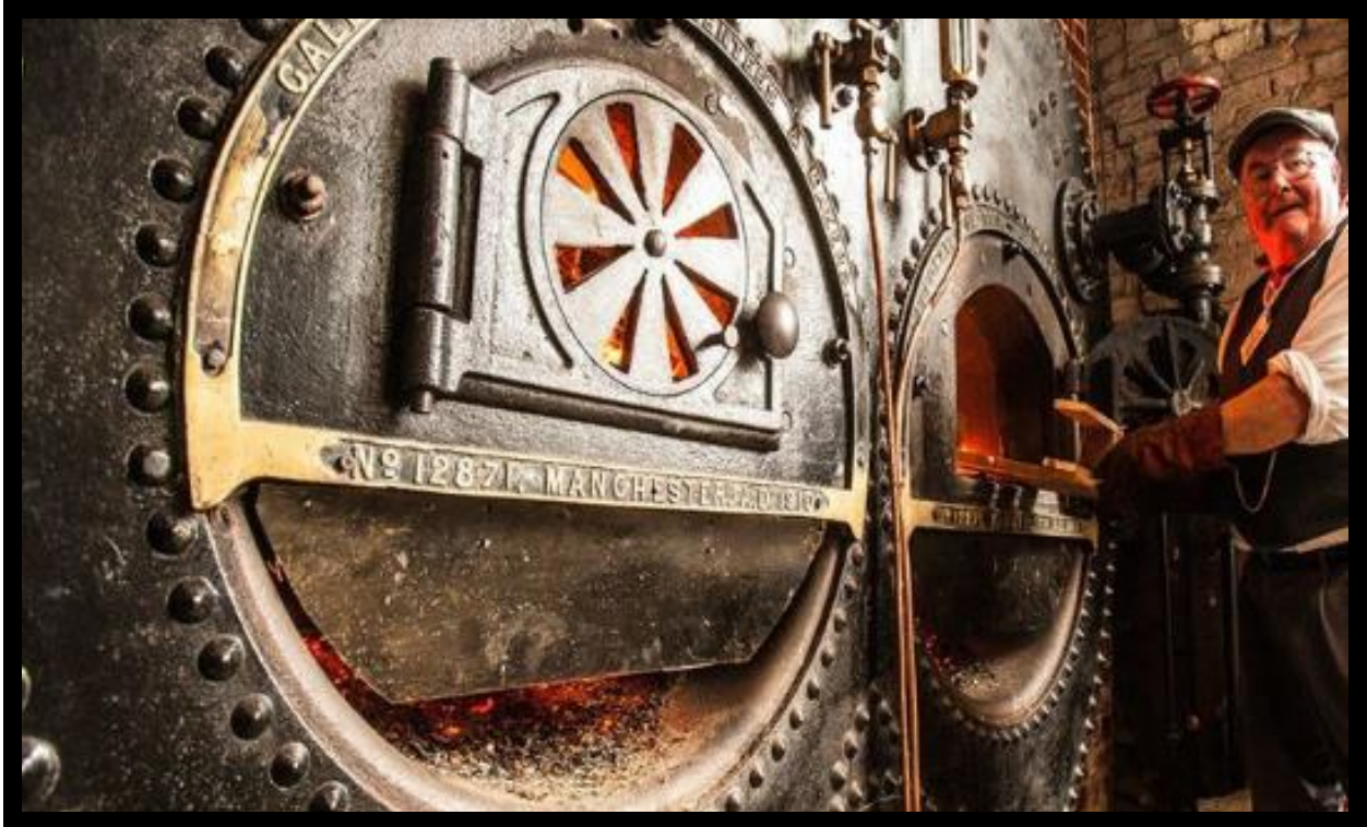
Feeding wood into a Galloway Steam Boiler at Coldharbour Mill in Devon.
