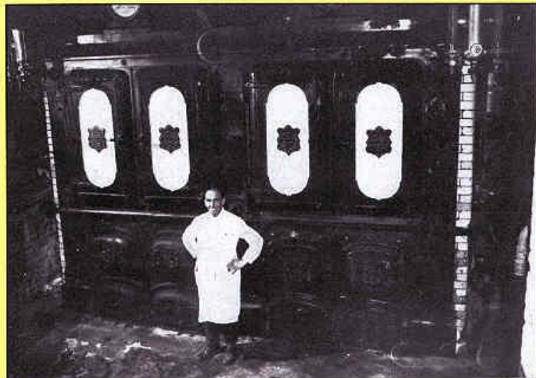
Babcock & Wilcox Boiler Installation at the National Liberal Club, Westminster, London, 1887. [Brian Roberts Collection]
