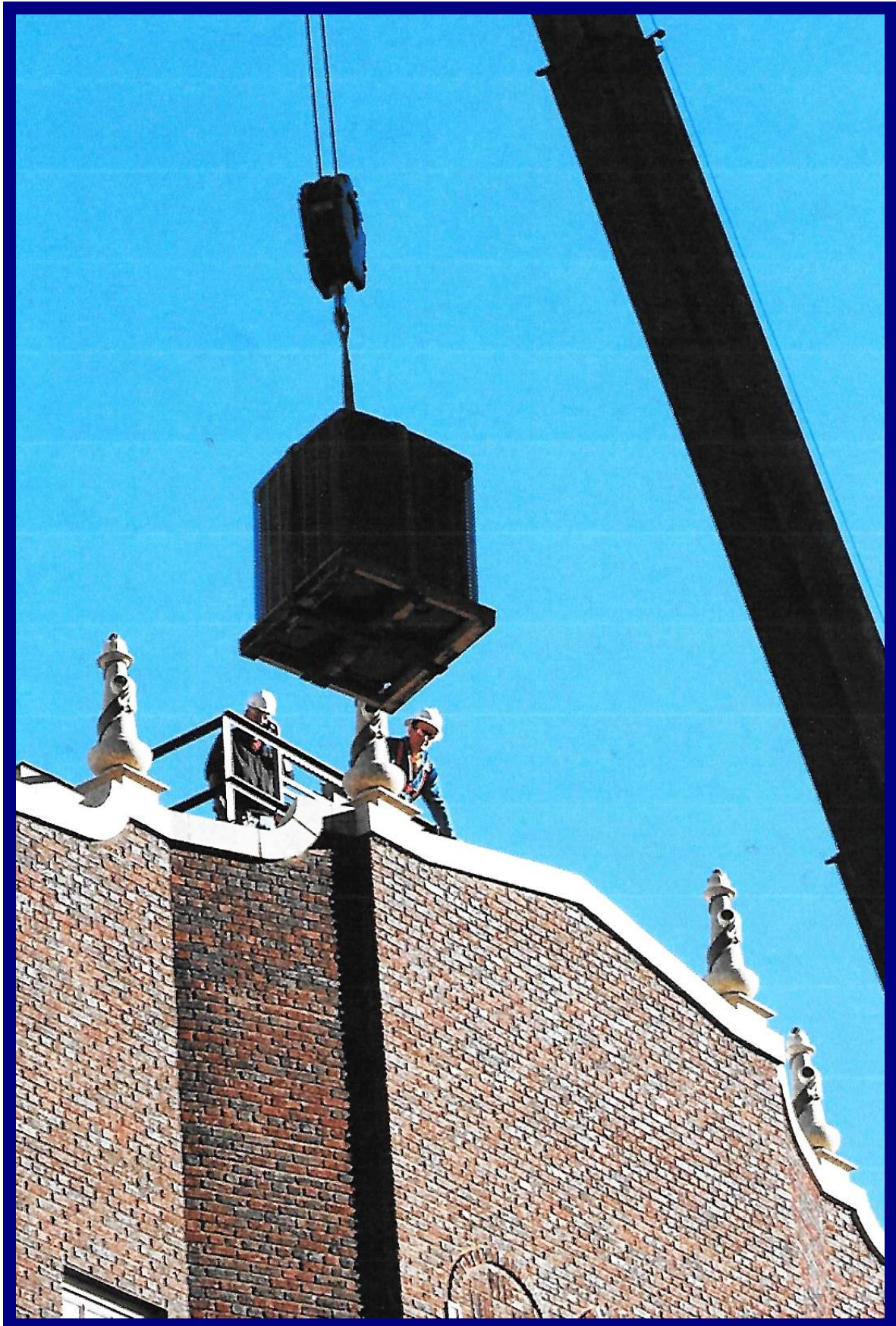
An air conditioning unit for the projection booth is hoisted to the roof in 2000.
