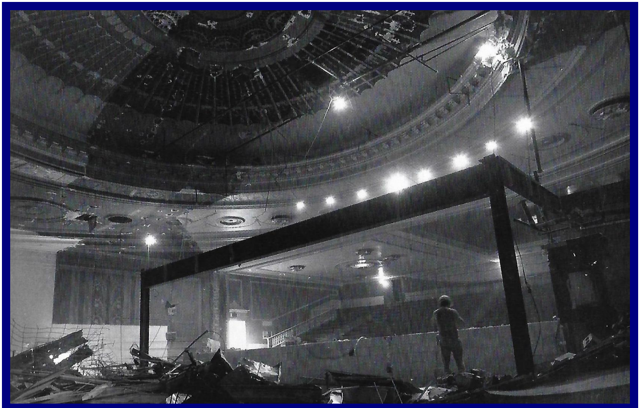
The sorry state of the auditorium as the 1970s restoration gets underway.
