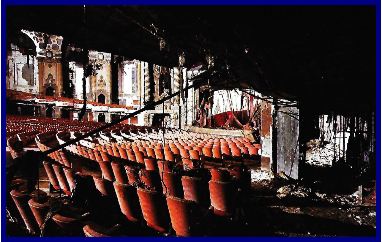
The collapsed balcony plasterwork in about 2009.
