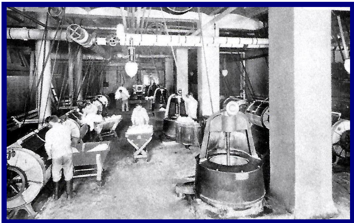
The Laundry, also on the basement level, capable of handling 65,000 pieces of bed and bath linens, tablecloths and napkins. Guest laundry and dry cleaning were located on upper floors. ("On the sub-basement, below the kitchen and laundry, were the hotel's steam-heat systems, hot-water boilers and electric power dynamos".)
