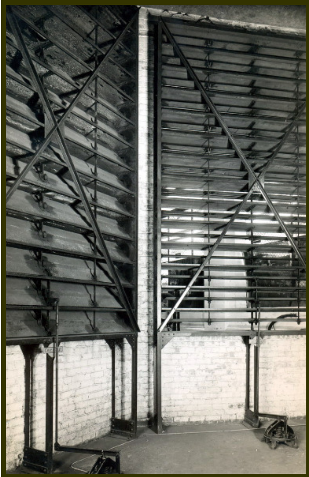
Air conditioning system mixing dampers, Bedford Mill Weaving Shed 1949.
