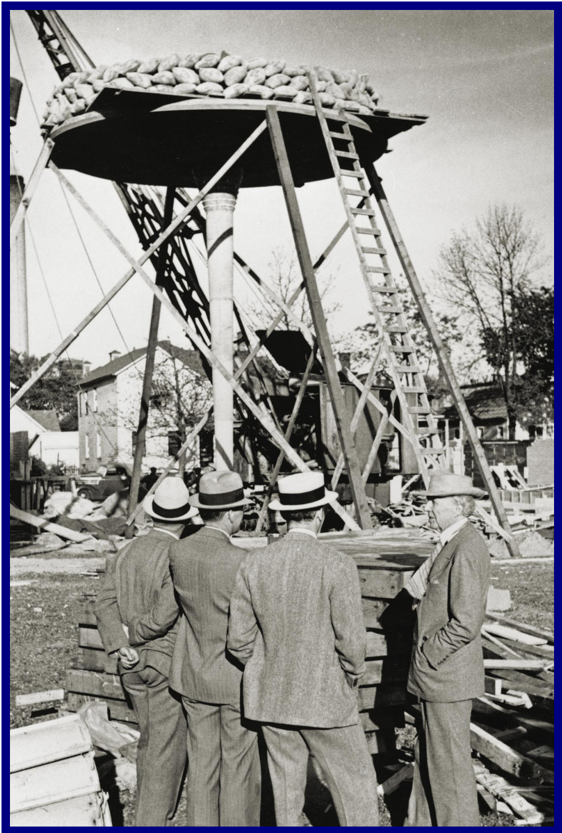
Wright witnessing a successful load test on one of his unusual mushroom structural columns. These were 21 ft high; the circular pad was 20 ft in diameter, the column tapering downwards to 9 inches in diameter, the pads interconnected at their tangent point to form a rigid frame.
