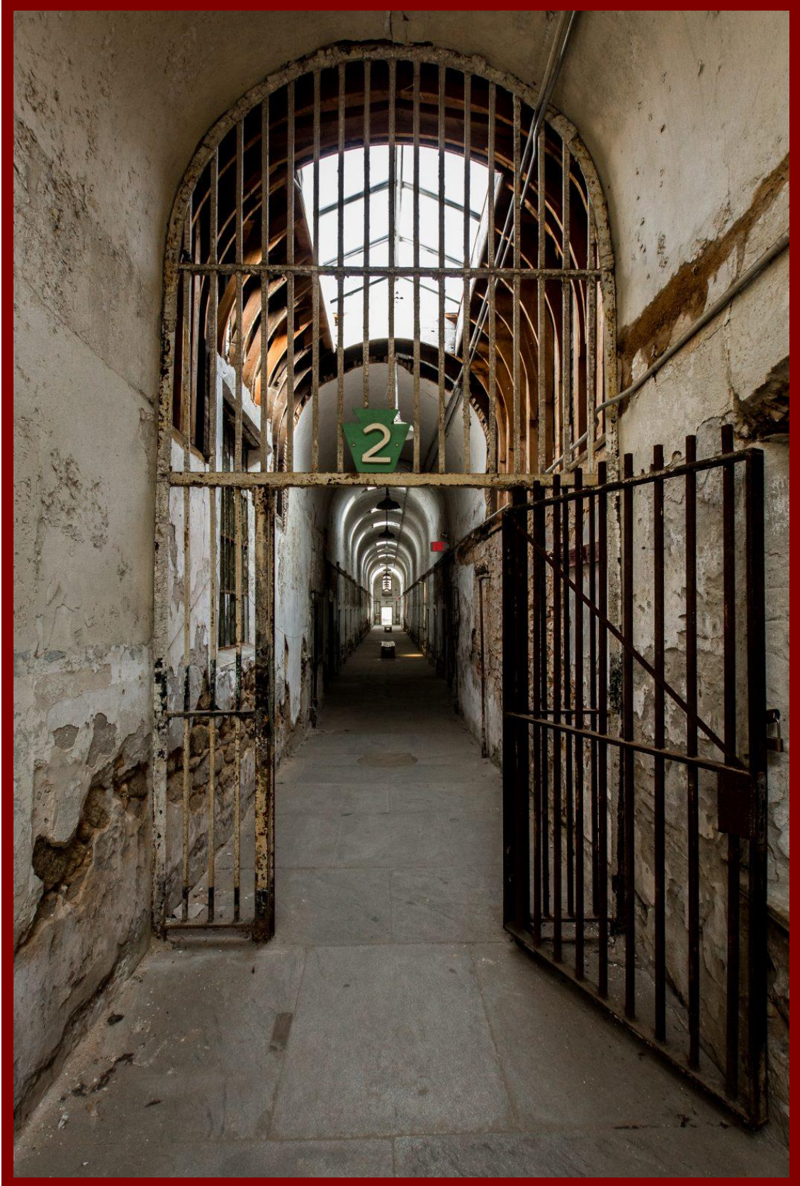
A crumbling corridor.
