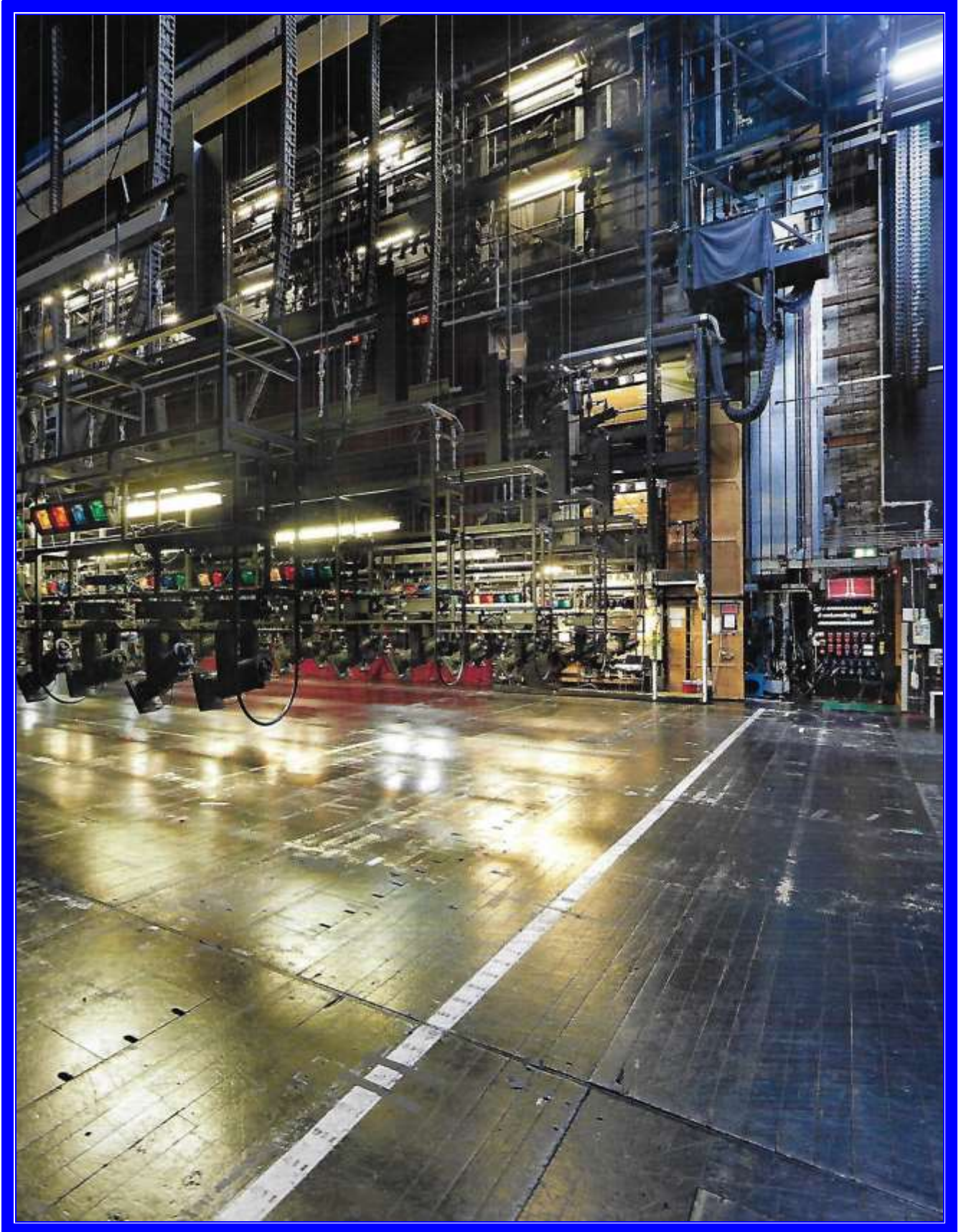
The Royal Opera House, Covent Garden, London, stage lighting and controls ( London Theatres ).
