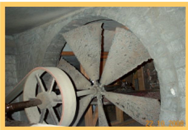
Supply fan belt drive showing propeller fan blades
