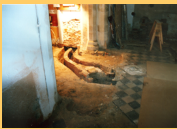
Underfloor flue ducts from cover plate A to Tower North Wall (exposed in 1997)
