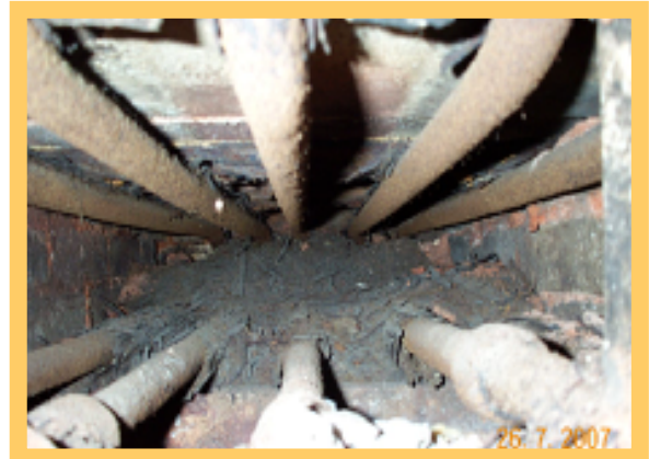
Pipe coils inside brickwork furnace
