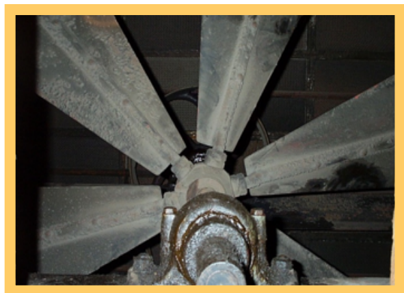
View along drive shaft to fan blades
