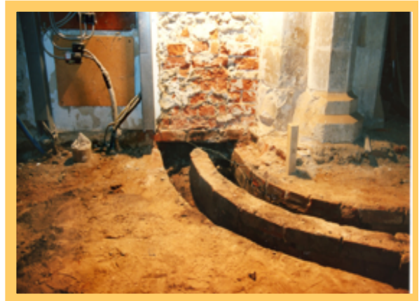
Underfloor flue ducts from cover plate A to Tower North Wall (exposed in 1997)
