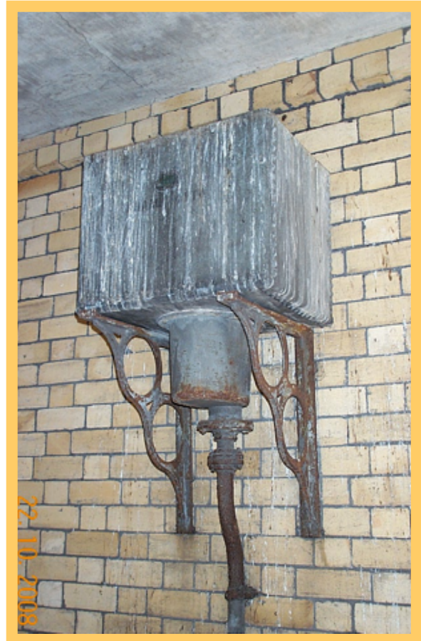
Original cold water storage tank supplying washer
