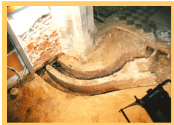
Underfloor flue ducts from cover plate A to Tower North Wall (exposed in 1997)
