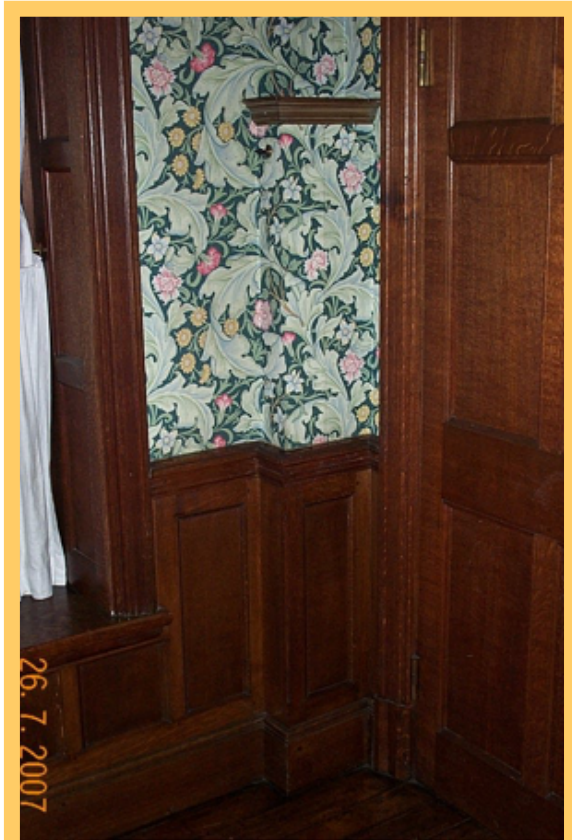
This tube has been carefully concealed within the timber and wallpaper. The timber top frame is evidence of its position
