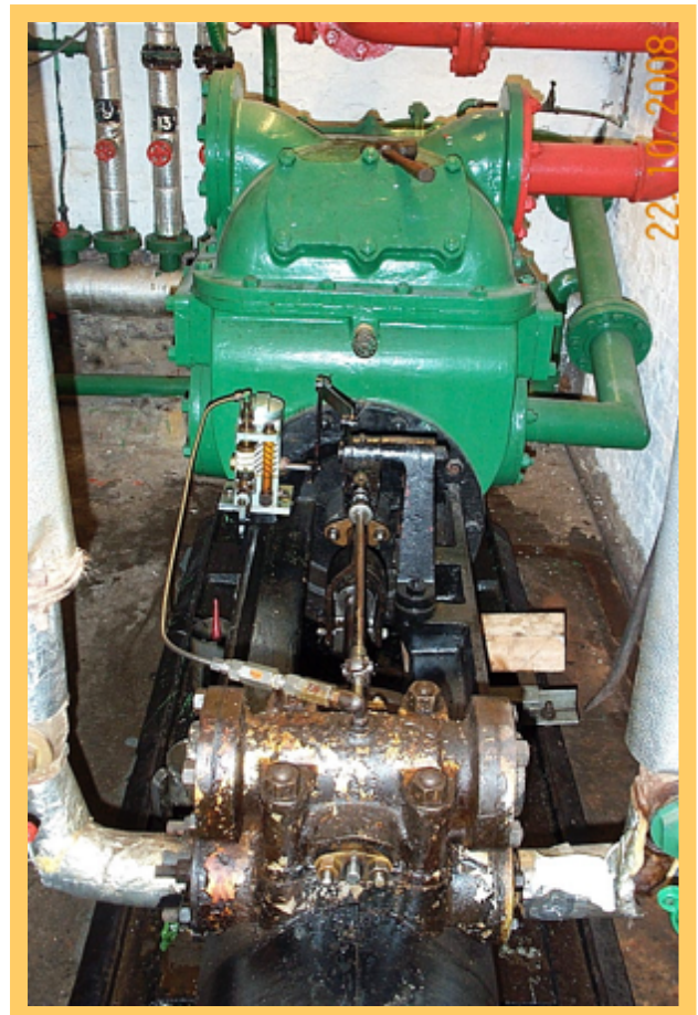
Right side Vacuum Pump
