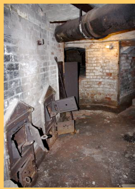
General view of the furnace room
