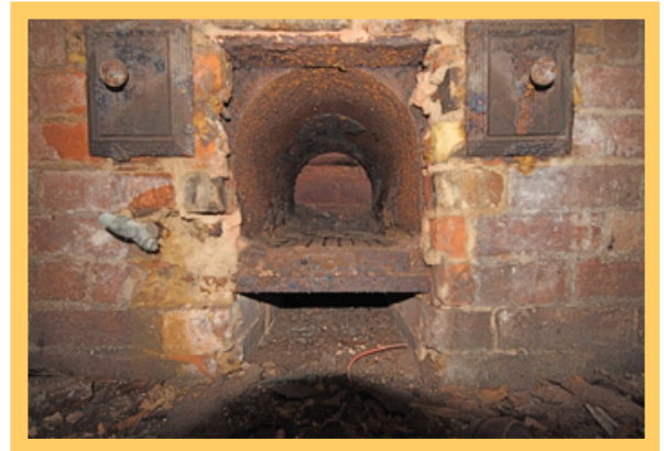
Face-on view showing the saddle boiler with the fire-grate and ash pit below
