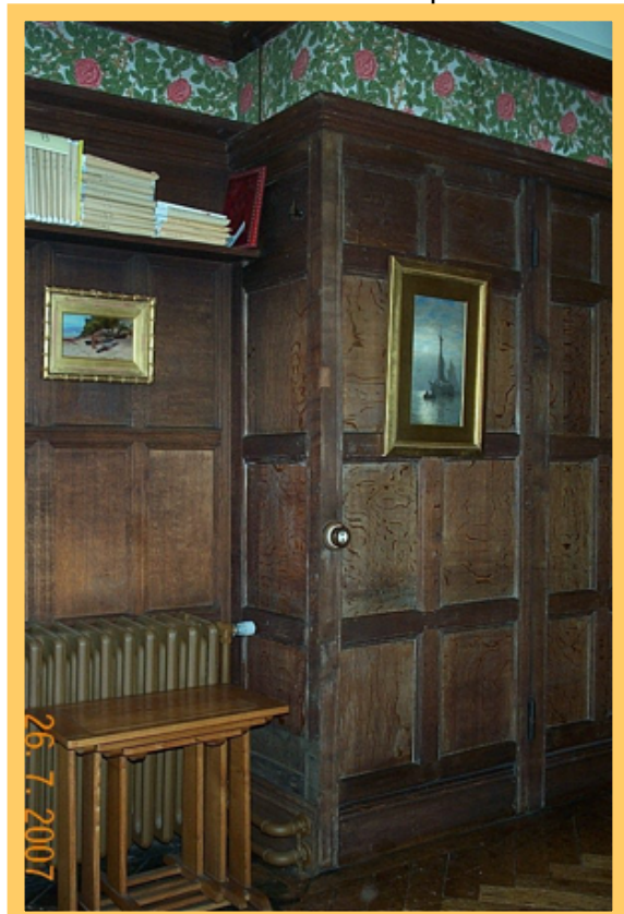
This tube has been hidden behind the timber panelling. The top of the tube is at the level of the timber moulding. Note the careful concealment of the control damper.
