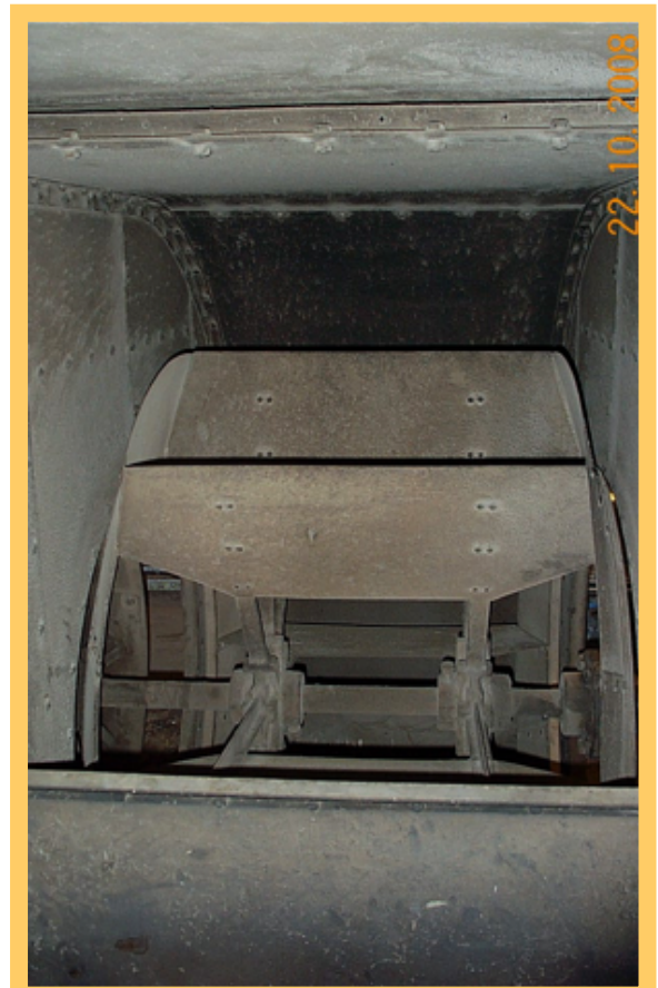
Looking into discharge outlet an extract fan
