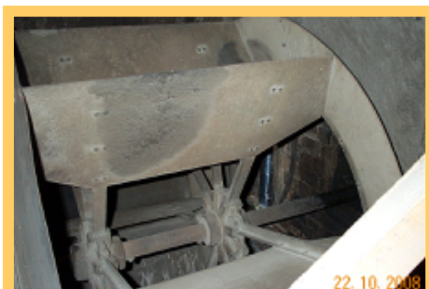
Looking into discharge outlet one extract fan
