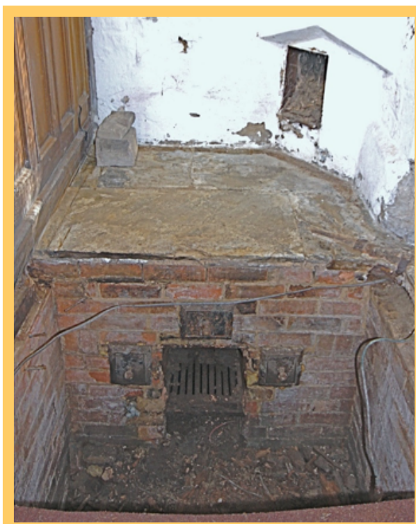
View into floor-pit facing the furnace. Note the pipework partially buried in the floor on the right-hand side
