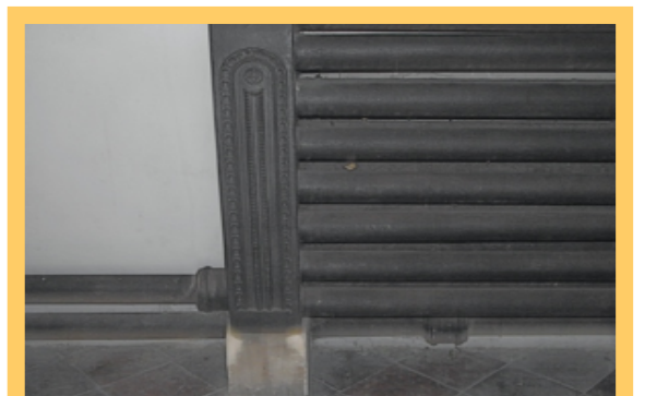
All the pipe coil heaters have decorative end header boxes.
