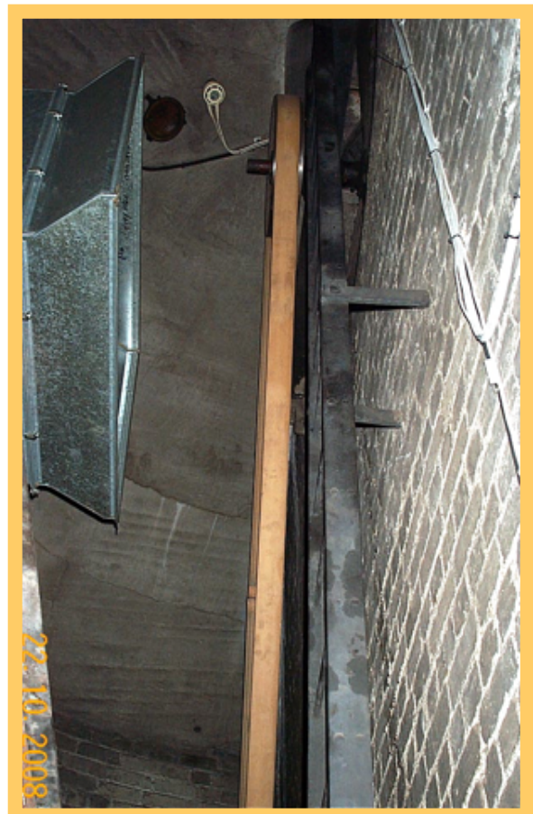
Extended belt drive to the supply fan
