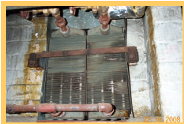
Steam & Condensate pipework to heater battery
