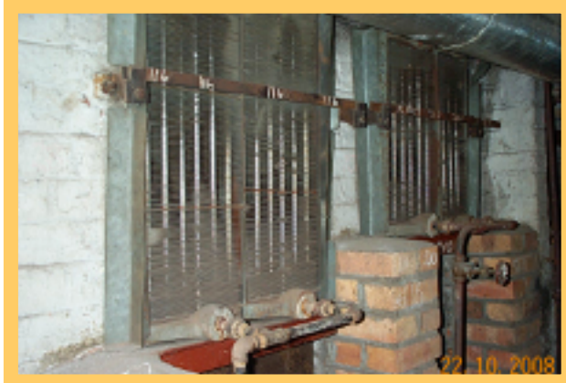
Pairs of finned steam heater batteries
