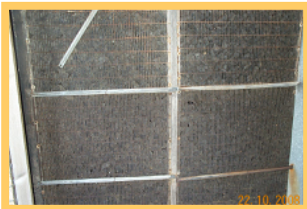
Six banks of filter cells filled with coke
