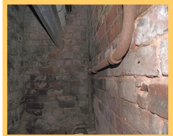
Pipe circuits on side of furnace brickwork
