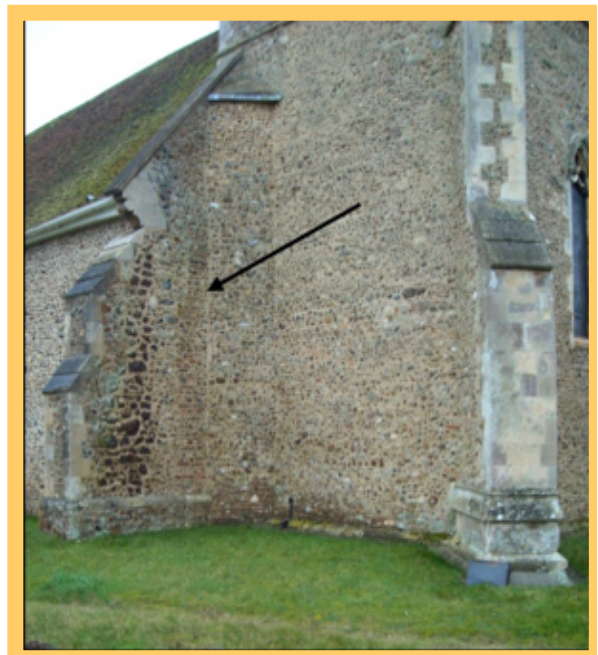
The arrow indicates the position of the angled quoin locating the likely position of the hypocaust A metal plate now covers the top of the quoin / chimney. The original chimney must have been much higher built against the wall of the tower but has since been demolished.
