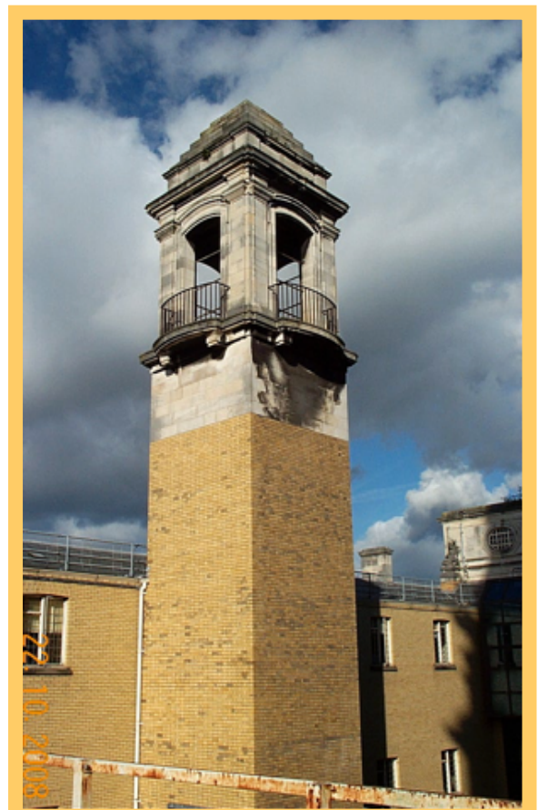
Main extract tower housing chimney and extract ducts
