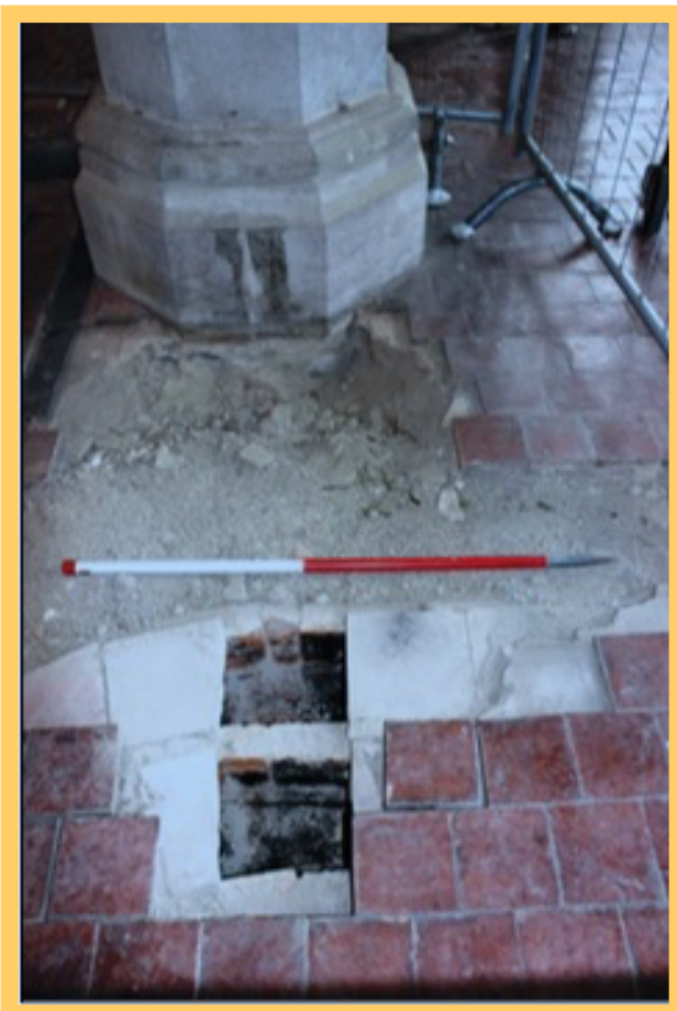
Twin floor ducts viewed from West
