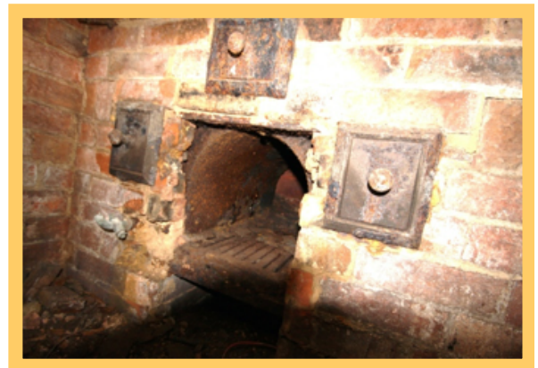
Angled view showing the 3 soot clean-out doors
