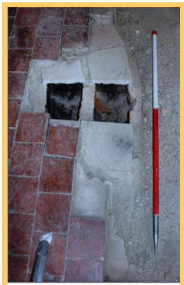
Twin floor ducts viewed from North
