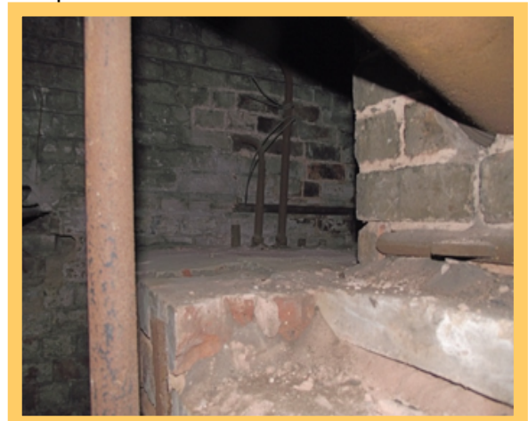
Pipe circuits on top of brickwork furnace
