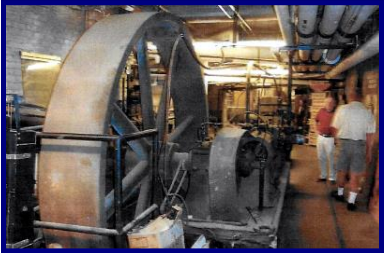
Flywheel of CO 2 refrigeration compressor.
