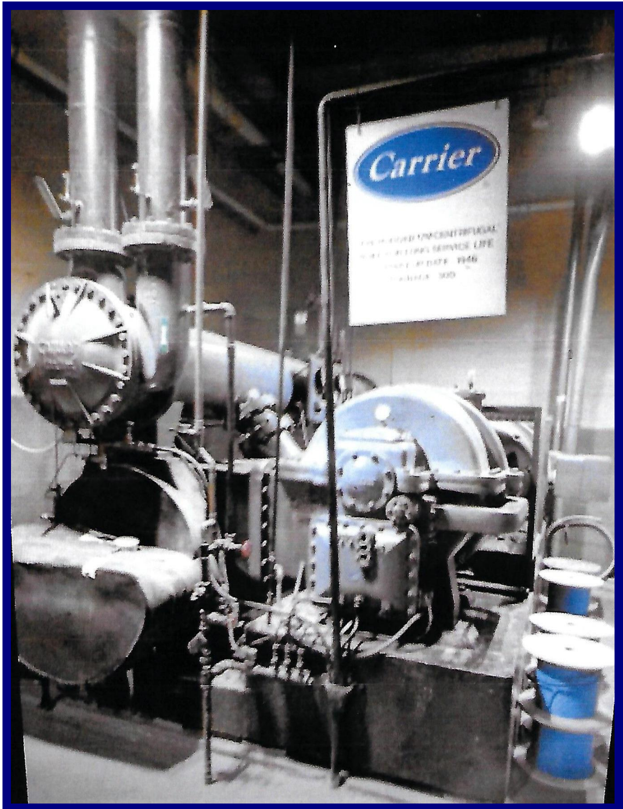
Air conditioned with NH 3 refrigeration 1926. Replaced with Carrier centrifugal 1946-64.
