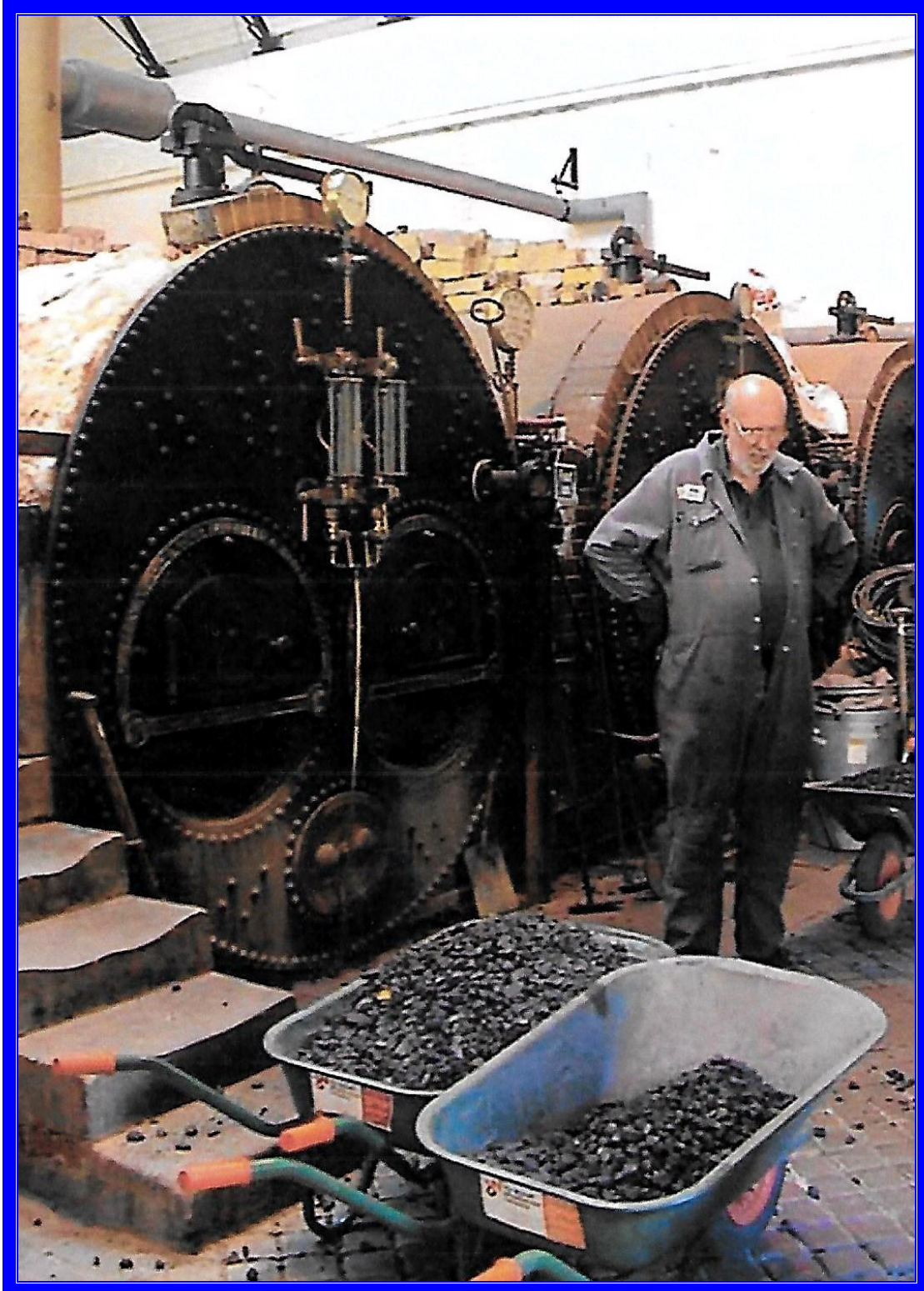
Three of the Galloway coal-fired steam boilers, original output 97 kW each, later updated.
