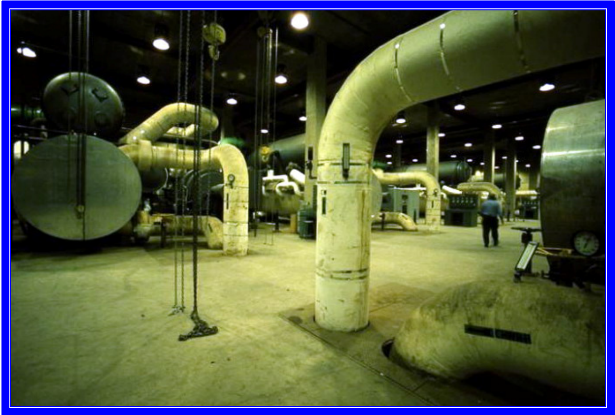
The sub-basement plant room housing the refrigeration plant
