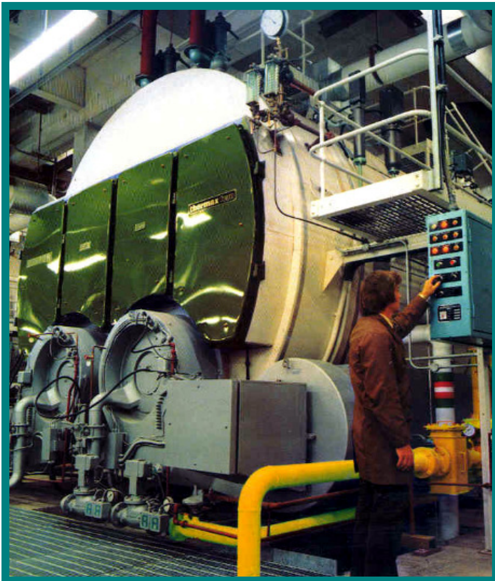
One of the gas-fired Thermax Steam Boilers in the Hartcliffe Power House
