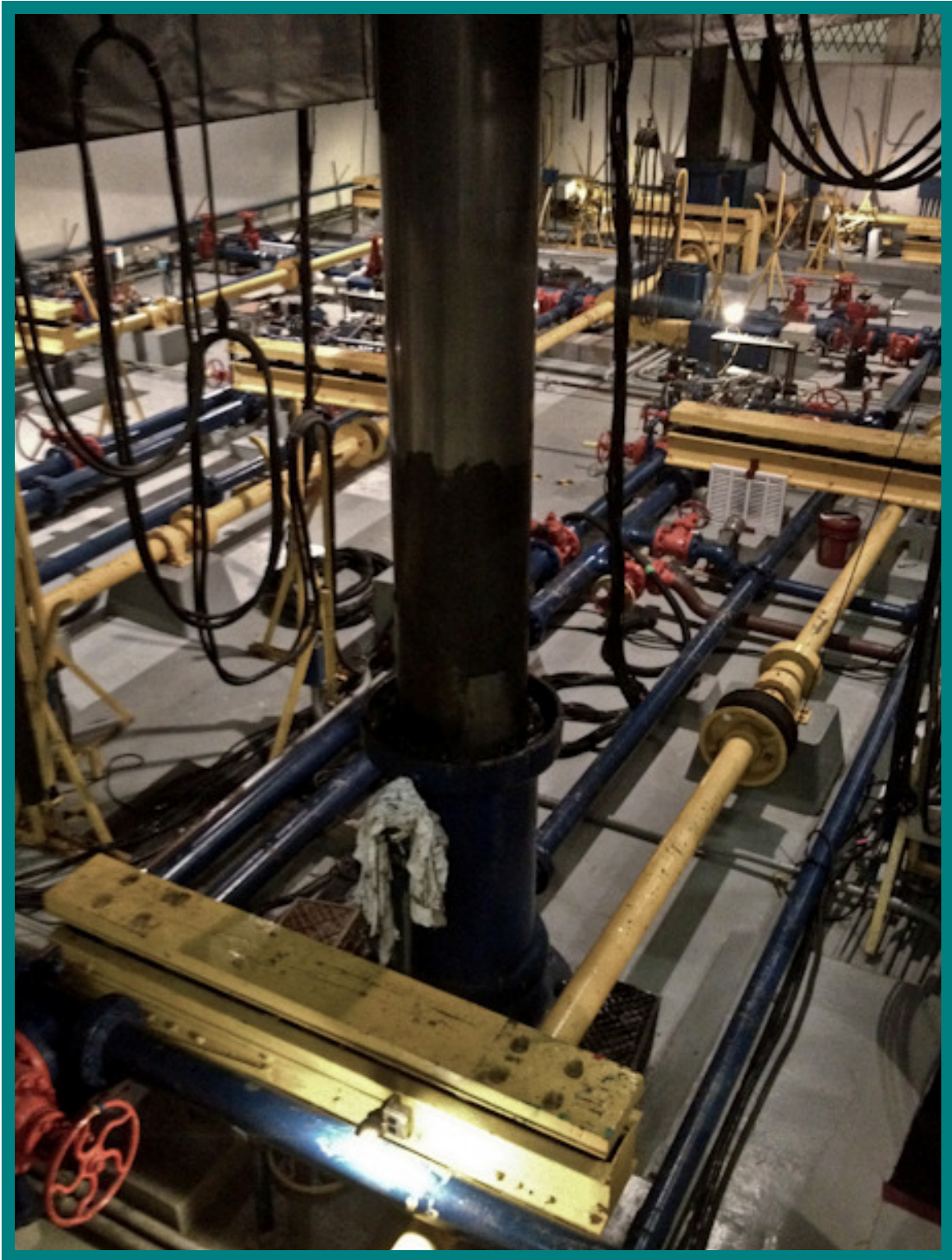
Part of the under-stage hydraulic elevator system capable of lifting a full symphony orchestra to auditorium level.
