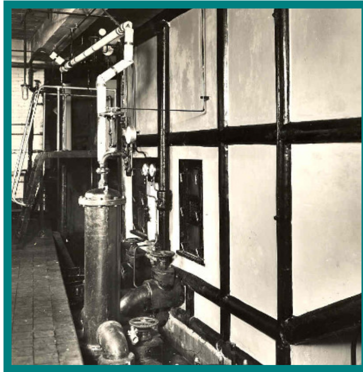
Air conditioned was installed by Carrier, the plant including this air washer
