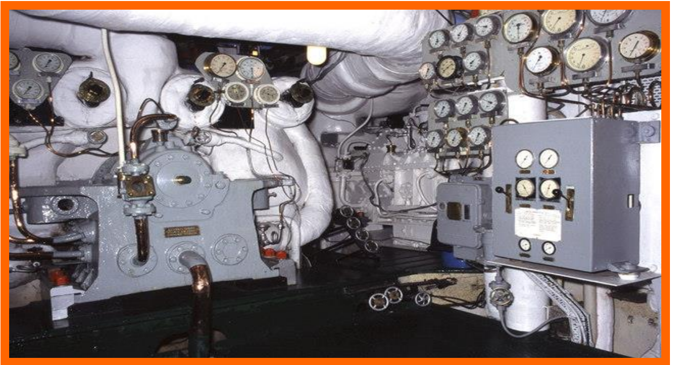
Forward engine room.
