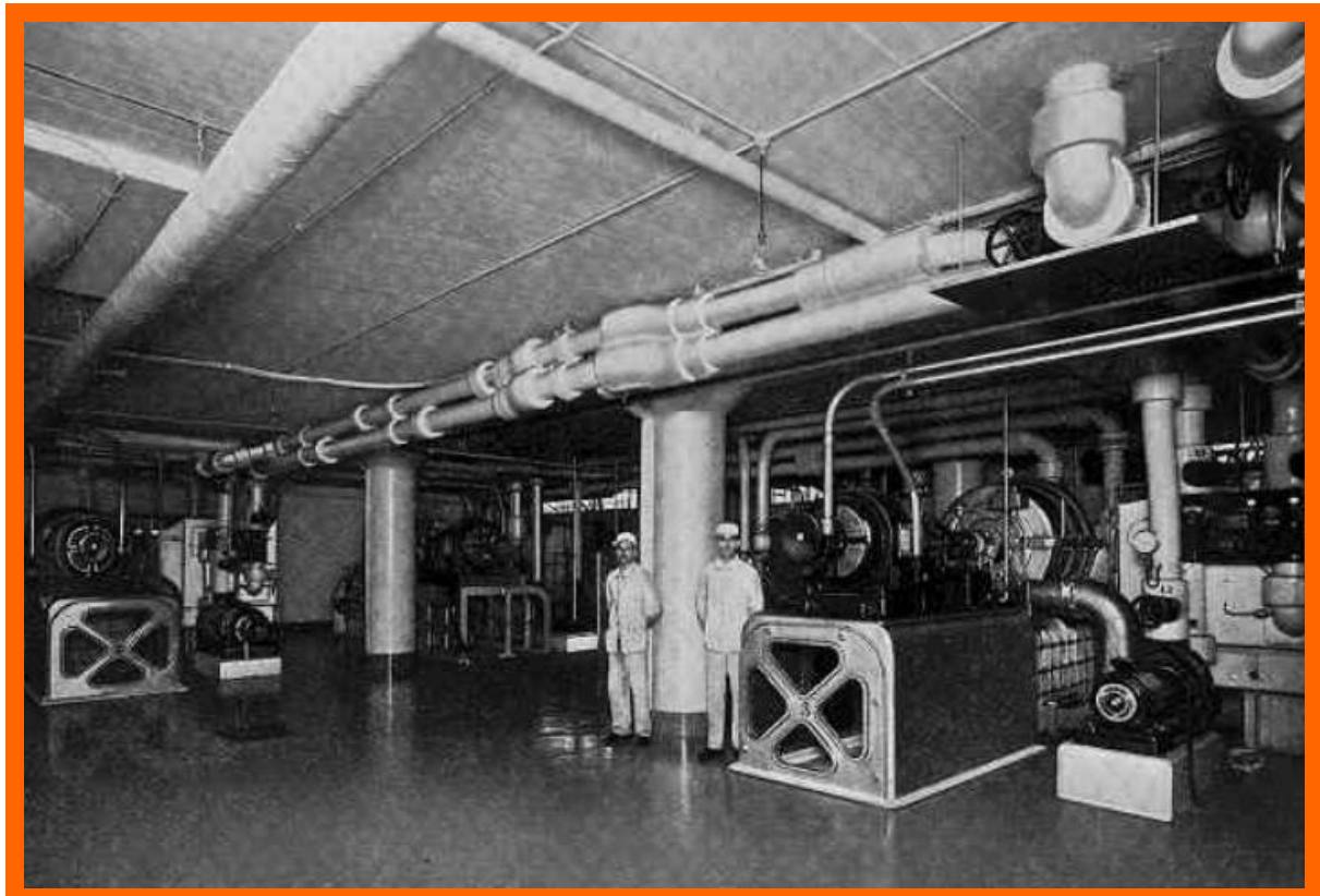
Three Carrier centrifugal water chillers (350 TR total) at Wrigleys, c.1928.
