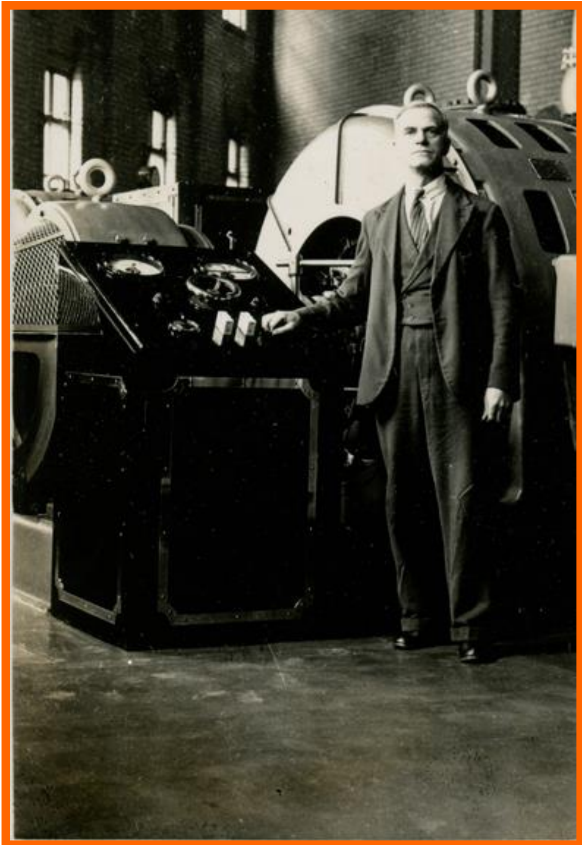
The J & E Hall refrigeration compressors. All photographs from The Grimsby Ice Factory Trust.
