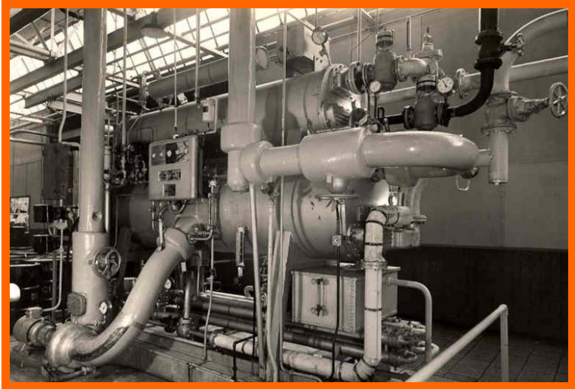
Carrier absorption water chiller (150 TR) at J. Lyons, Greenford, c.1962.
