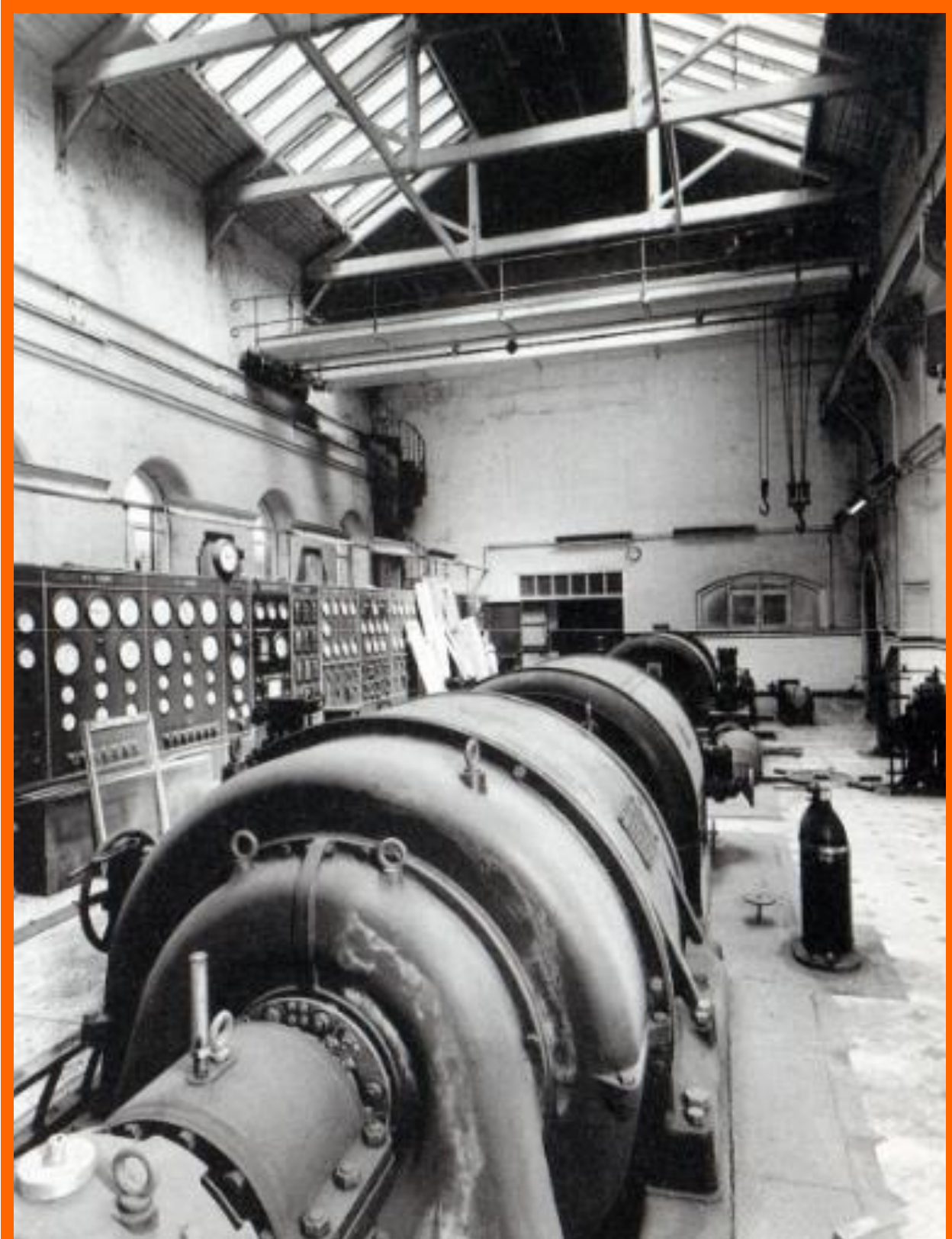
Turbine and switch room at Manningham Mills, Bradford in Yorkshire, 1930s.
