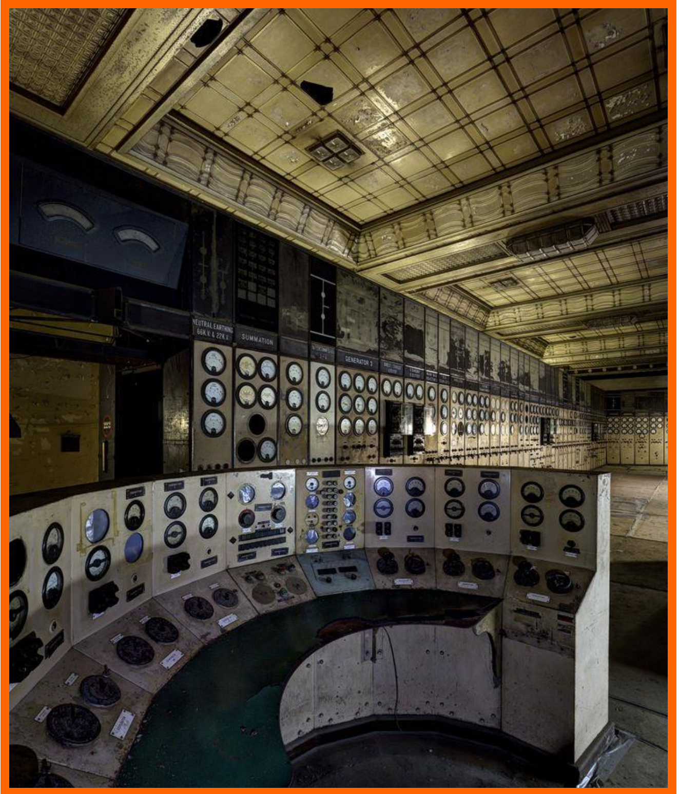
Just a part of the complex operating and monitoring control panels.
