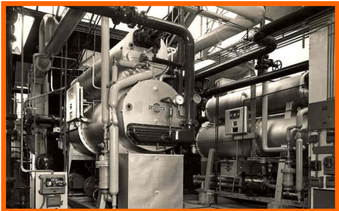
Two Carrier absorption water chillers at James Pascall, Mitcham, 1960s.
