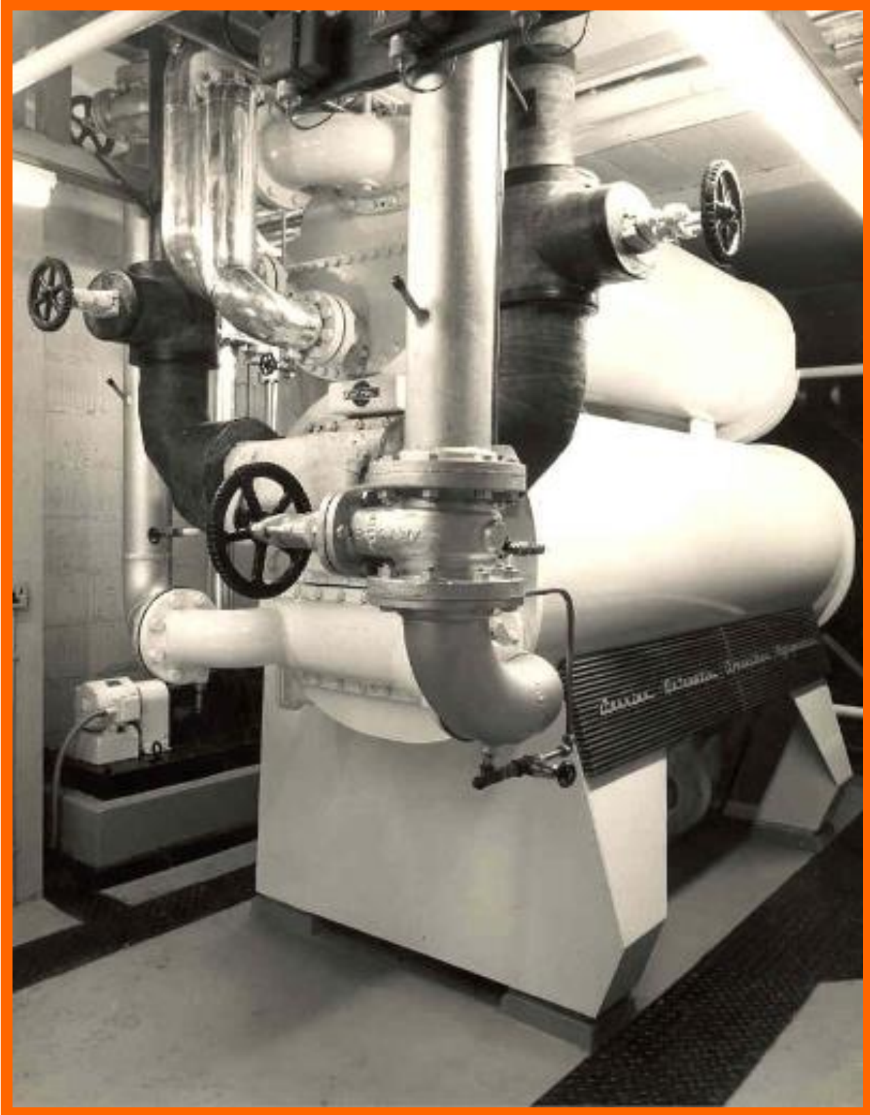
Carrier Type 16E absorption chiller in Carrier House, Victoria, London, 1963.
