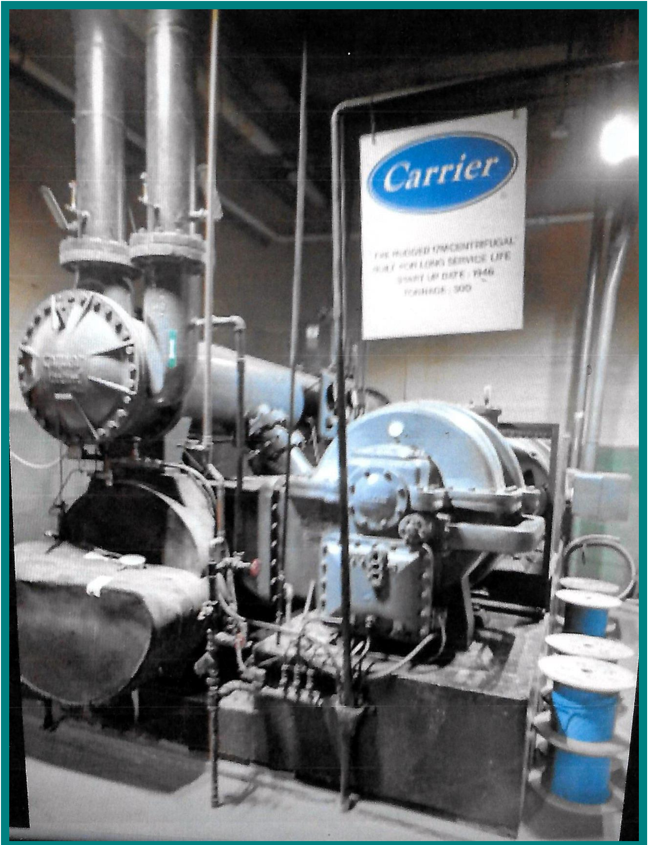
The original centrifugal chiller installed in the Fox Theatre, Atlanta in 1929. Replaced in 1960.
