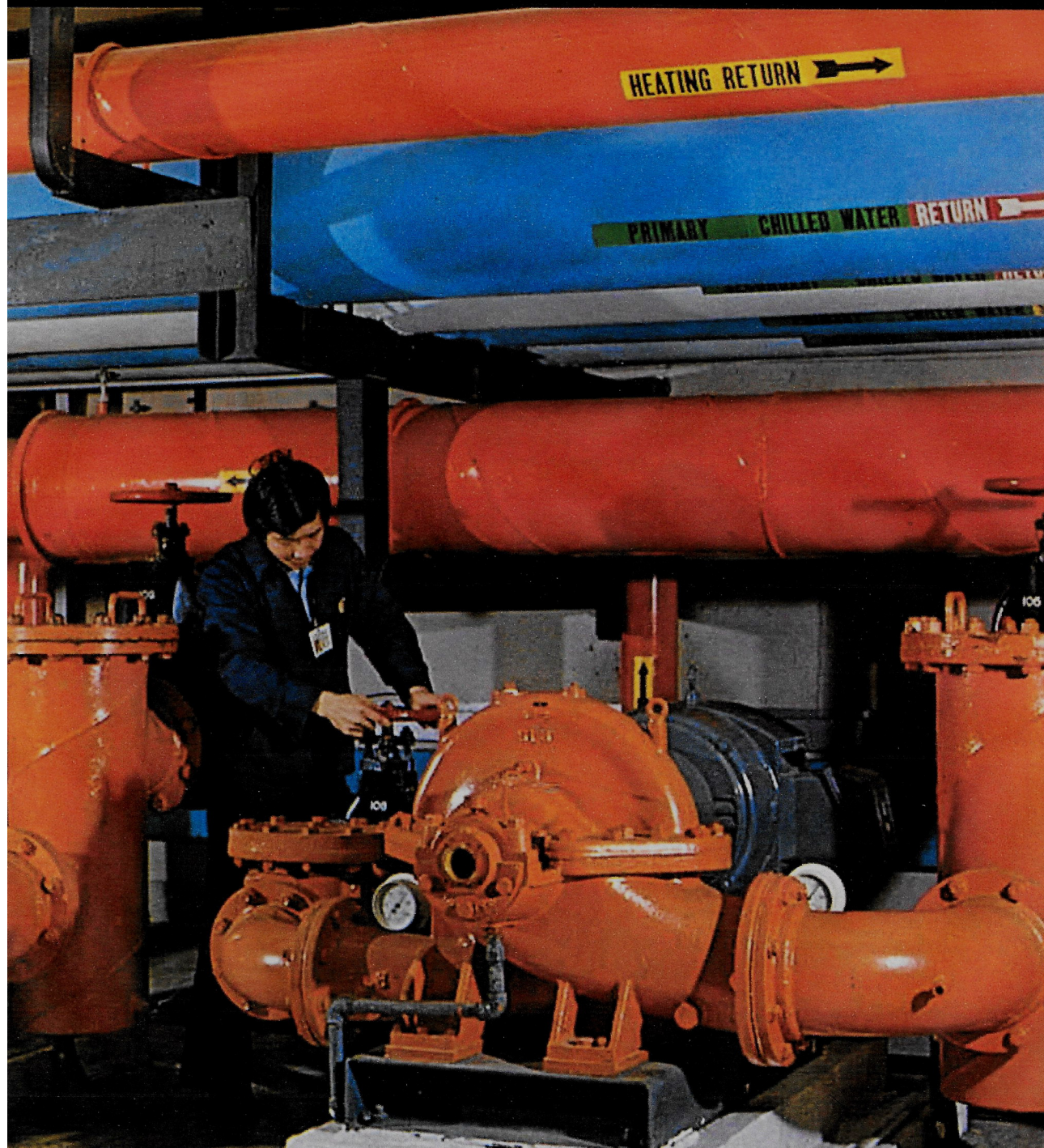
Refrigeration plan room, Cable & Wireless, Hong Kong
