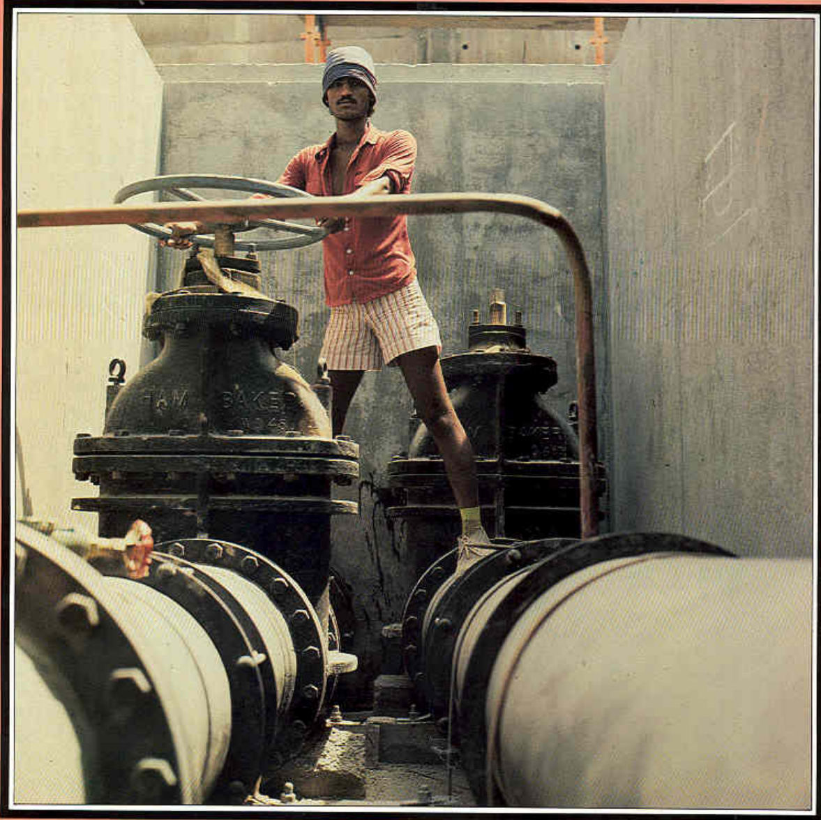
Above / Rashidiya Water Tank, Dubai, U.A.E. / Lunar Drake & Scull (U.A.E.) was responsible for all mechanical and electrical engineering services associated with the construction of this 12 million gallon water tank.
