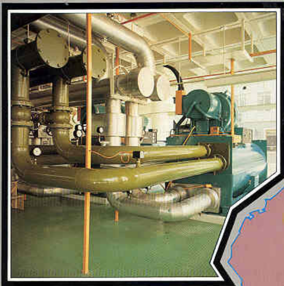
Above / Willis, Faber & Dumas Ltd., Head Office Ipswich / All the mechanical engineering services for this RIBA award winning office building accommodating some 1350 people were installed by Drake & Scull. Heavy mechanical equipment including the fridge unit above is located at ground floor level, where it forms an architectural feature visible through the glass walls.
