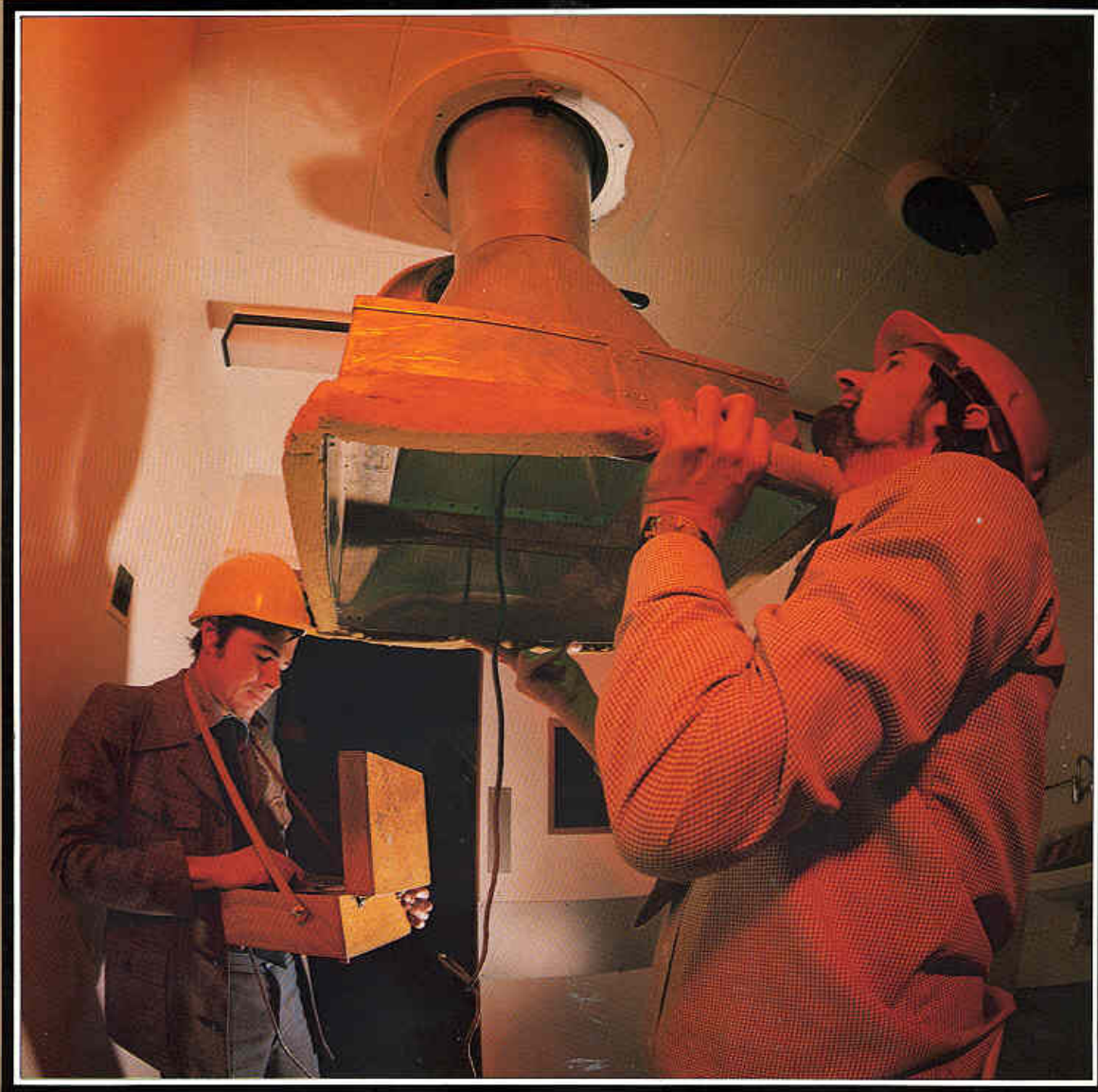
Above / King's Lynn District General Hospital / Drake and Scull was the main engineering services contractor for this new 'Best Buy' 500 bed hospital, installing the heating, ventilation and air conditioning, hot and cold water services, sanitation, medical gas supplies, fire protection, electrical power and lighting, street lighting, alarms and control systems.
