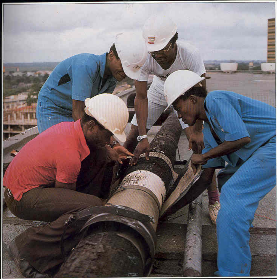
Above / Secretariat and Museum Complex, Port Harcourt, Nigeria / Drake & Scull (Nigeria) Ltd. was responsible for all electrical, mechanical, air conditioning, and plumbing services to this new complex.
