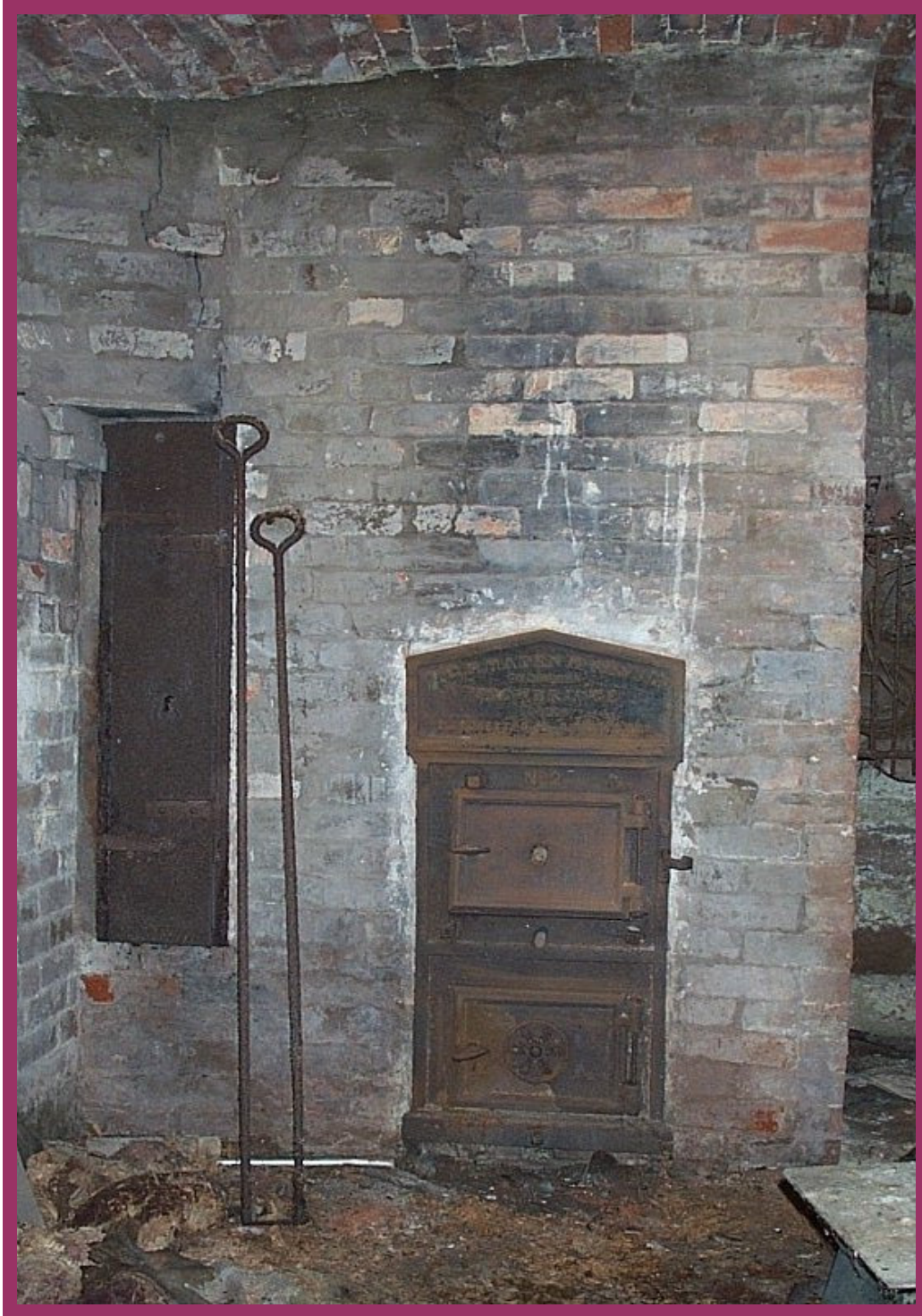
1860 G N Haden stove, Size 2, Serial 1907 Holy Trinity Church, Ventnor, IoW Architect C E Giles of Taunton
