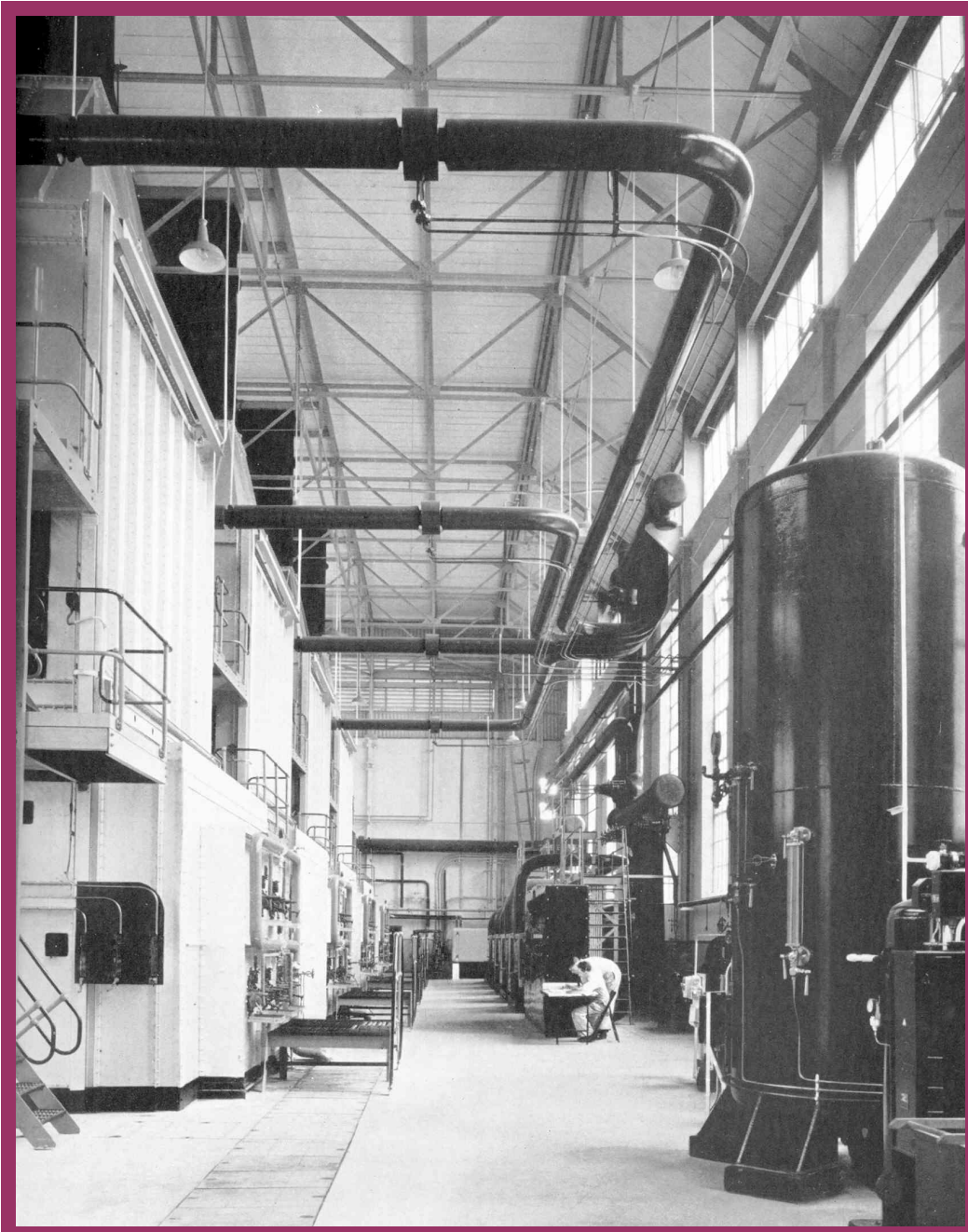
Leyland Motors Ltd, Ministry of Supply Factory, Lancashire Heating by HPHW working at 225 psig provided by four boilers with a total capacity of 184 million Btu/h and with waste heat reclaim from diesel generators and the rubbish incinerator [Architect Harry S Fairhurst & Sons]
