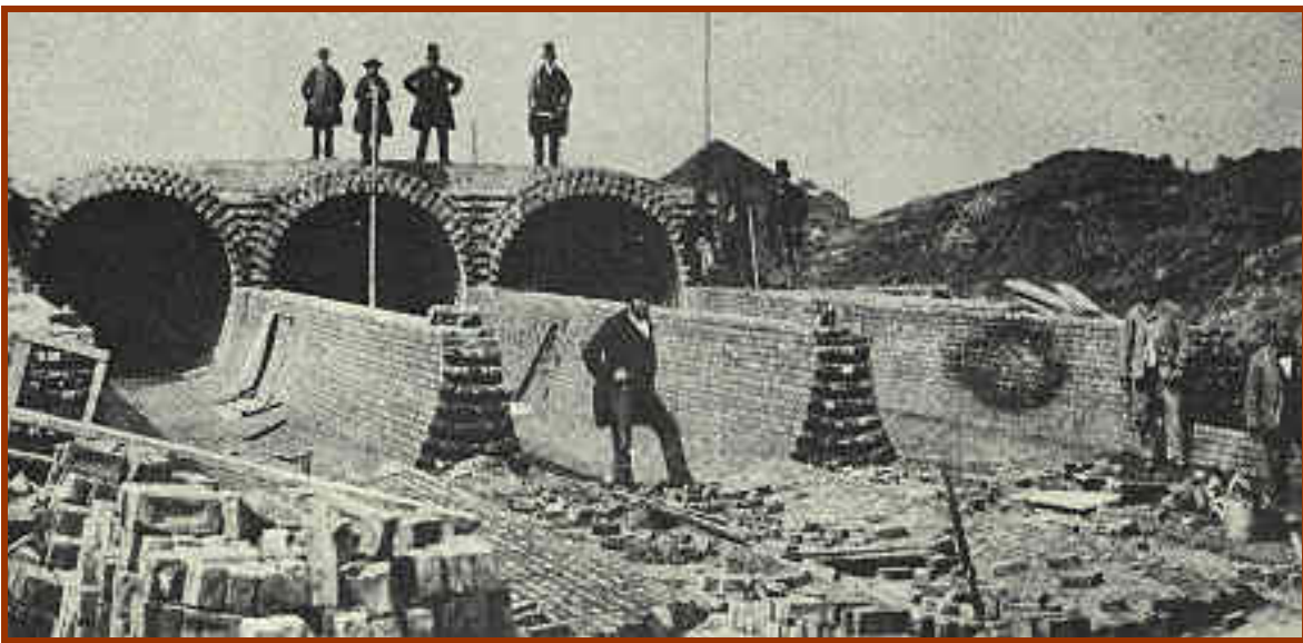
Construction of the Crossness sewage treatment works at Crossness, at the confluence of the Thames and Barking Creek (London page 73)
