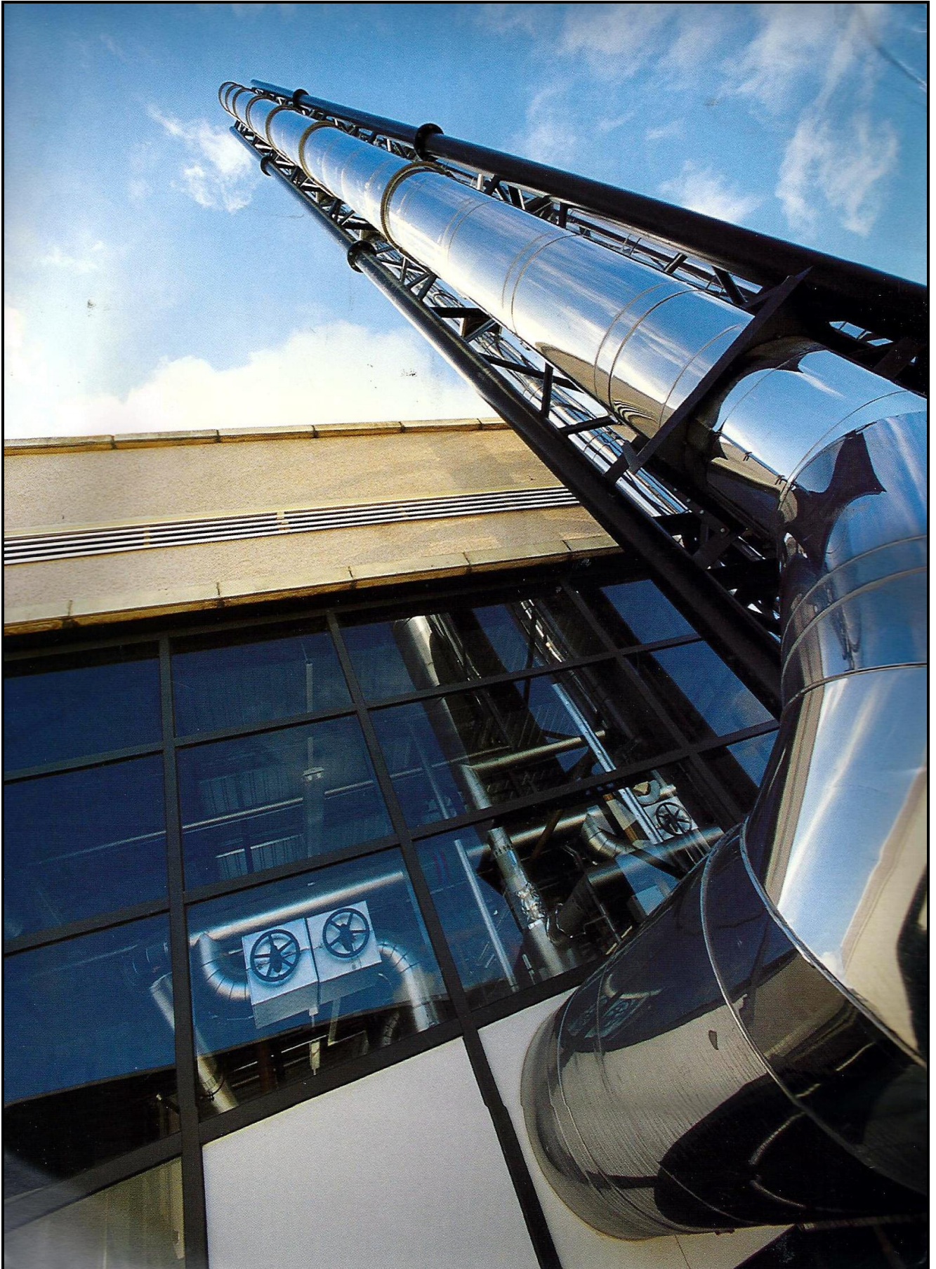
Boiler House & Chimney (Richard Irwin Building Services) (The original Company dates back to 1871)
