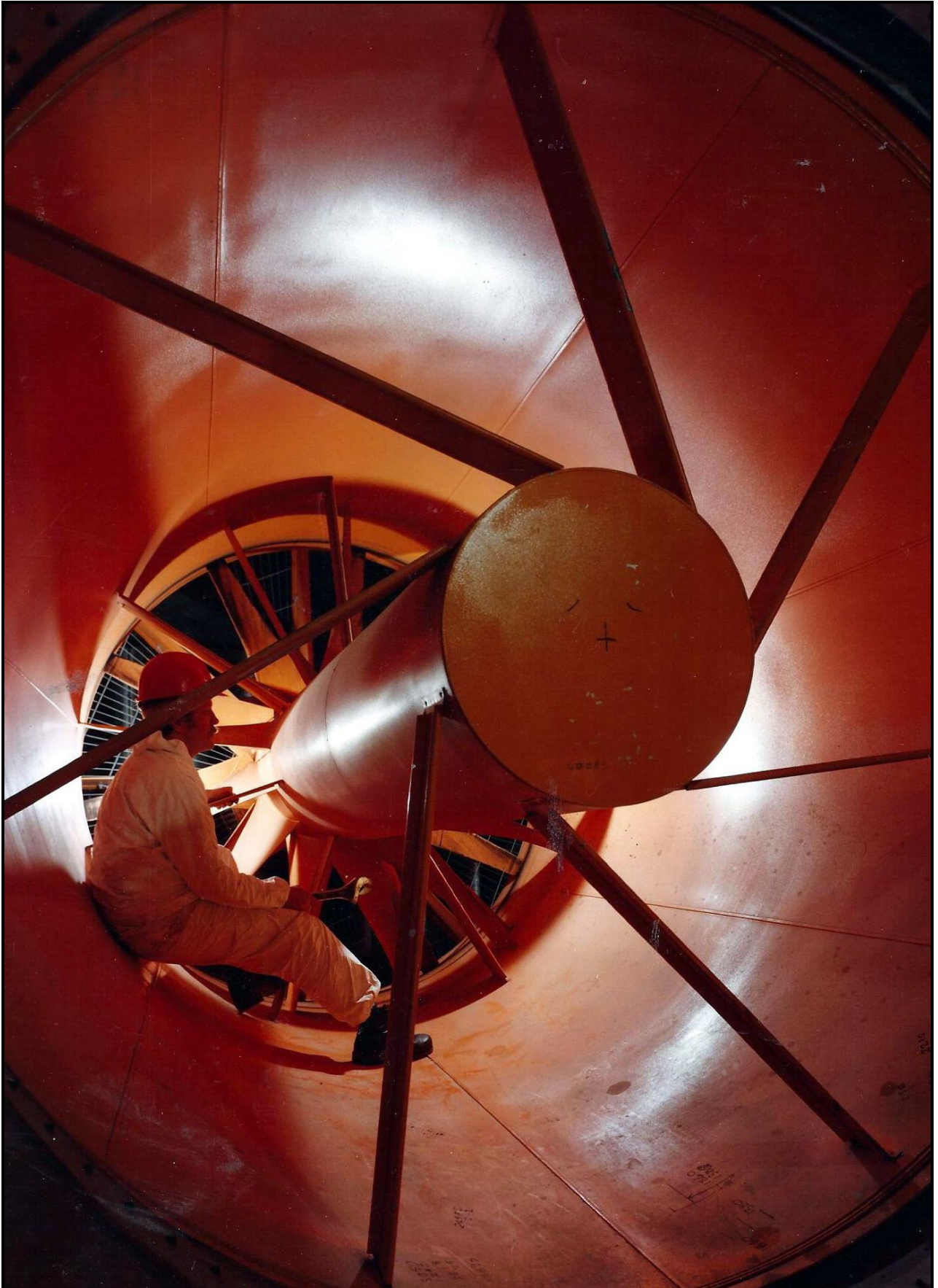
Commissioning the main supply air fan at Glasgow Royal Infirmary DSSR was established in Glasgow in 1945
