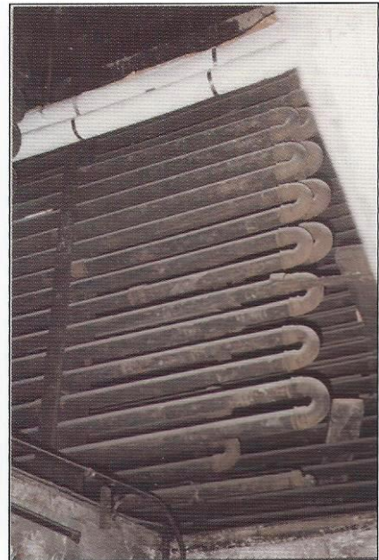
Existing heating coils
