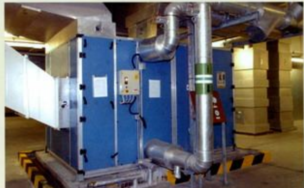
Air-conditioning plant at Tiu Keng Leng Station completed in 2002
