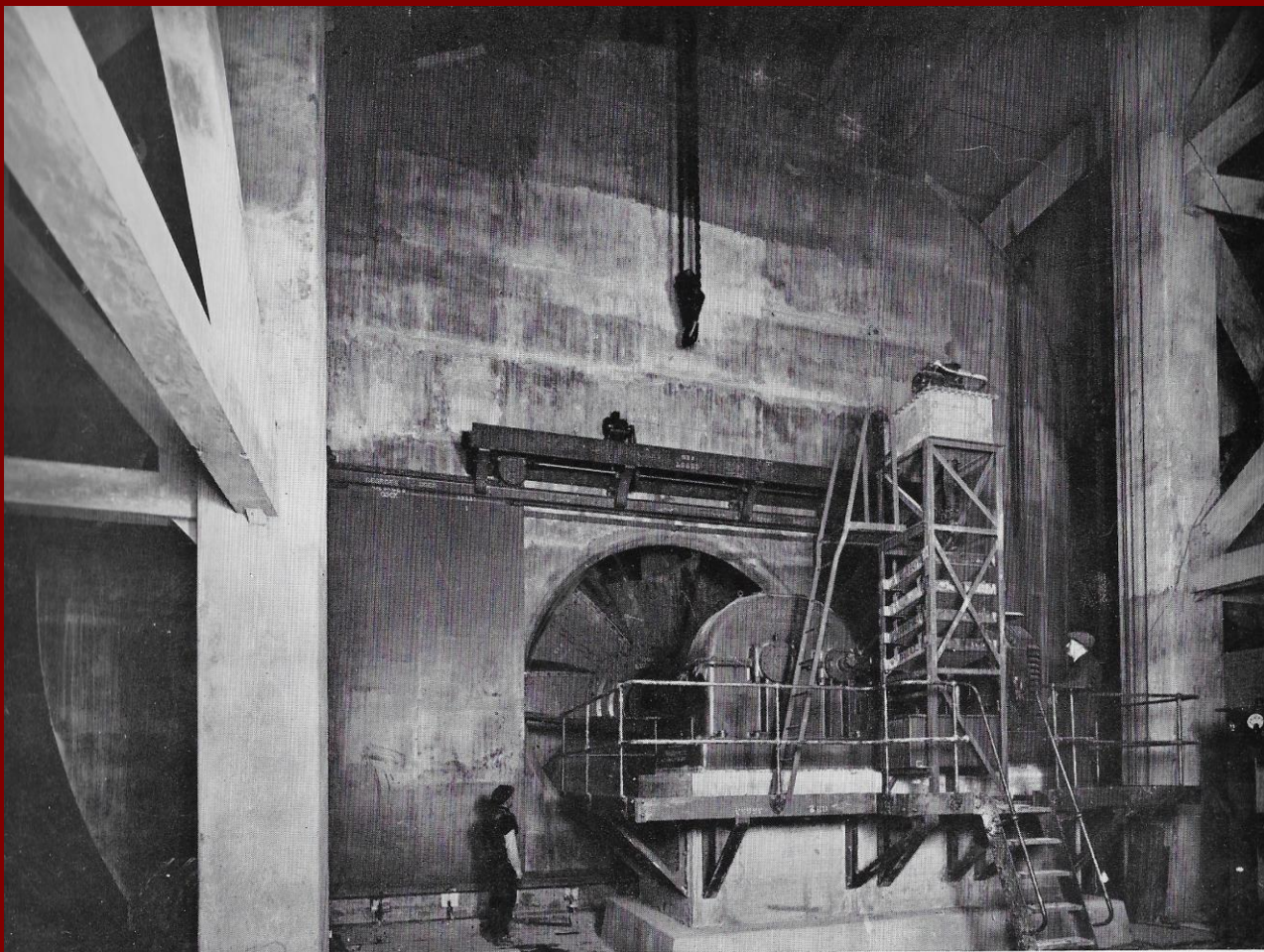
Blowing fan and casing at George's Dock ventilation station, Liverpool
