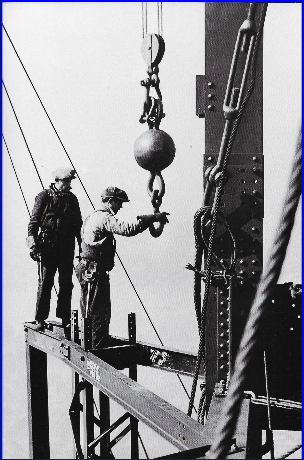
Photograph by Lewis W. Hine of Empire State Building steelwork mooring mast
