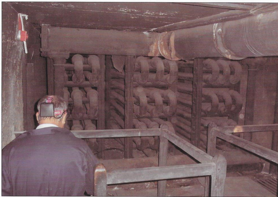
Heating chamber and coils as existing today
