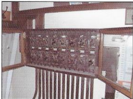
Electrical distribution board
