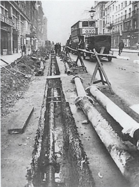
Replacing LHP Co. hydraulic mains in Piccadilly around 1930. The original cast-iron pipes with oval flange spigot and faucet joints are being removed and replaced with new steel pipes using Victaulic joints. Mercury Communications press photo.
