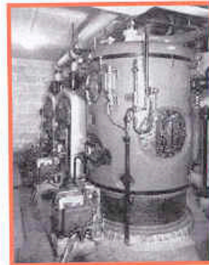
1939 Finsbury Health Centre, London (Oil-fired boilers by G N Haden & Sons)
